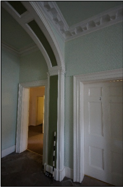
Plate 9: The depressed arch and cornice of Hallway 08 and architrave and door leading into Room 04, viewed looking north-east.
