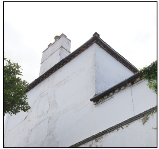
Plate 5: The dentil cornice extending across the east gable and elevation, viewed looking west.
