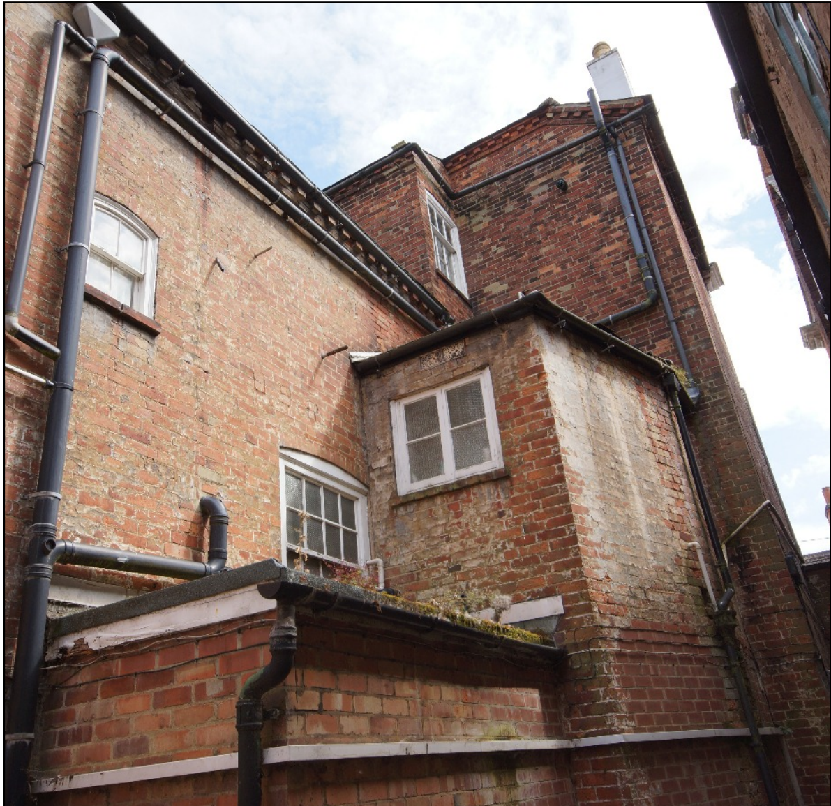
Plate 6: The west gable and elevation and later two storey extension, viewed looking south-east. Note the dentil cornice extending around both the gable and elevation and the three sash windows which are the only surviving original windows in the building.
