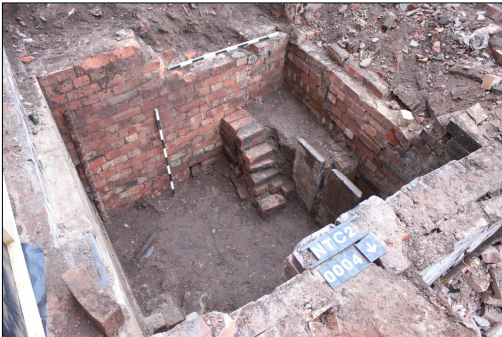
Plate 40: View of southern wall [0006] (on left) and western wall [0007] (on right) of 'cellar' [0004]. Fill partly excavated, showing brick pile placed in the corner.
