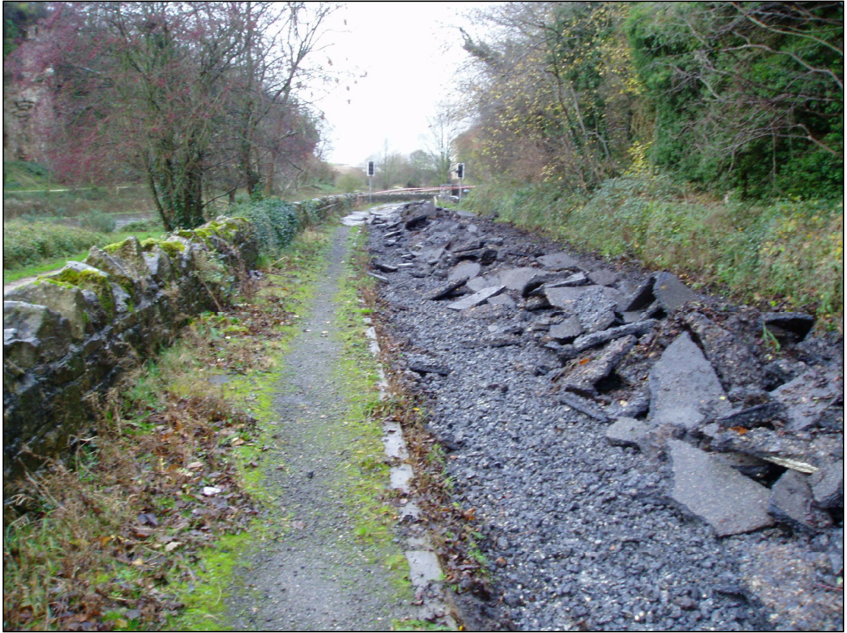
Plate 13 Old Road during early stages of breaking up the tarmac. Looking west
