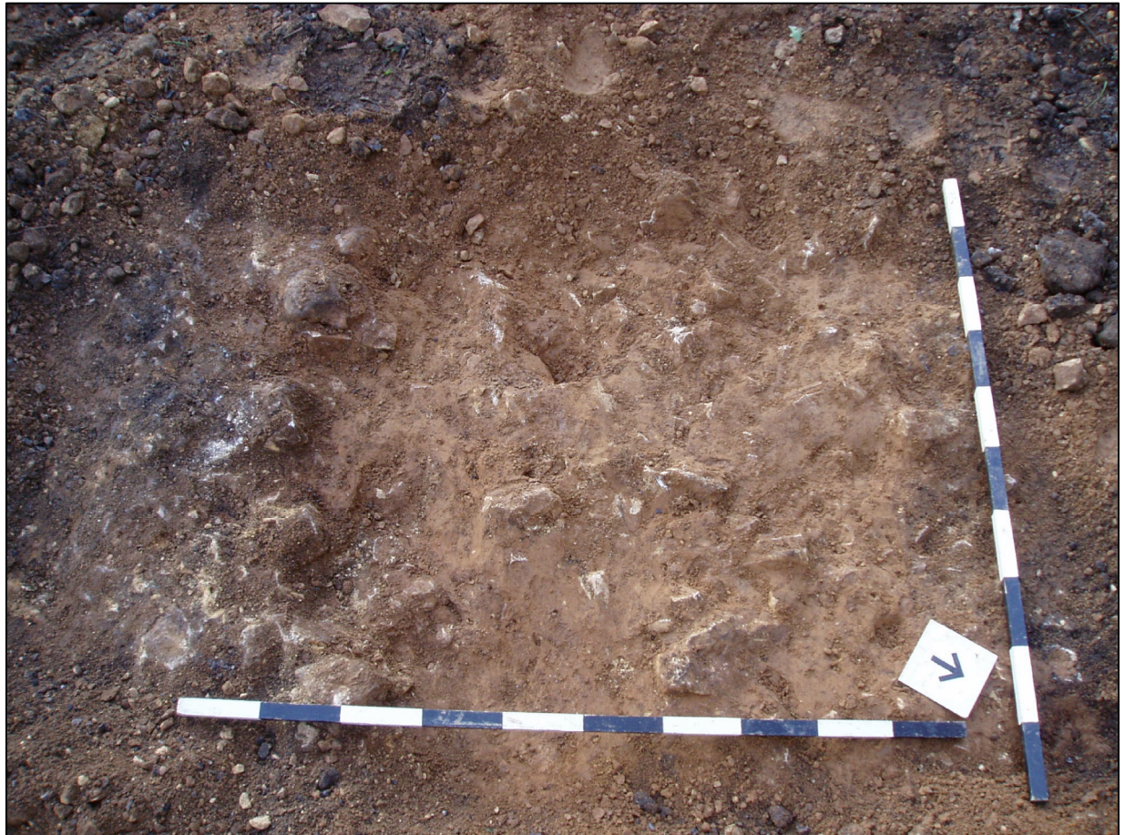
Plate 14 Area 210 at the western end of the gorge. Here the tarmac and sub-base was thin and overlay a silty sand clast supported matrix with frequent limestone inclusions
