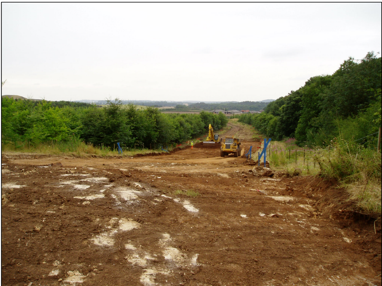
Plate 6 New Road line during topsoil stripping. Taken from the western rise looking east
