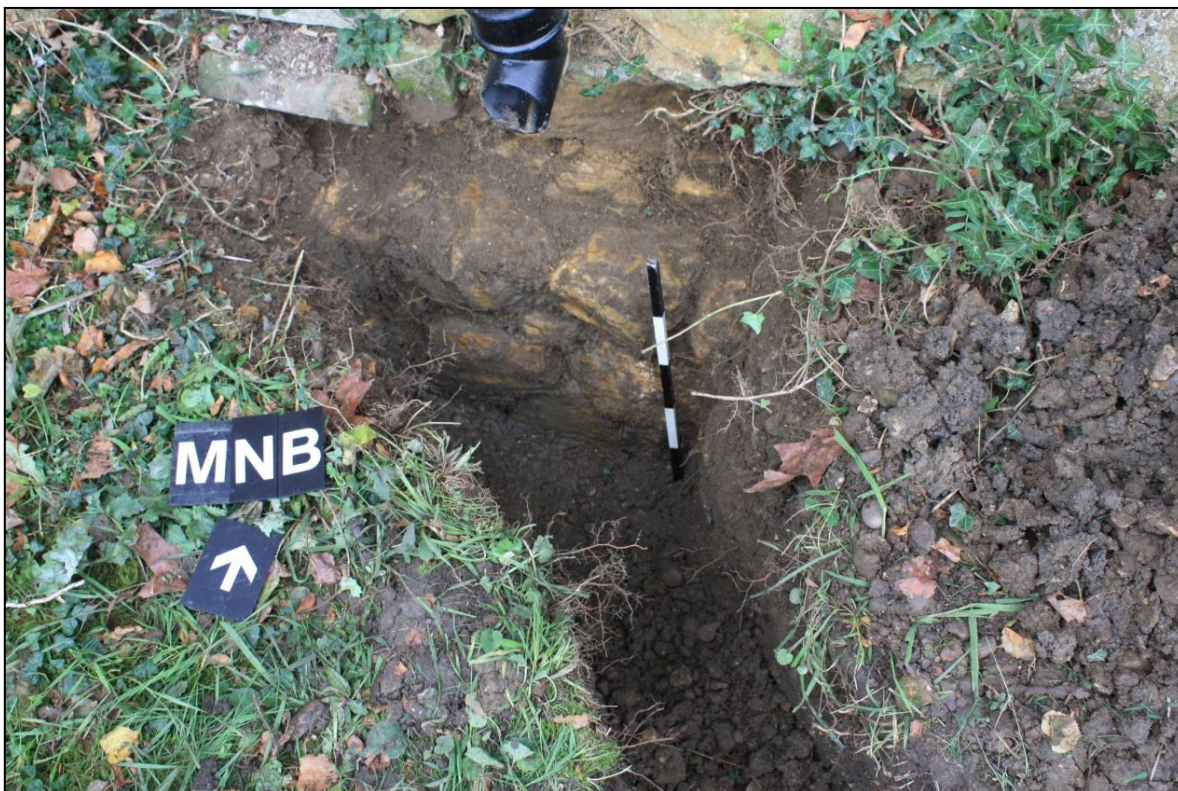
Plate17: Area 04. Original foundations for the South wall of the chancel. Looking North.
