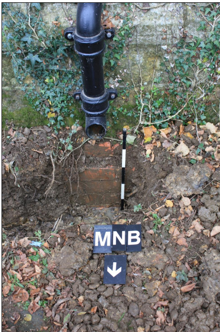
Plate 18: Area 06. Brick underpinning of the foundation of the North wall. Looking South.
