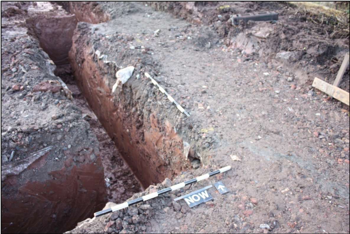
Plate 3: Machine excavation of foundation trenches, looking north east. Scale 1m x 1m.
