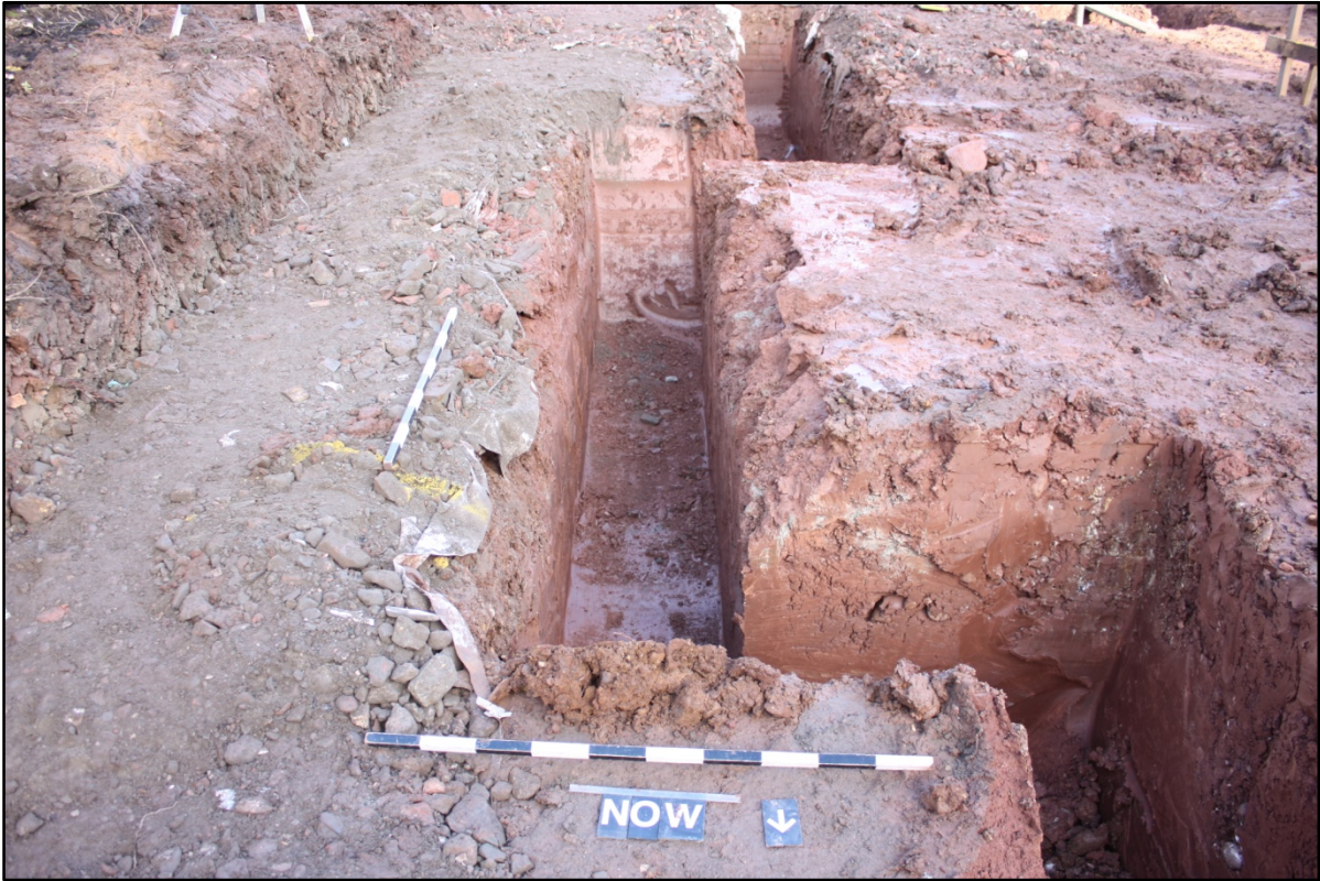
Plate 4: Overview of the northwestern extent of the site; machine excavation of foundation trenches. Looking south. Scale 1m x 1m.
