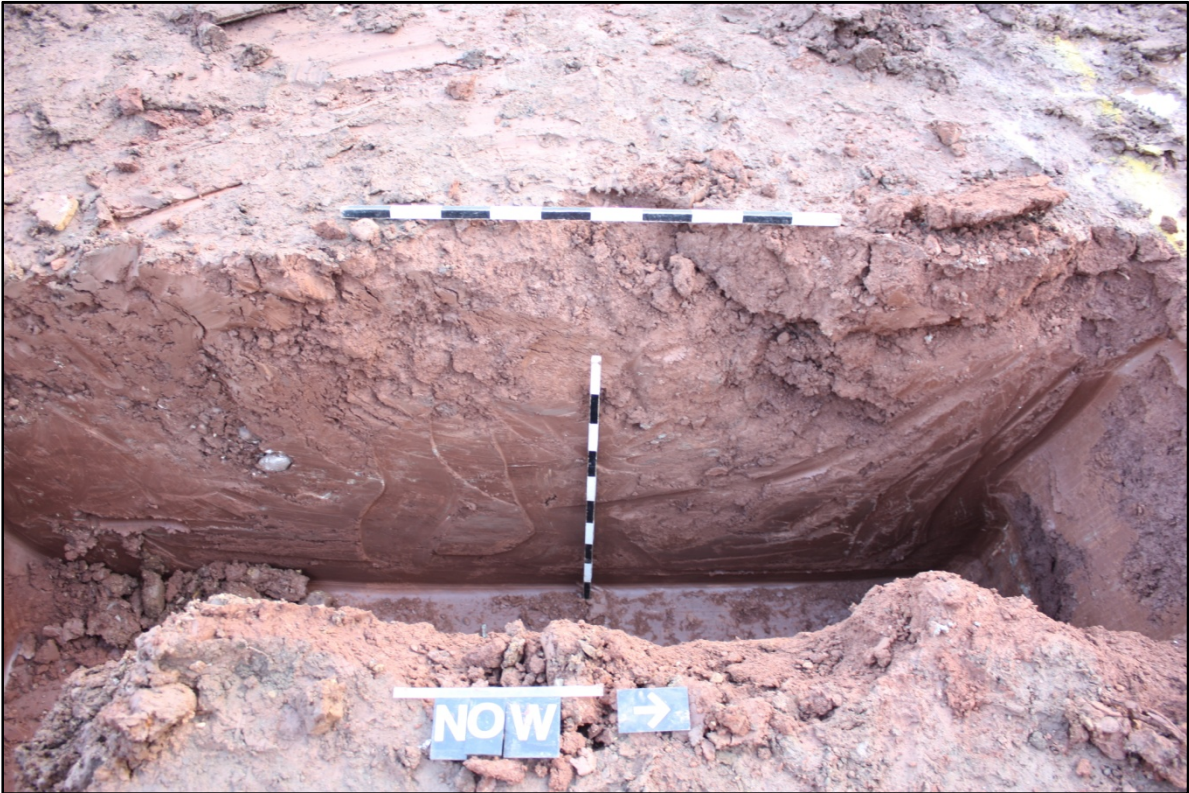
Plate 6: East facing section of the machine excavated trench for building foundations. Looking west. Scale 1m x 1m.
