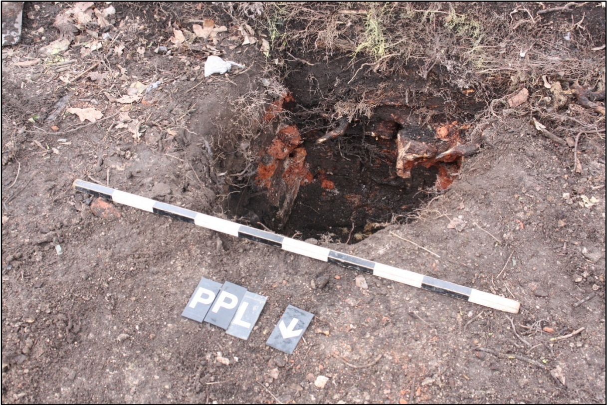
Plate 5: P2: Oblique post-excitation photo. Partial demolition of c.19th wall foundations for excavation of pillar hole, looking south-east. Scale 1m
