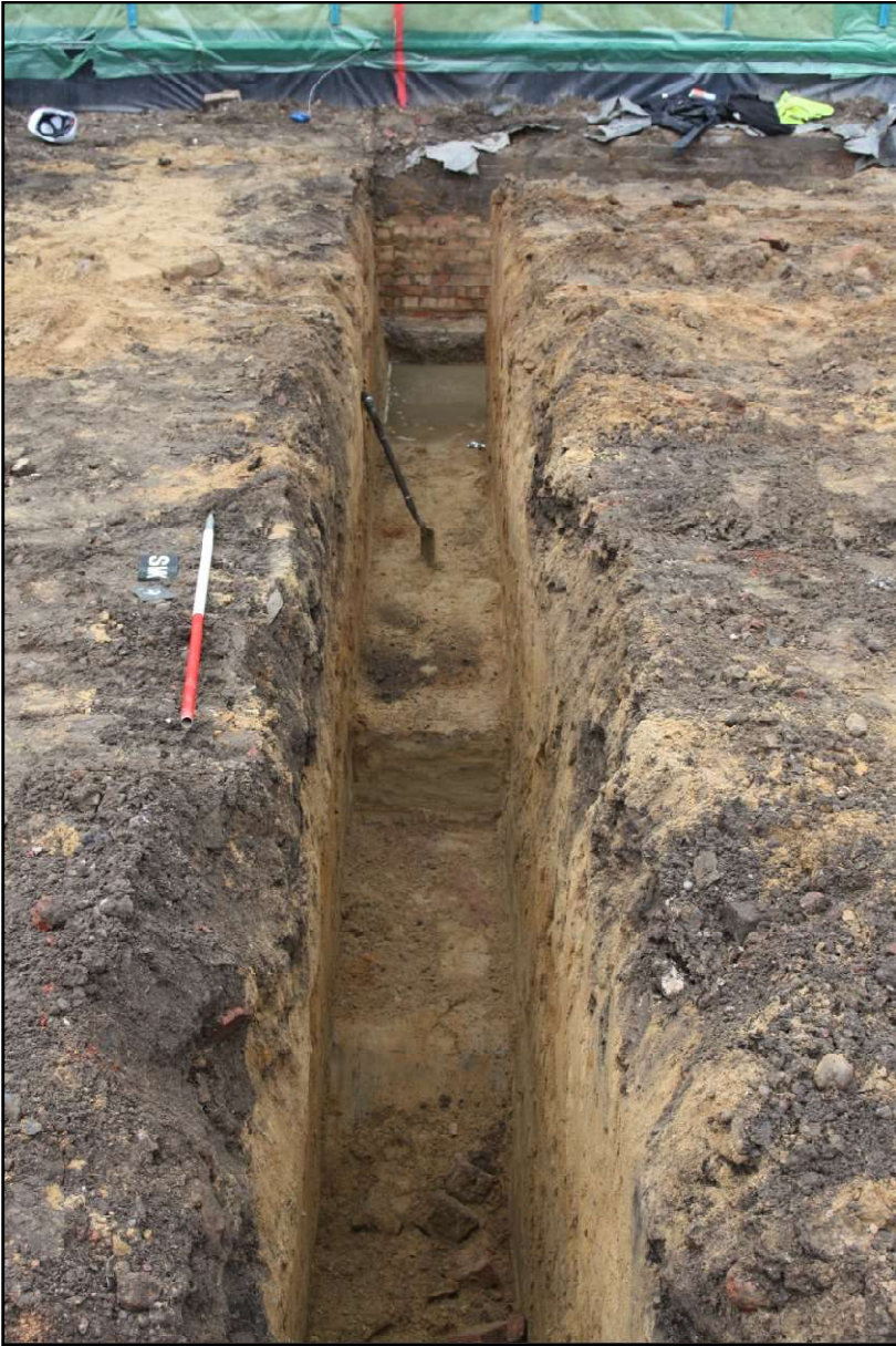
Plate 12: Excavation of the building foundations showing wall [0315] to the southeastern limit of the site. Looking south-east. Scale 1m.
