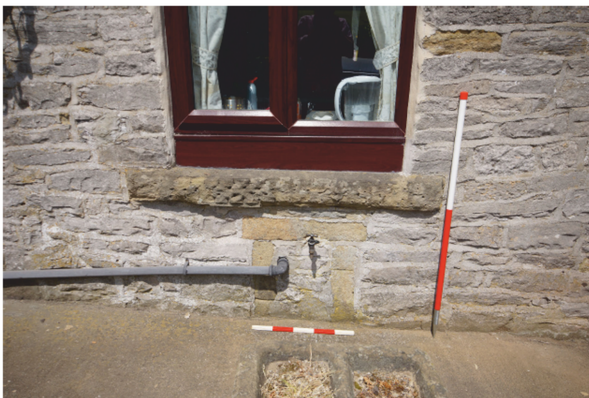
Plate 36 - Blocked opening below ground floor window on south elevation of farmhouse
