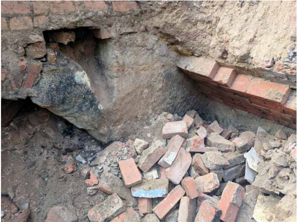
Plate 25: Detail of the sandstone skewback and brick arch in Cell 2, as well as the partially exposed rock cut wall with another barrel arch springing from it, facing south-west.
