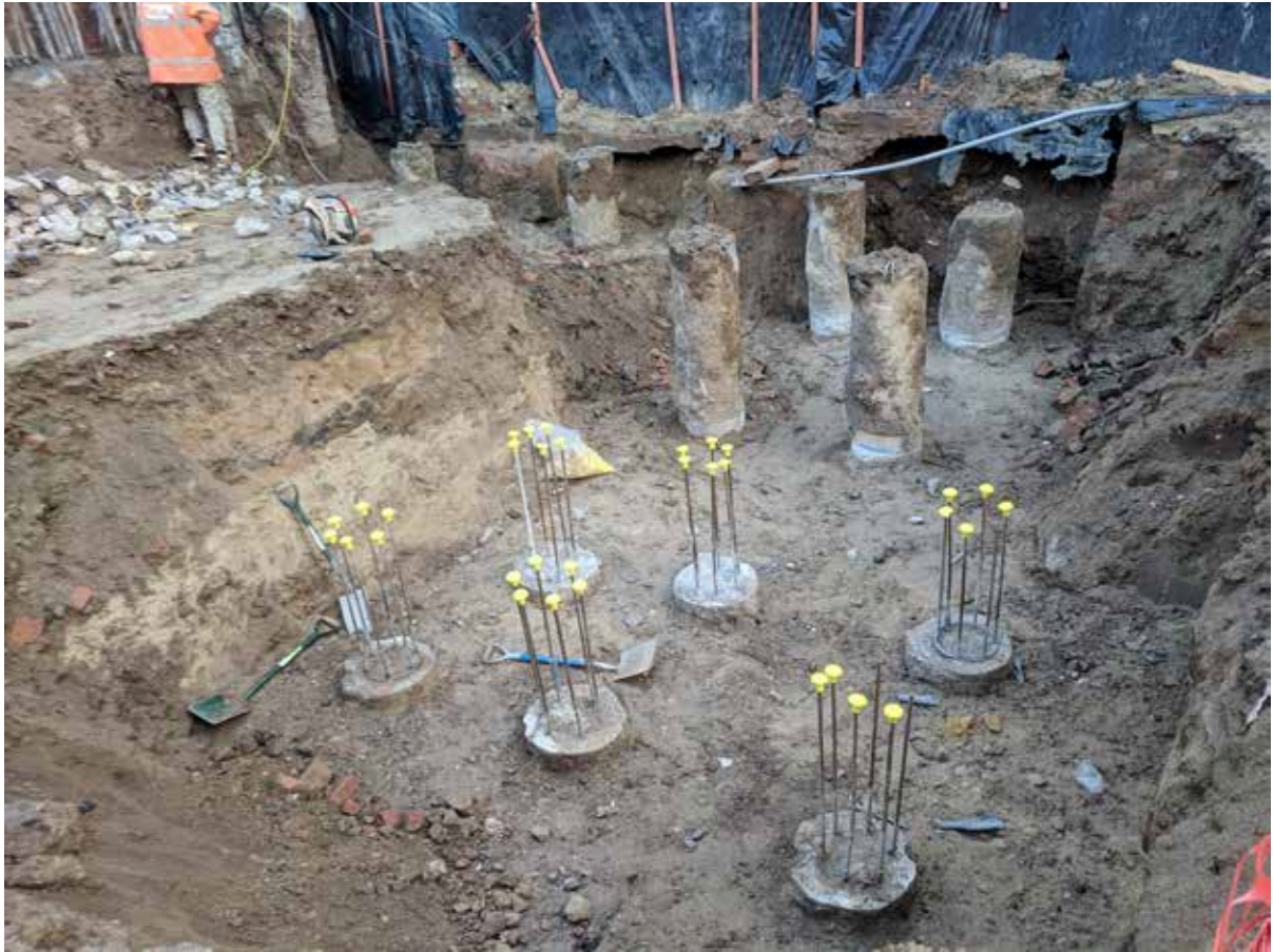
Plate 29: Site visit, facing north-east. The sandstone can be seen in the foreground. In the background, behind the unreduced piles, the partially exposed remains of a brick arch can be seen.
