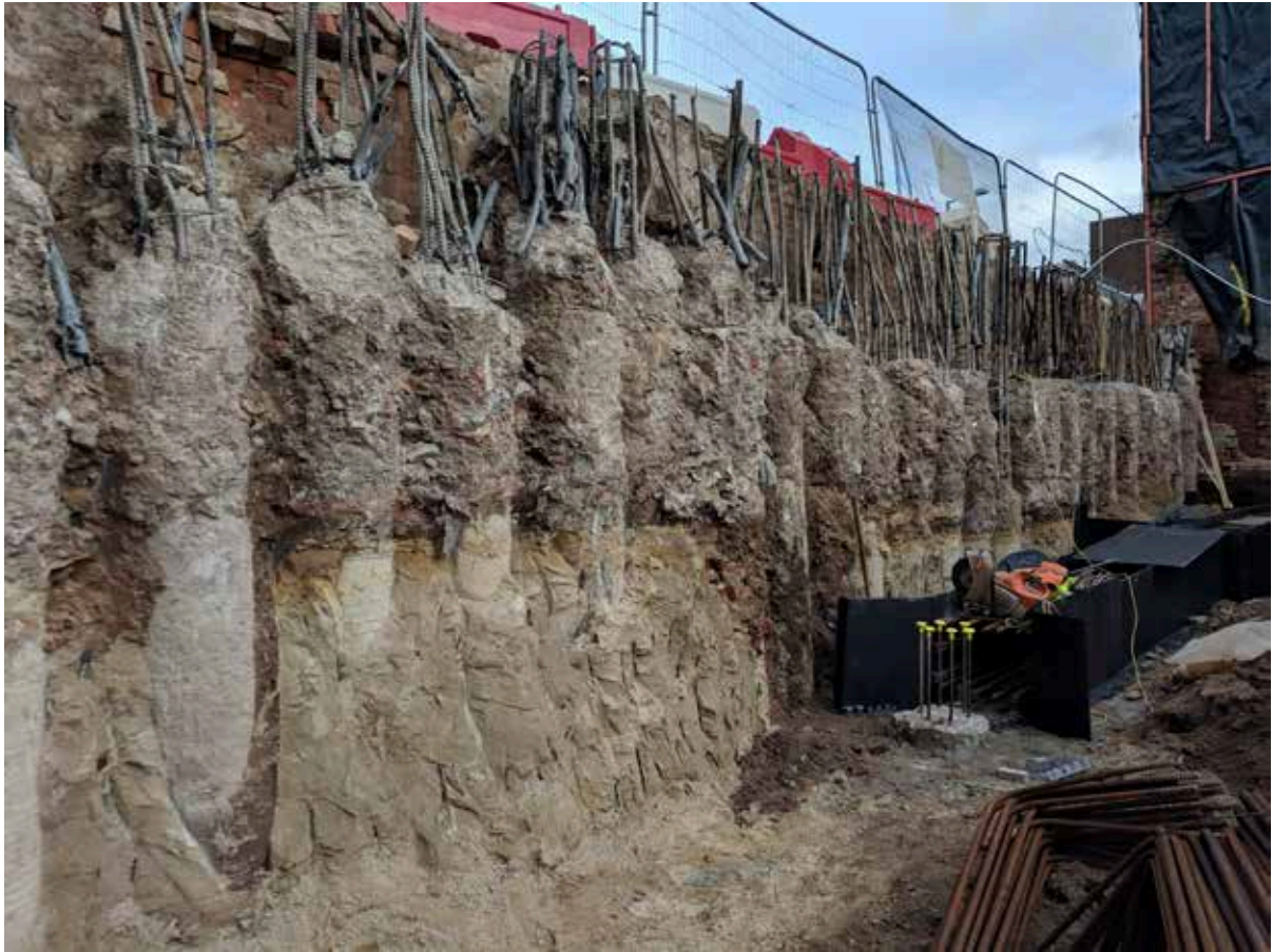
Plate 33: Site visit, facing north-east. Historical piling can be seen supporting a retaining wall to the south of Wollaton Street. In the foreground, remnants of the sandstone bedrock are visible.
