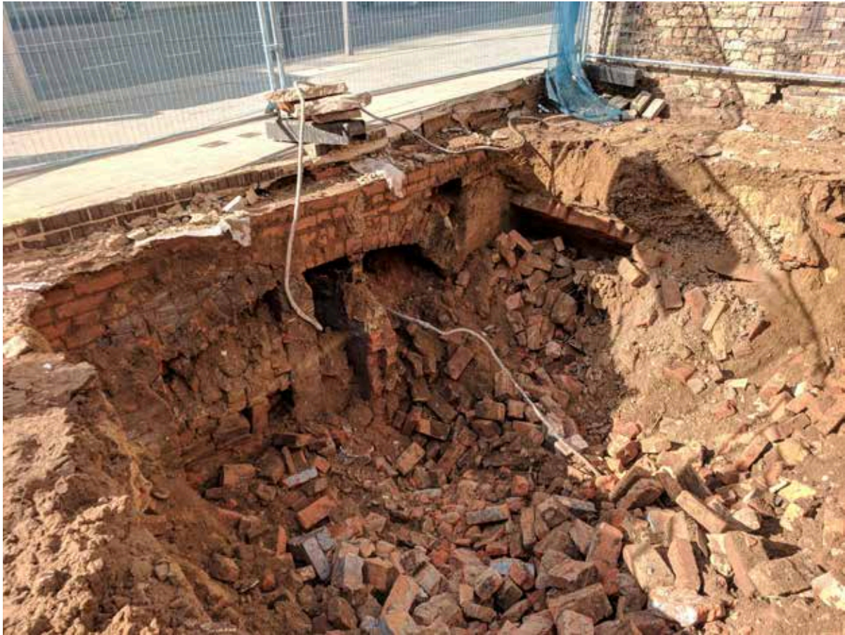
Plate 22: Cell 1 following the breach of the dividing wall into Cell 2, revealing an earlier brick arch, facing south-west. Derby Road is in the background.
