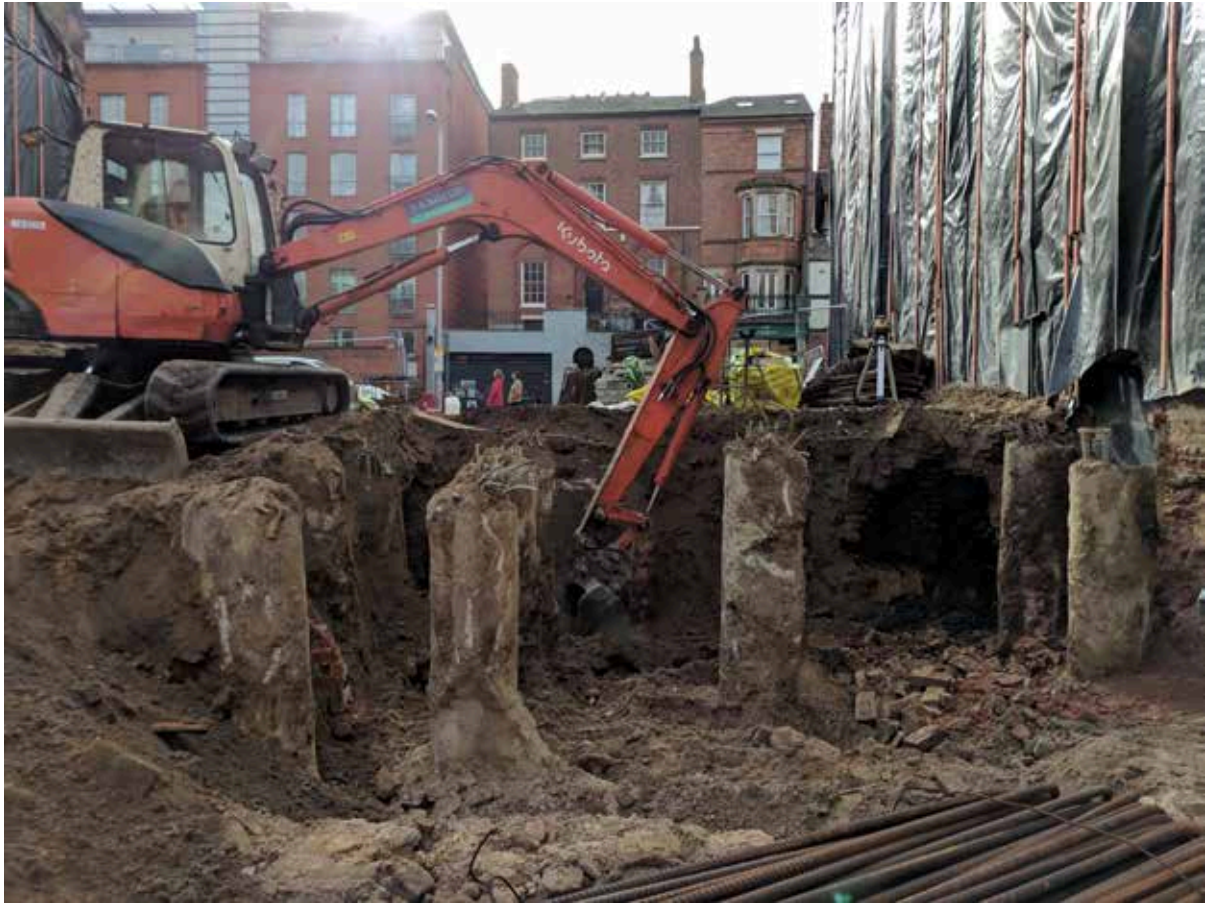
Plate 32: Site visit, facing north towards Derby Road. A partially exposed brick wall can be seen to the west (right) of the machine.
