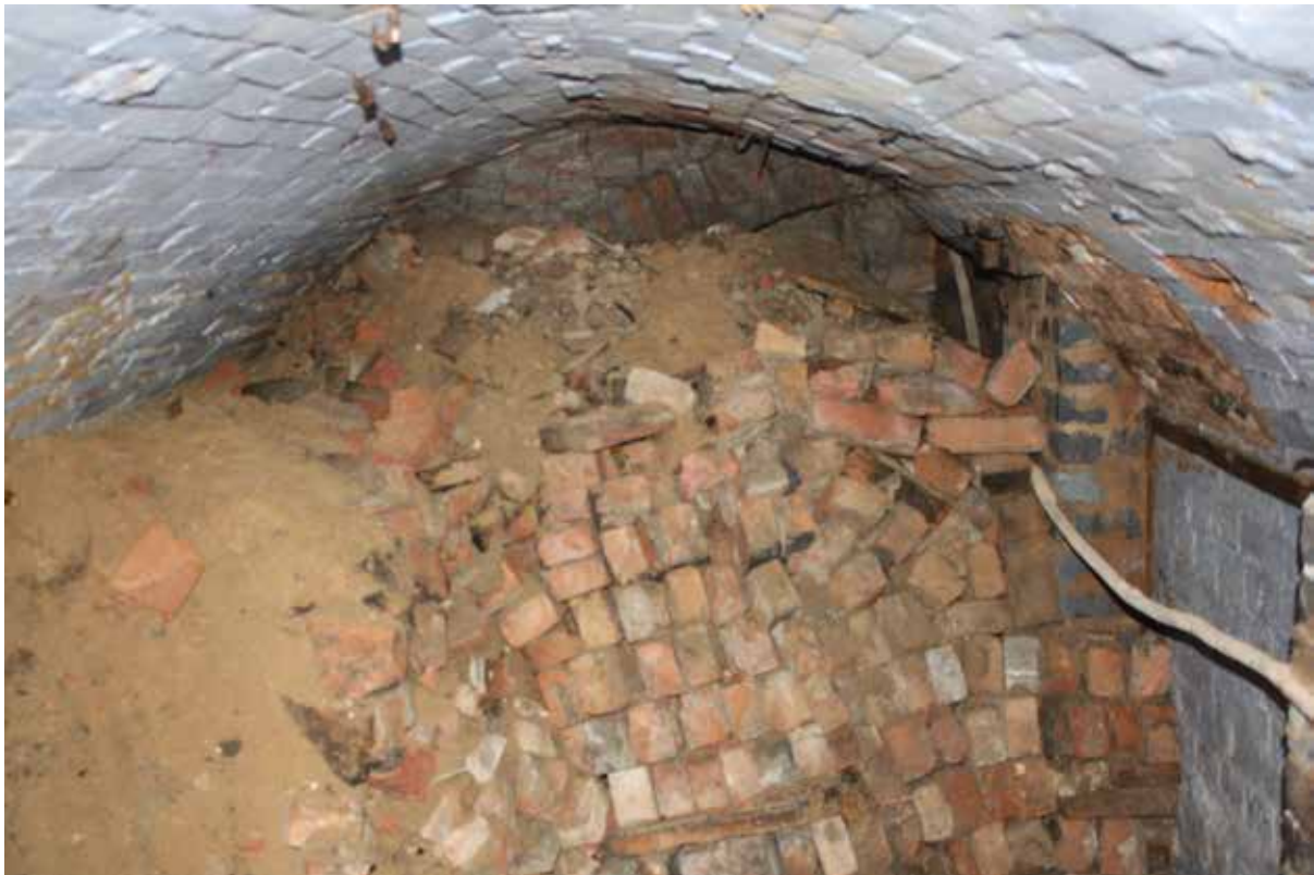
Plate 16: Cell 1, looking south, prior to exposure during ground reduction. Note the infilled material from a partial collapse as well as the arches in the background from earlier phases of construction. The bricks were loosely stacked as if being stored.
