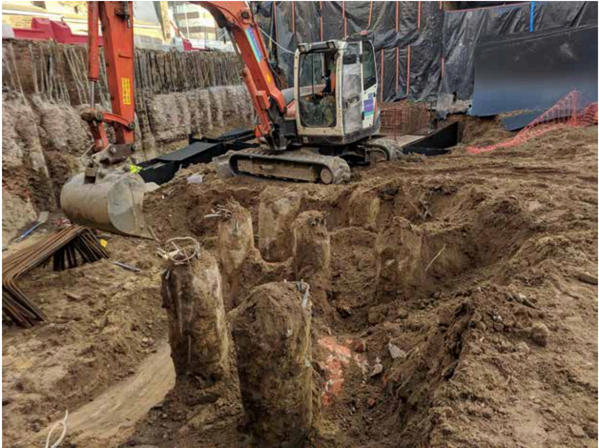
Plate 31: Site visit, facing north-east. In the foreground an area of piling can be seen, having truncated and largely destroyed a likely cellar structure.
