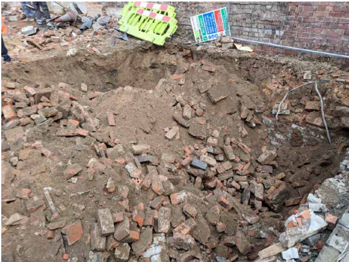
Plate 18: Partially backfilled and demolished cellars in the south-eastern corner of the site, facing north-east. It appears that the cellars were backfilled prior to demolition works on the site as well as being partially collapsed.
