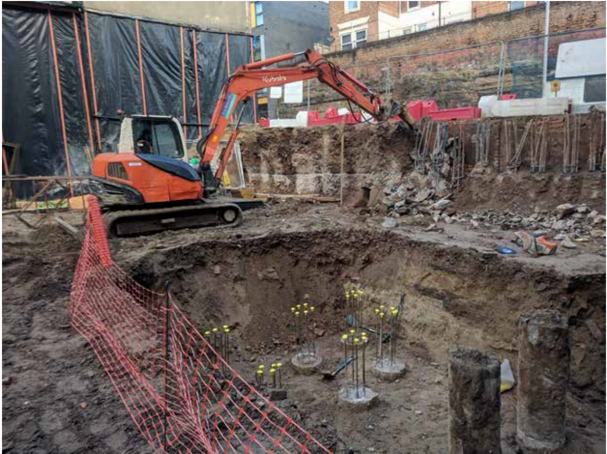
Plate 28: Site visit, facing north-west towards Wollaton Street. The sandstone bedrock (Chester Formation) can be seen in the foreground, behind the unreduced piles. The machine is exposing historical piling, which provided support for the retaining wall for Wollaton Street. Exposed sandstone bedrock can also be seen in the background of the image, on the northern side of Wollaton Street.
