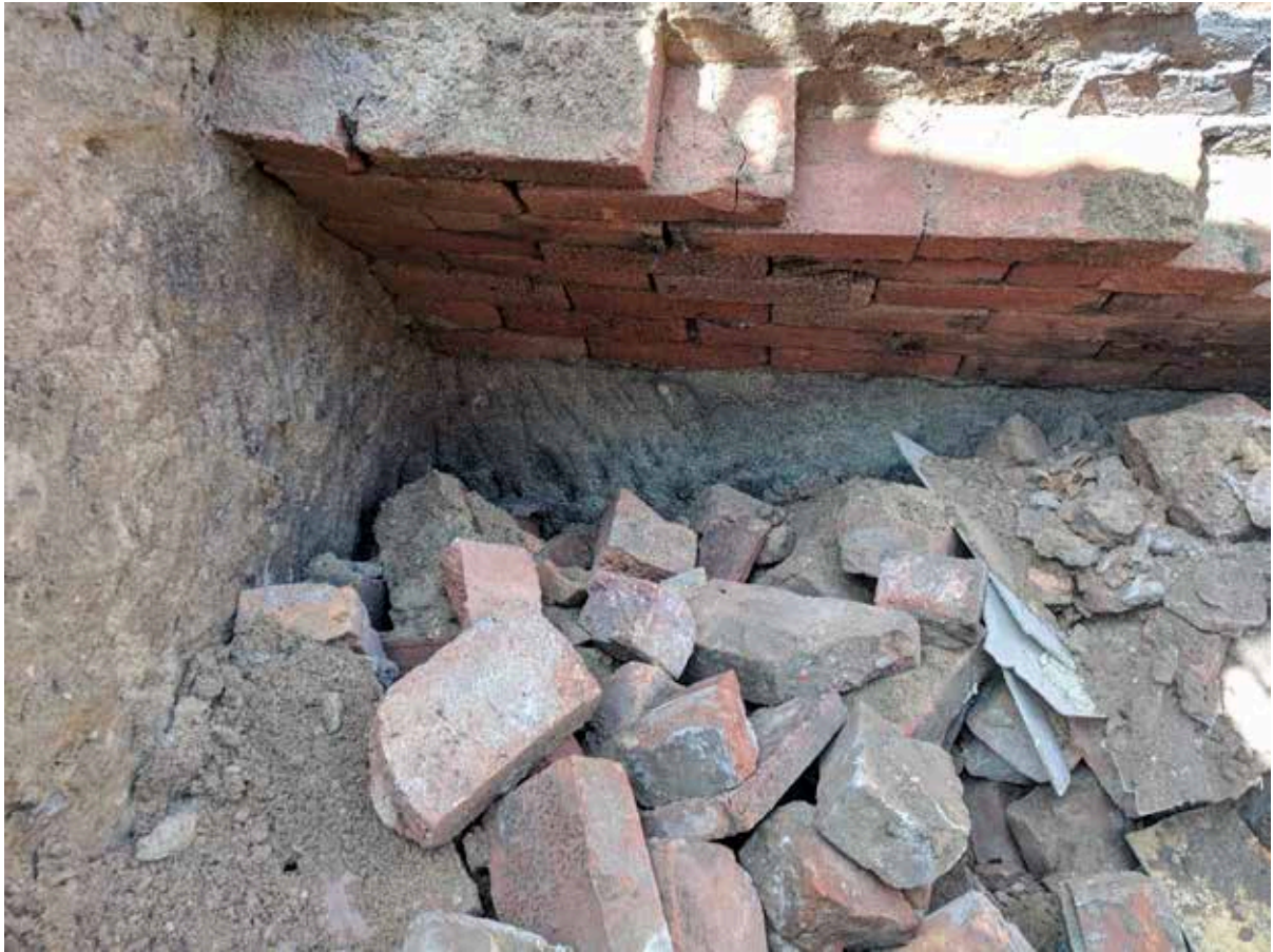
Plate 26: Detail of the rock cut wall and barrel vault bricks springing from the sandstone wall, facing west.
