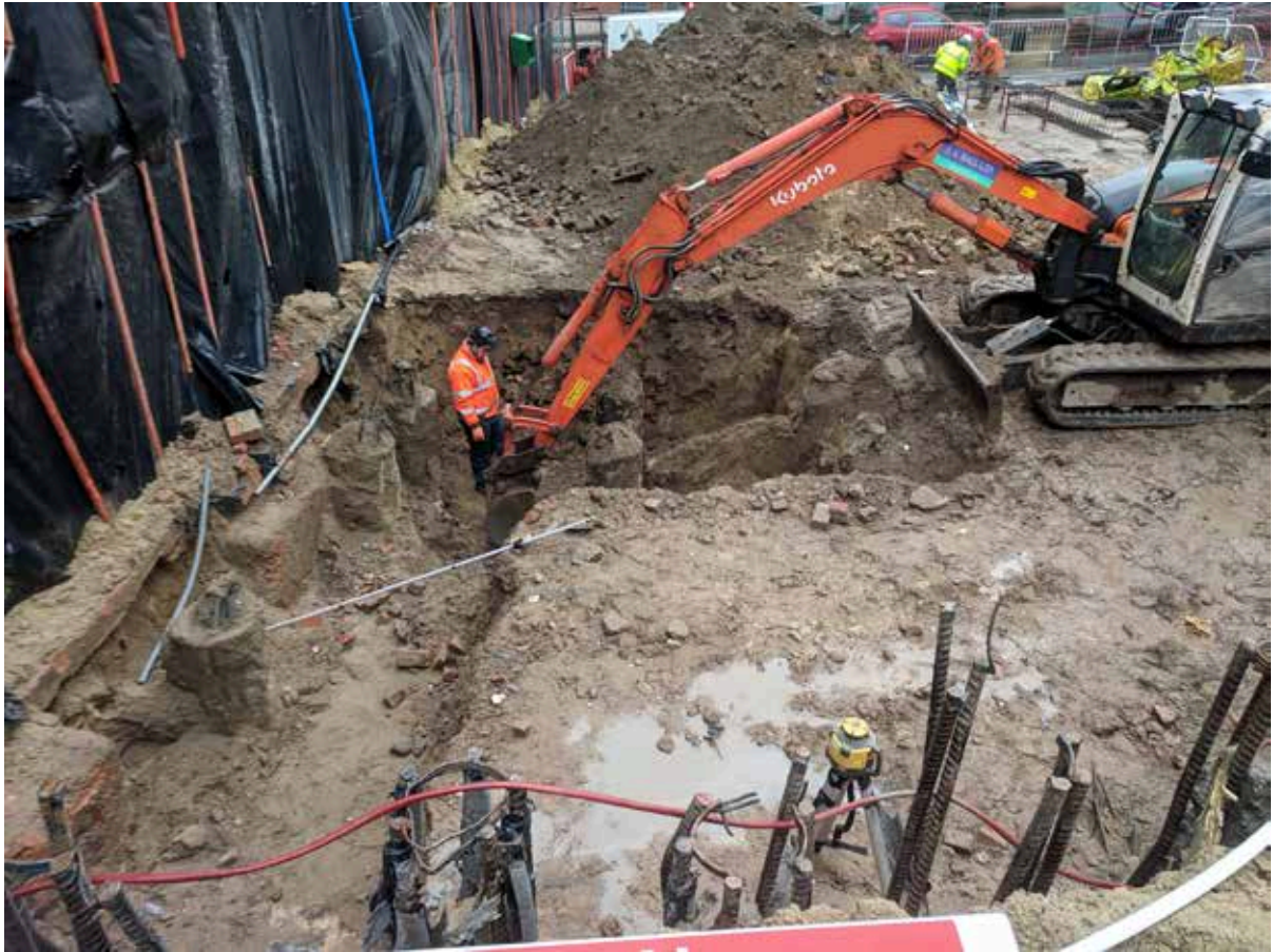
Plate 27: Site visit post-piling, facing south towards Derby Road, from Wollaton Street. The partially exposed brick arch can be seen to the west, behind the machine banksman.
