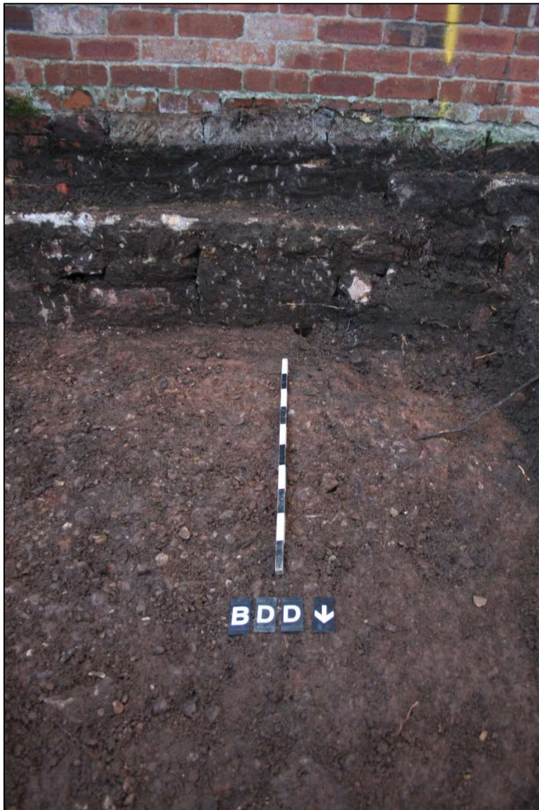
Plate 6: North facing section of trench showing the depth of foundations; looking south.
