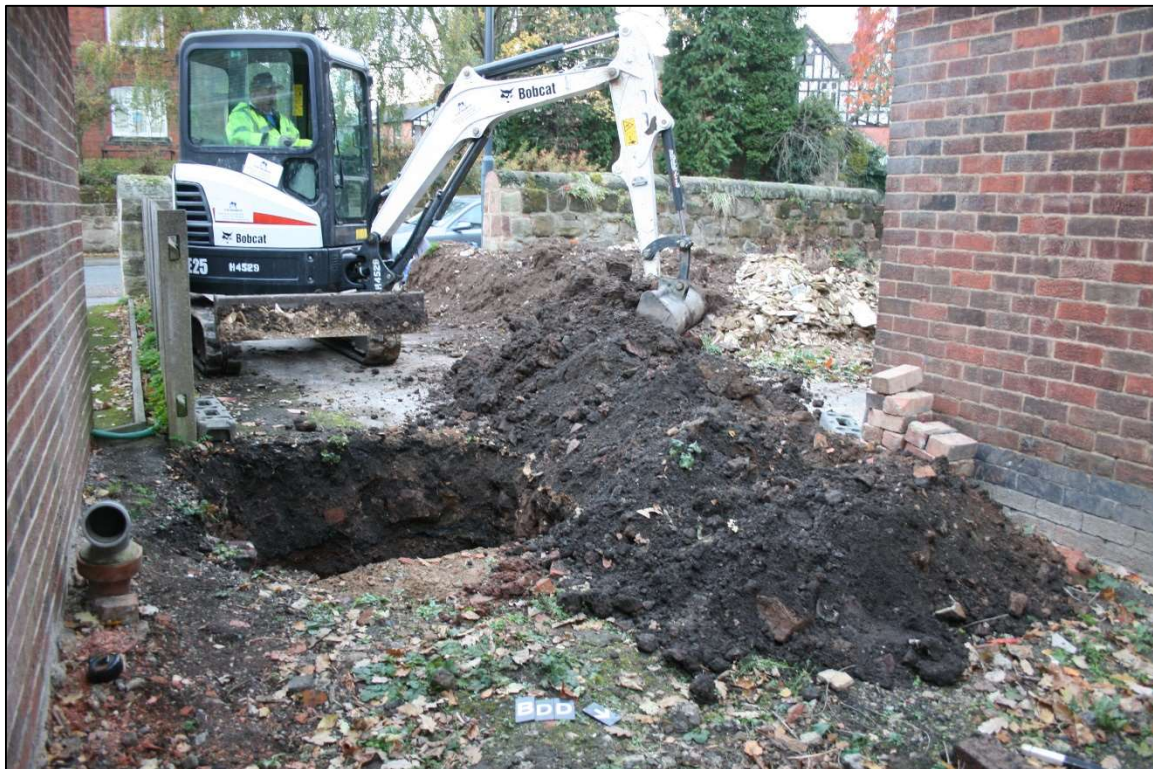
Plate 2: Excavation of the initial trial hole to find the total depth of foundations. Looking south-west
