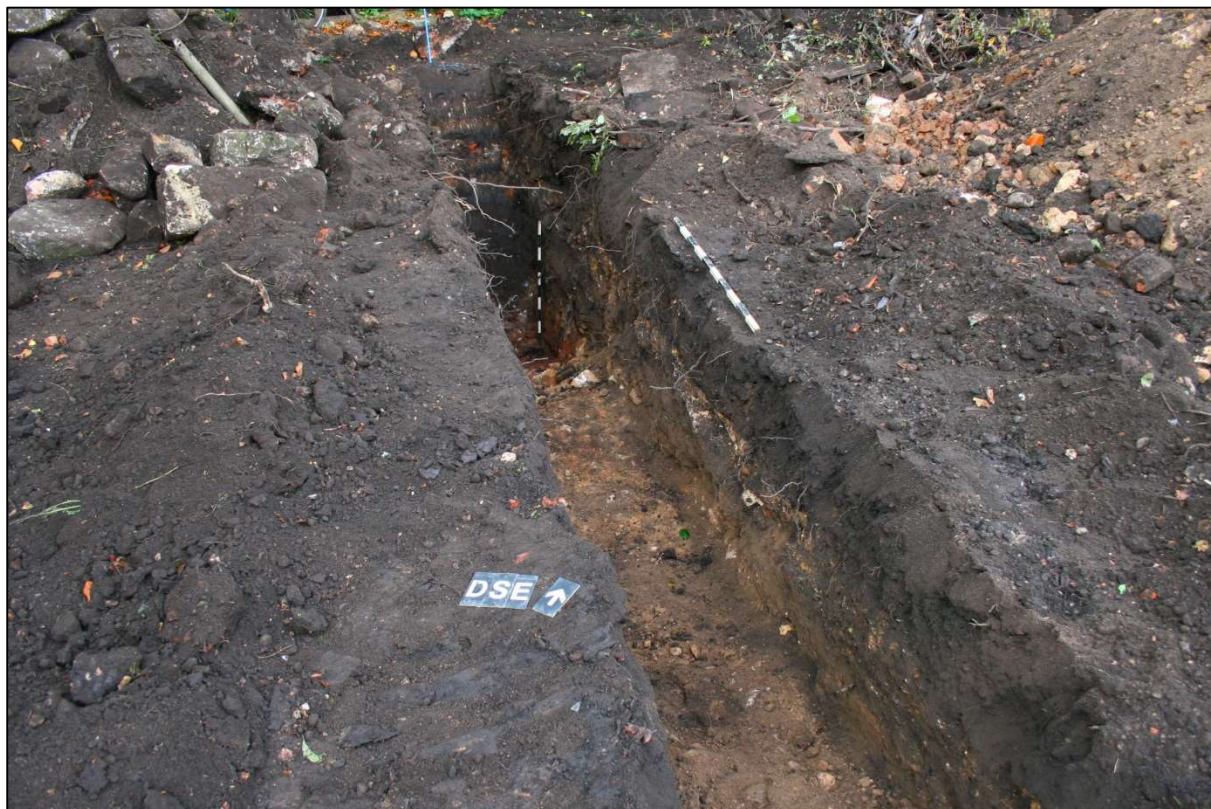
Plate 5: Representative image of trench footings, excavated to a depth of c.2m to the north-west of the site (incorrect sitecode: SBE), looking north-west. Scale 1m x 1m.
