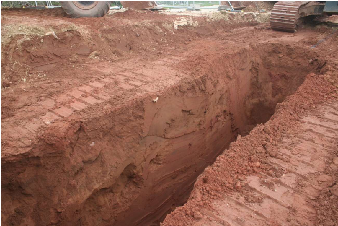
Plate 3: Excavation of additional drainage ditch to the south-east of the site. No scale.
