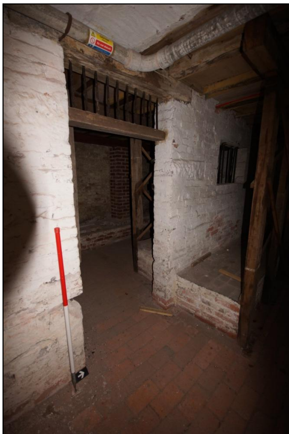
Plate 38: Inserted wall between Rooms C02 and C03, viewed looking north-north-west. Scale = 1m.
