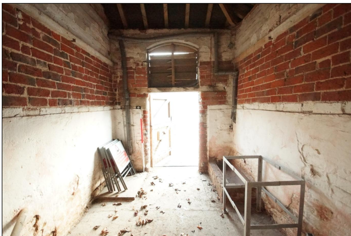
Plate 96: General view of the southern bay of Building 16, viewed looking east. Scale = 1m.
