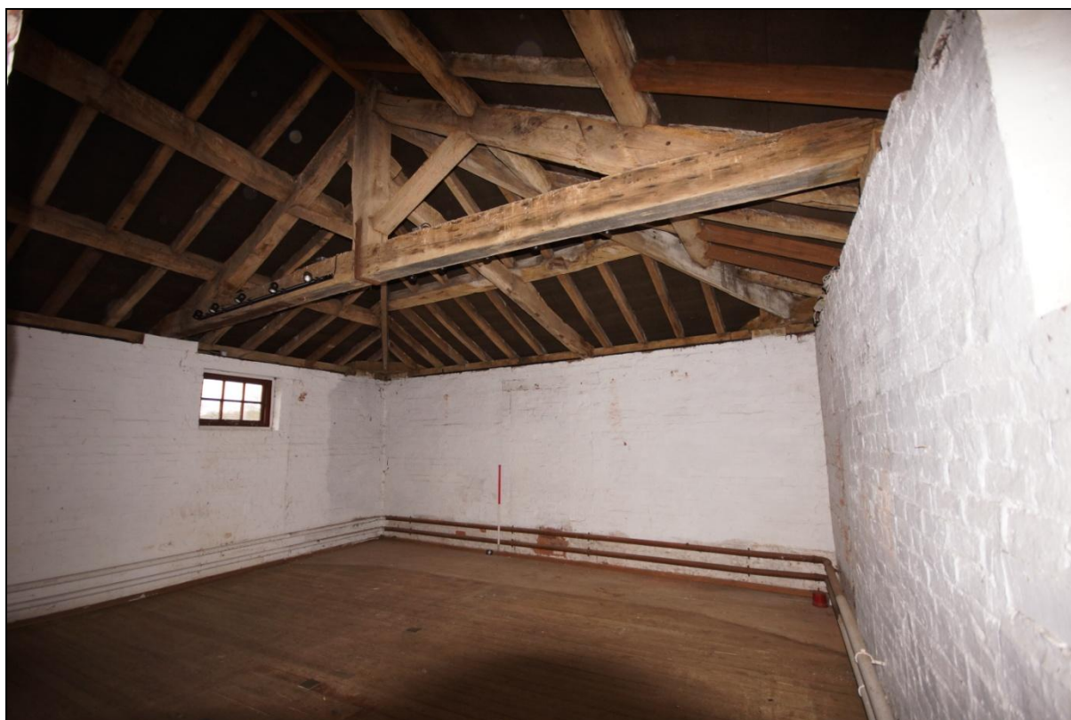
Plate 79: General view of the first floor of Building 12, viewed looking south-west. Scale = 1m.
