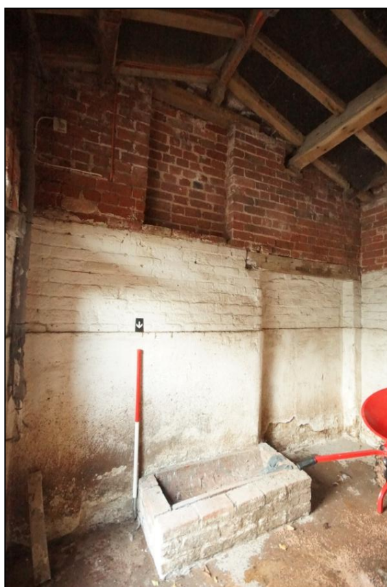
Plate 90: South wall of Building 13 showing the two blocked openings and the low brick-built trough, viewed looking south-west. Scale = 1m.
