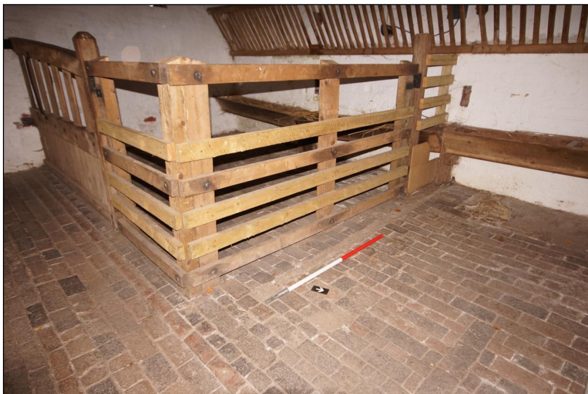
Plate 78: Central drain and former stall bed in the ground floor of Building 12, viewed looking south-west. Scale = 1m.
