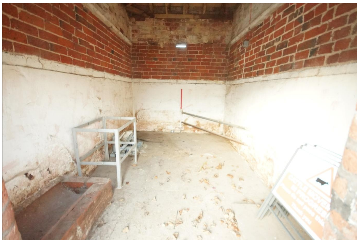
Plate 95: General view of the southern bay of Building 16, viewed looking west. Scale = 1m.
