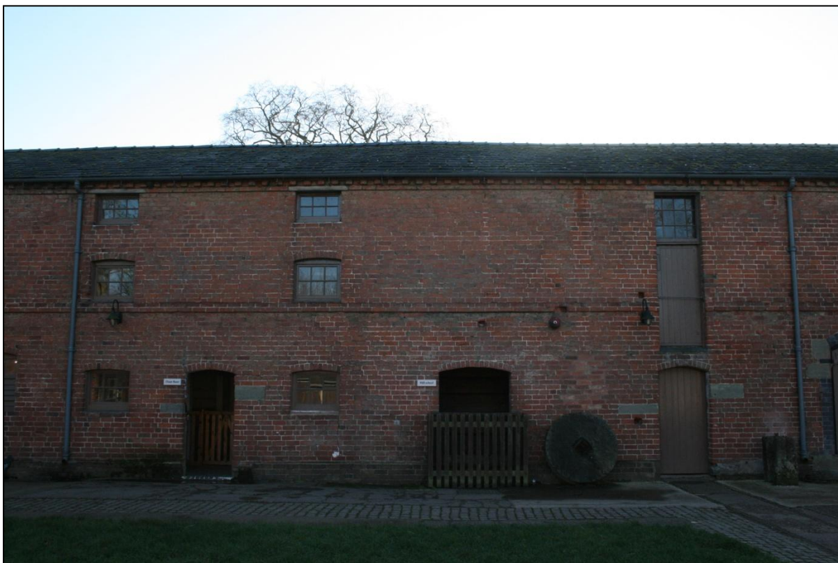
Plate 50: North elevation of Buildings 08 and 09 (The Water Corn Mill), viewed looking south.
