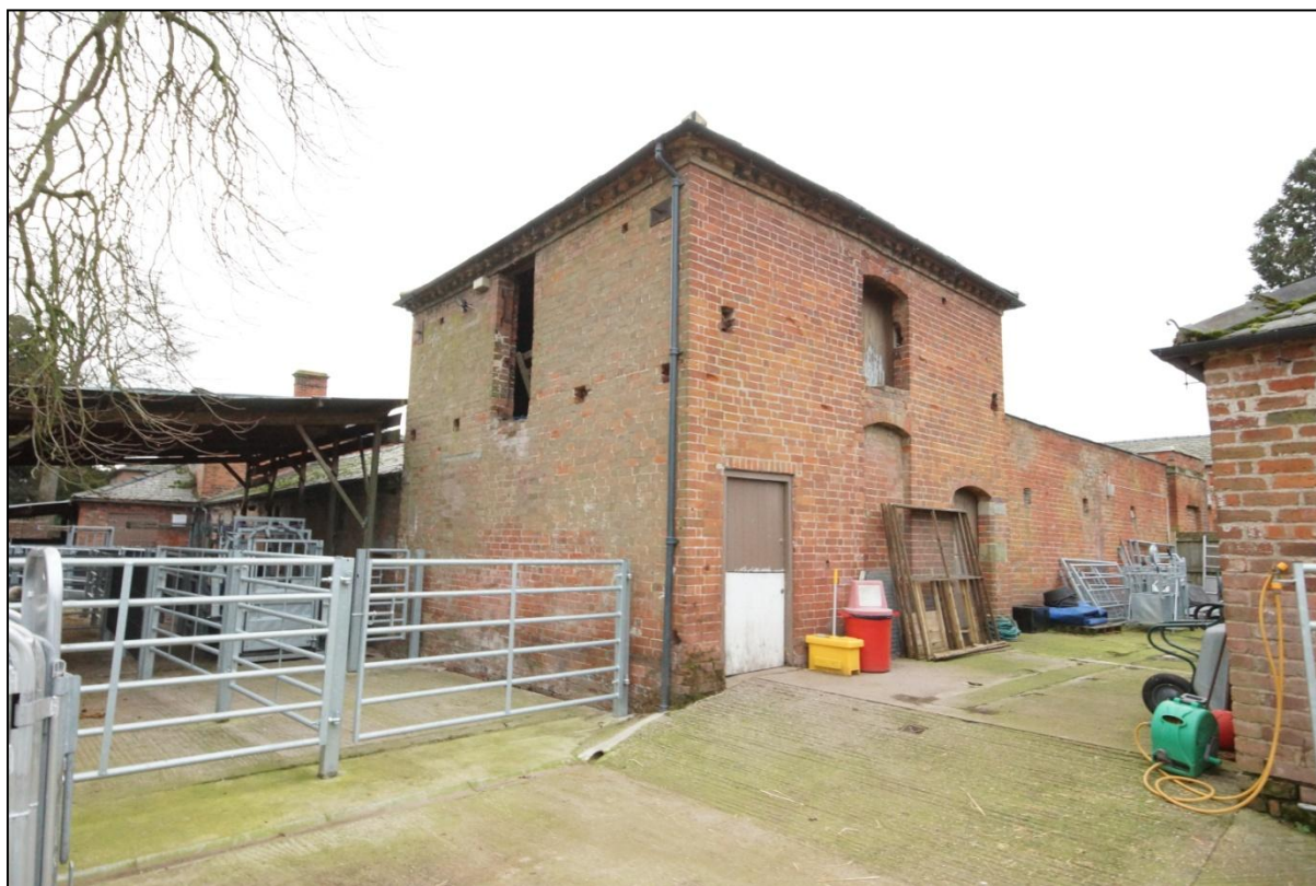
Plate 104: Oblique view of the north and west elevations of Building 17, viewed looking south-east.
