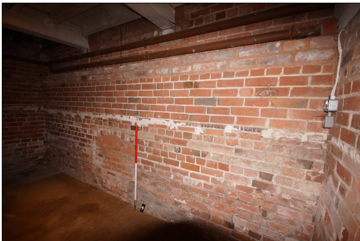
Plate 75: A course of perforated tiles and blocked opening within the north wall of the ground floor of Building 11, viewed looking north-west. Scale = 1m.
