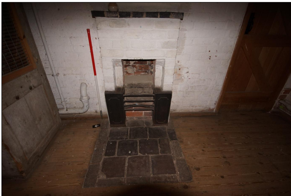
Plate 66: The fireplace within the east wall of the first floor of Building 08, viewed looking east. Scale = 1m.
