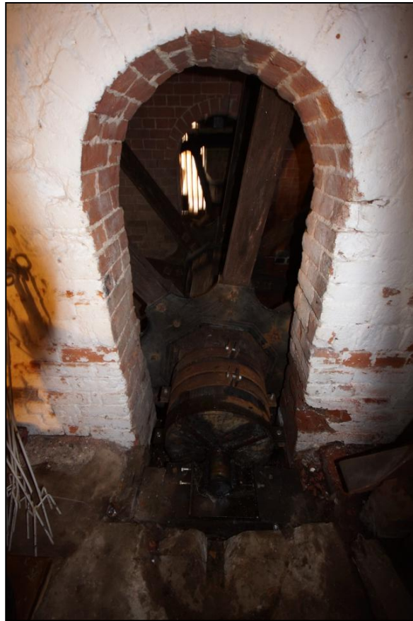
Plate: 69: Cog wheel within the east wall of the ground floor of Building 09, viewed looking east.
