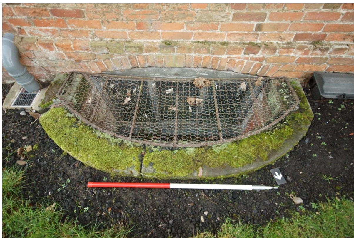
Plate 7: Cellar window in the north-east elevation of Building 01, viewed looking south-west. Scale = 1m.
