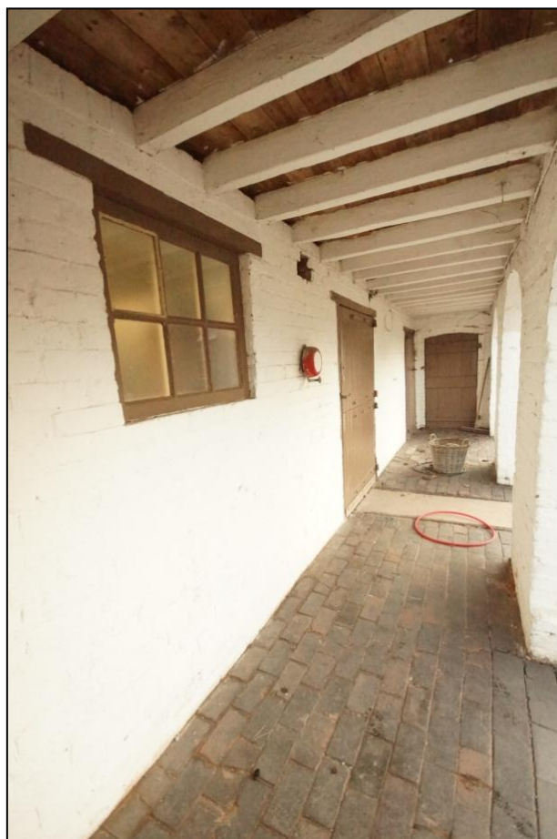
Plate 117: Inserted wall behind the arcade within the south elevation of Building 19, viewed looking east-north-east.
