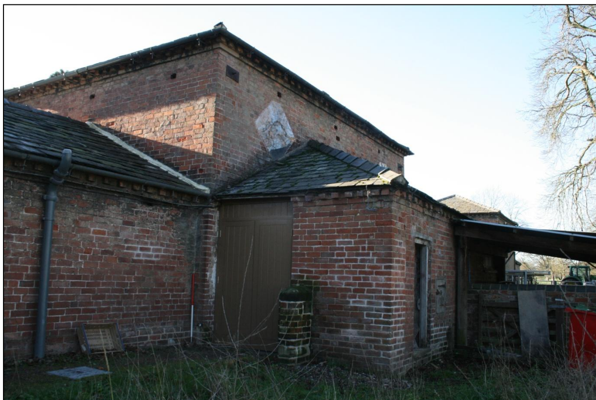
Plate 108: Oblique view of the north elevations of Buildings 19, 20 and 21, and the east elevation of Building 20, viewed looking south-west. Scale = 1m.
