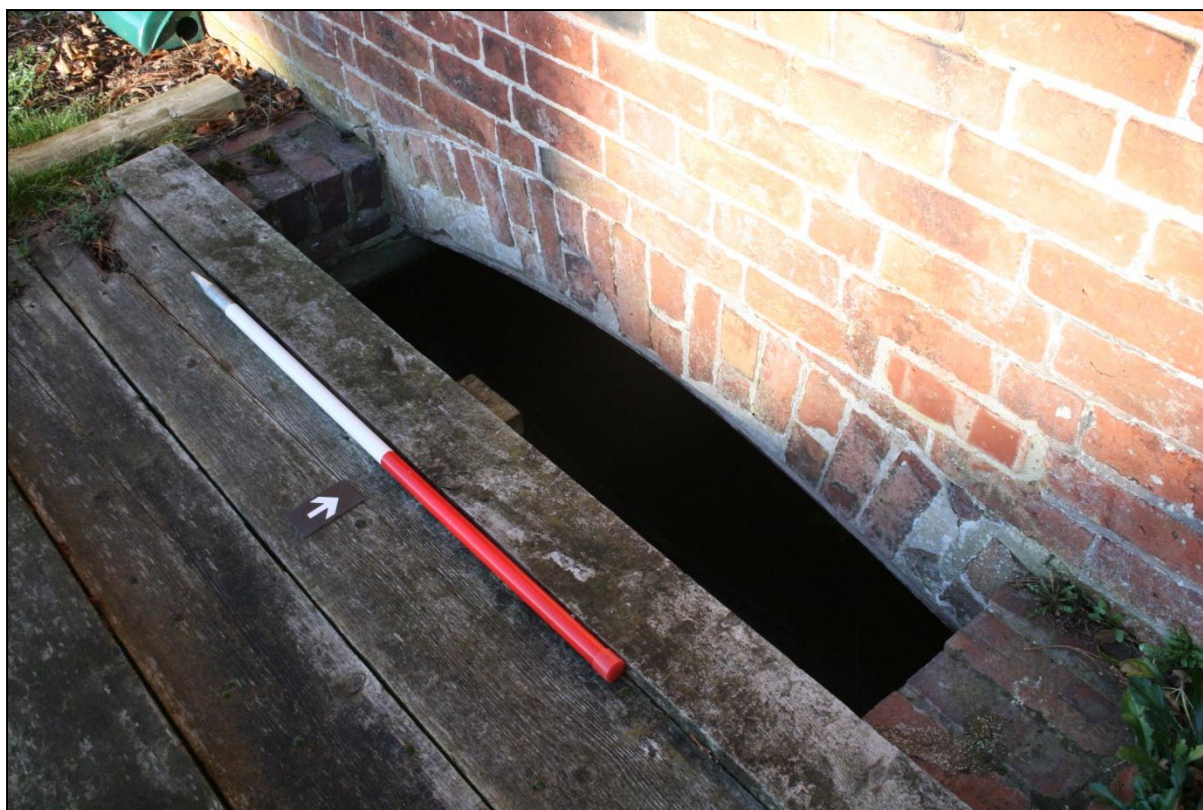
Plate 47: Opening within the south elevation of Building 09 for the water gates, viewed looking north-west. Scale = 1m.
