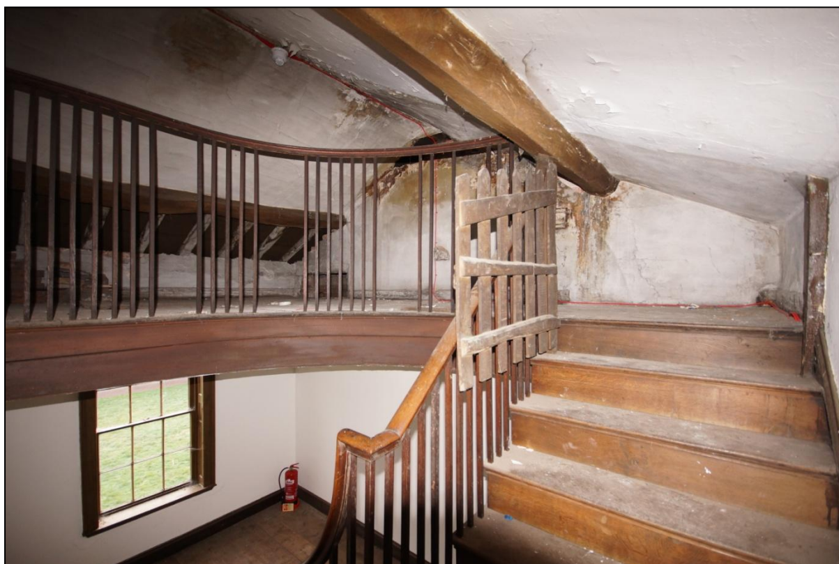
Plate 30: General view of the second floor of the Farm Steward's House, viewed looking south.
