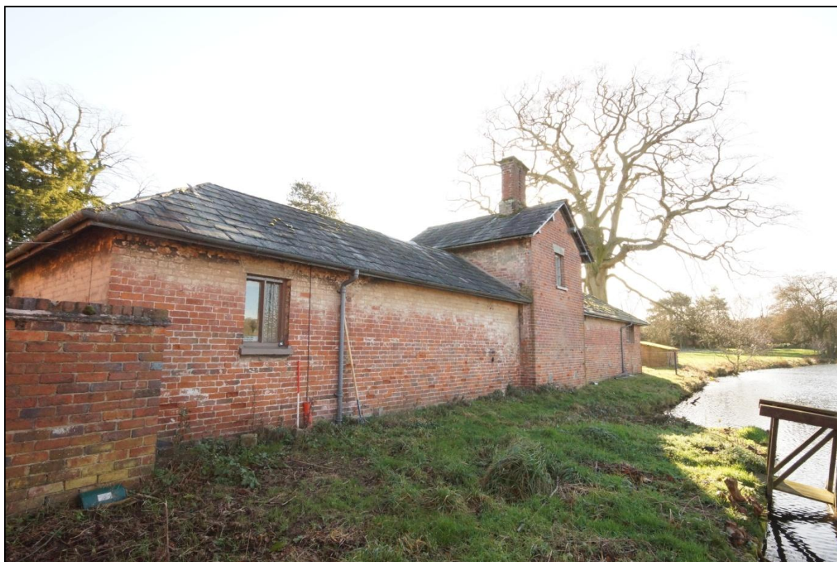
Plate 130: Oblique view of the North-west elevation of the Dairy Range, viewed looking south.
