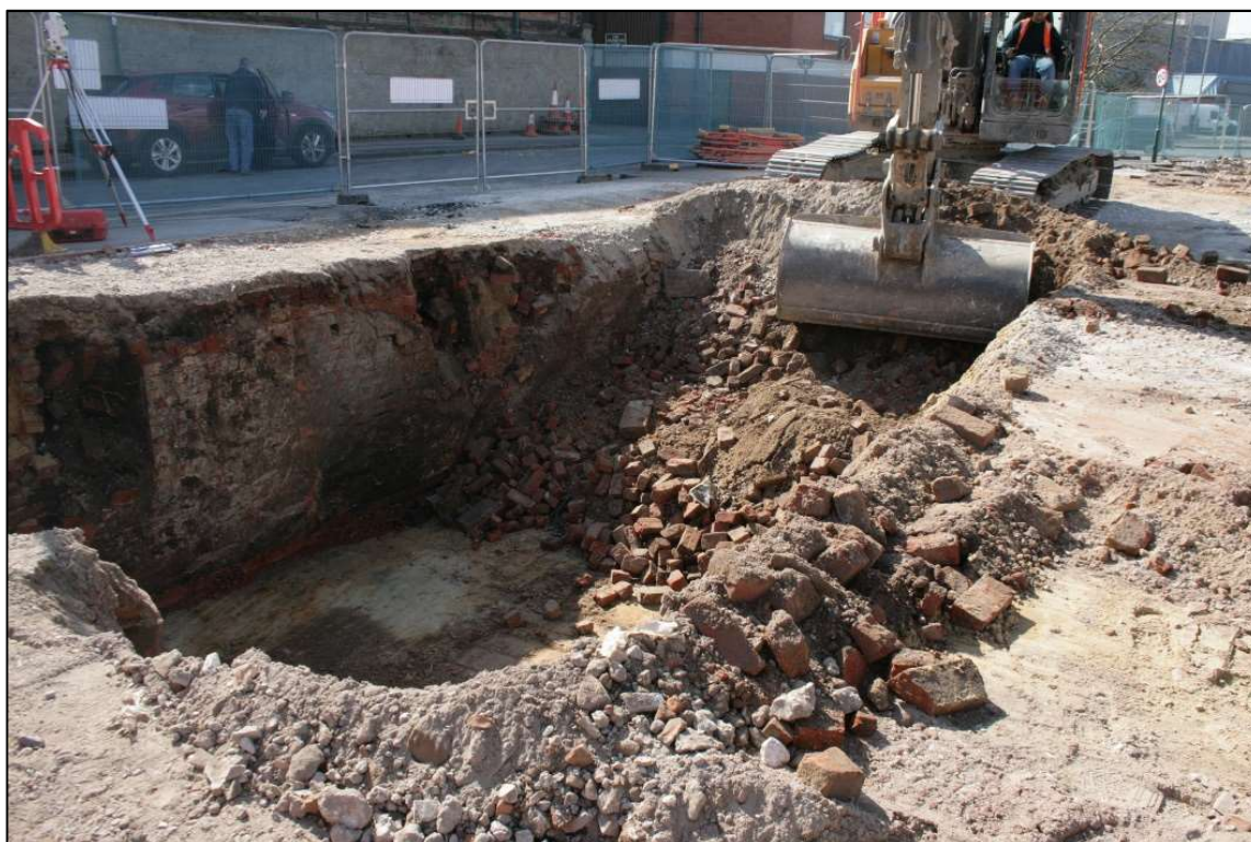
Plate 6: Block B showing wall structures associated with former terraced housing which fronted Great Freeman Street. No scale.
