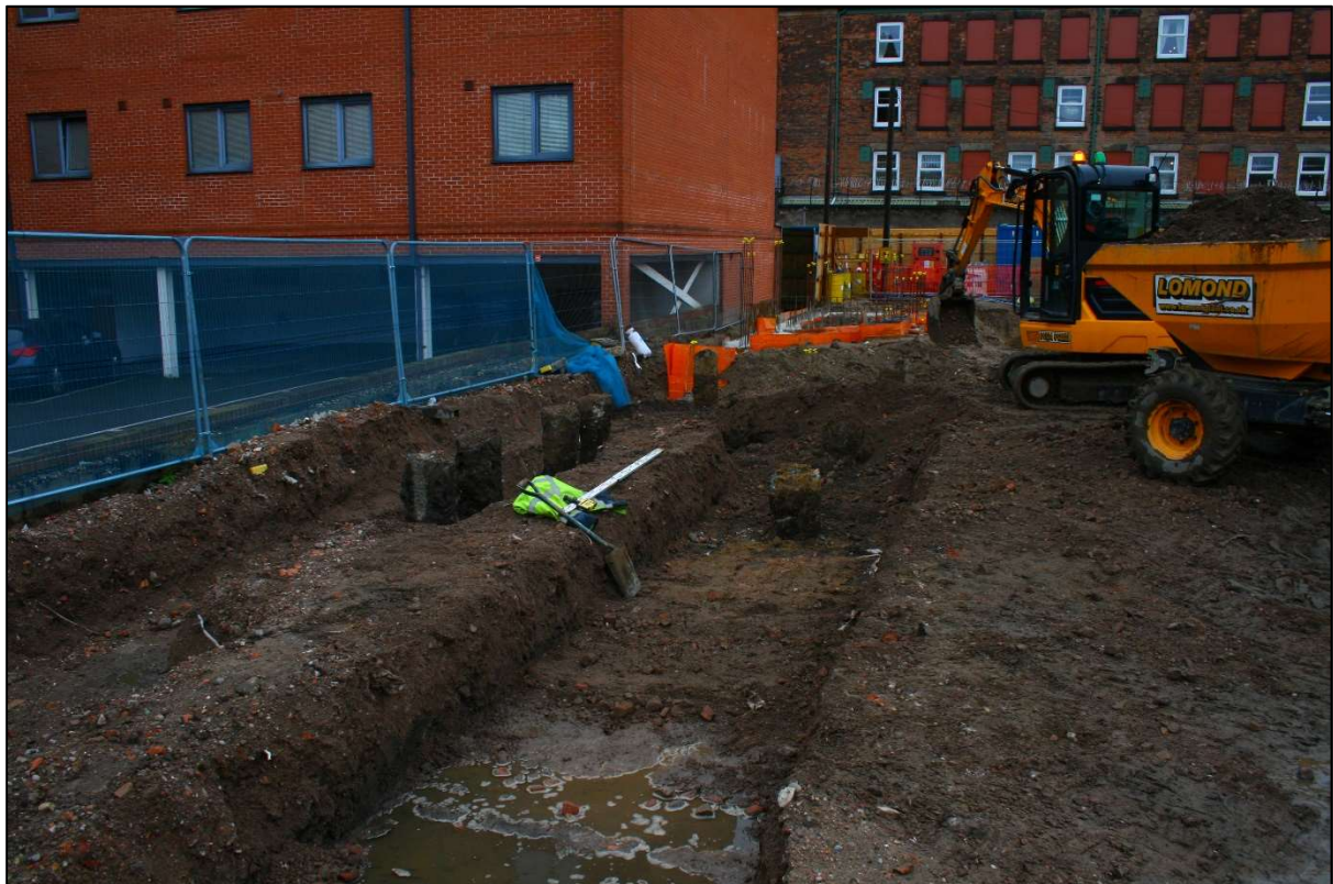
Plate 12: General overview of ground reduction within Blocks C & D. Looking north-east, no scale.
