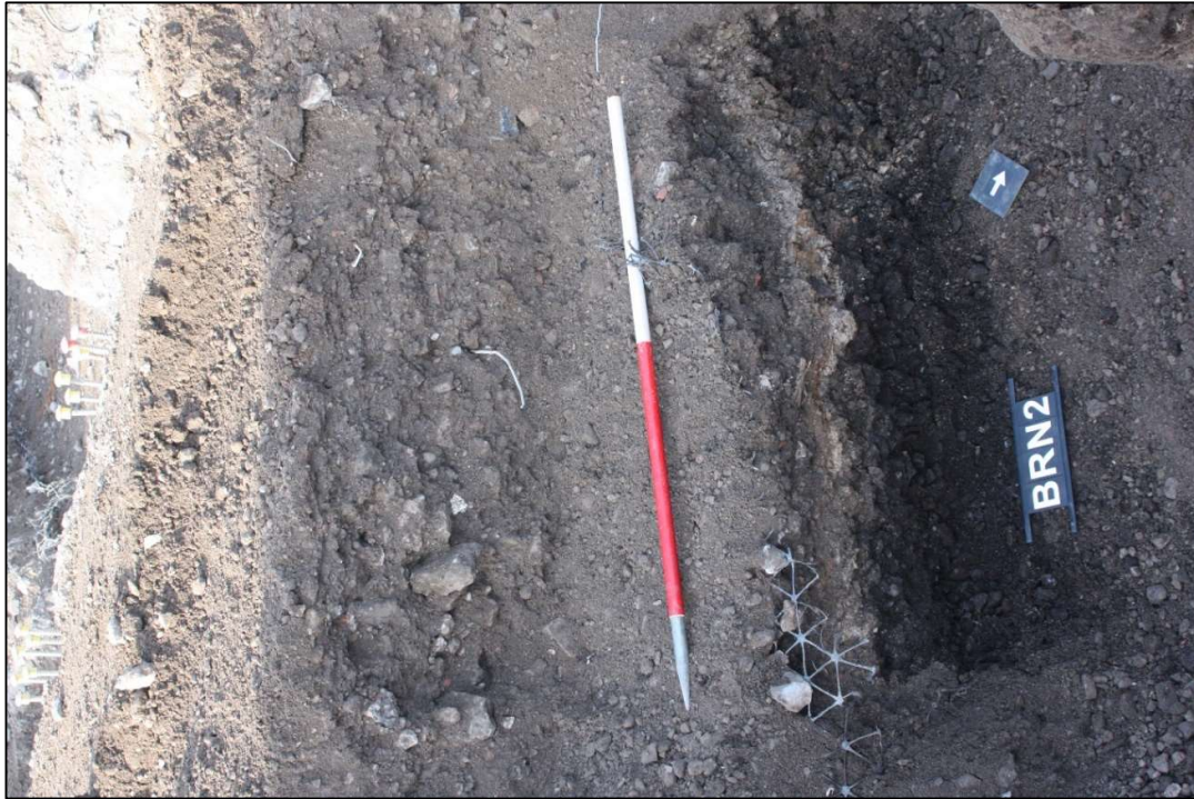
Plate 25: Watching brief: Piling phase. Example of below ground stratigraphy within the central portion of the site. Showing demolition and ground levelling material with a depth of c 1.8m. Scale 1m. Looking south-east.
