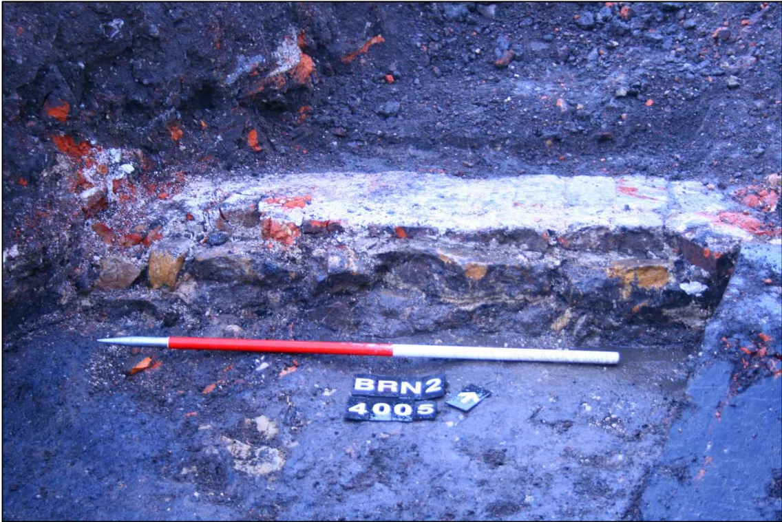
Plate 5: Trench 2, showing the remains of the probable medieval sandstone wall [4005], underlying 19th century housing foundations [4006]. Scale 1m. Looking north.
