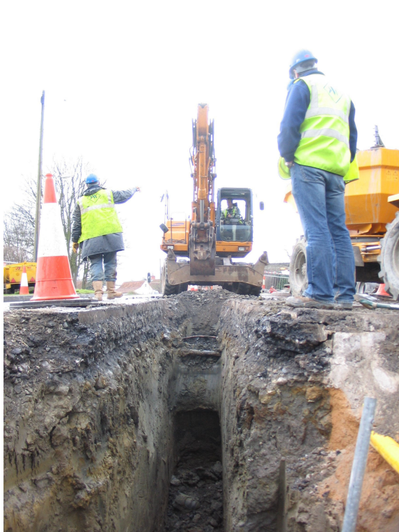
Fig 3. Photo of pipe trench showing level of visibility and technique of excavation of pipe trench through road ( Area 06).
