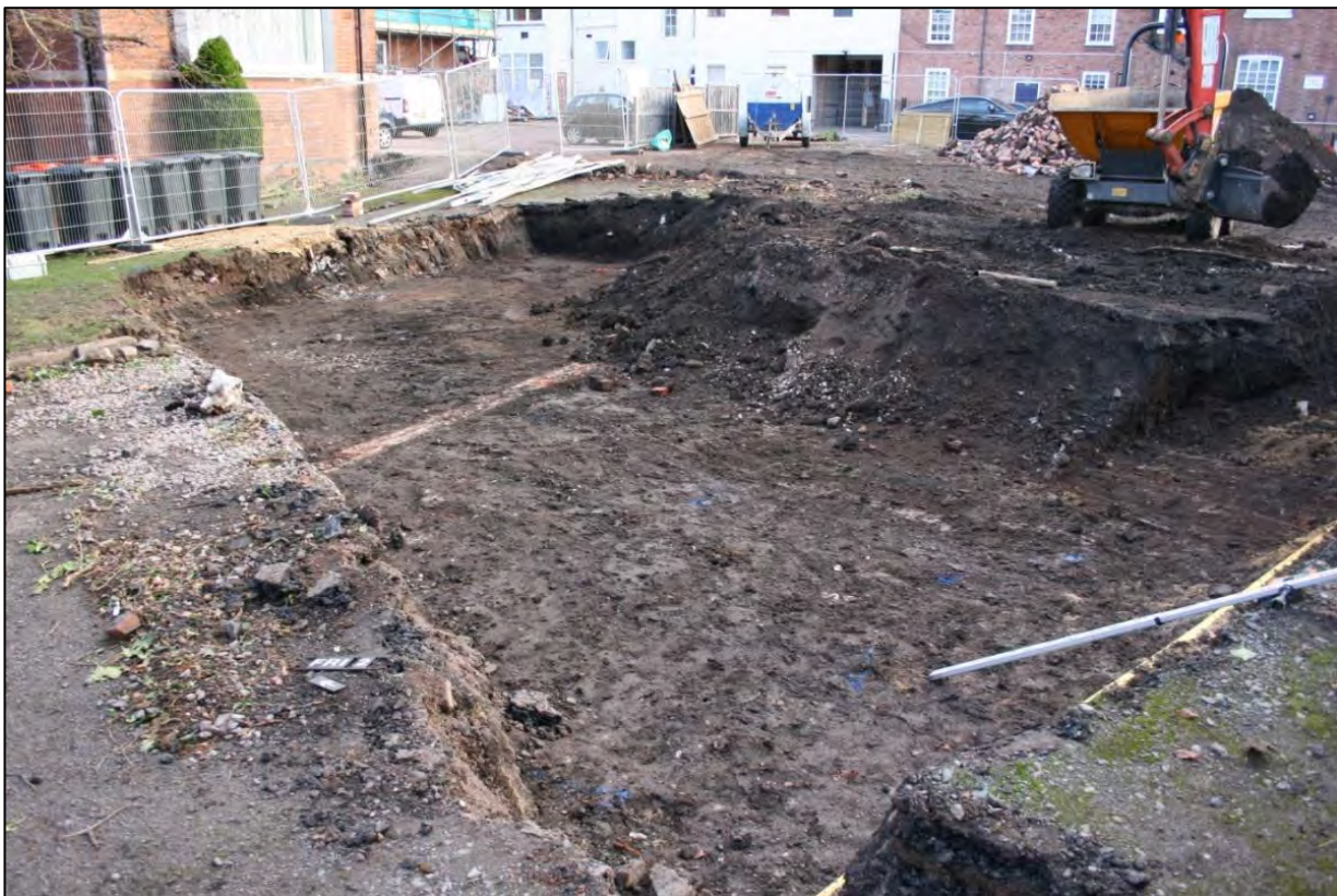
Plate 5: General site overview showing housing foundations within the northern portion of the site. looking northeast.
