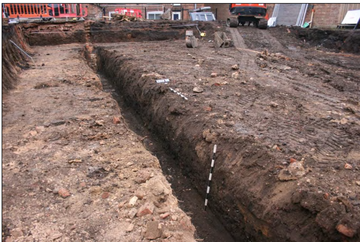
Plate 20: Located within the central portion of the site, after removal of early 19th c garden wall (2039). East facing section showing c.300mm of mixed 18th/19th c. construction/demolition material overlying a black silty soil (actual 18th ground level). Scale 2 x 1m
