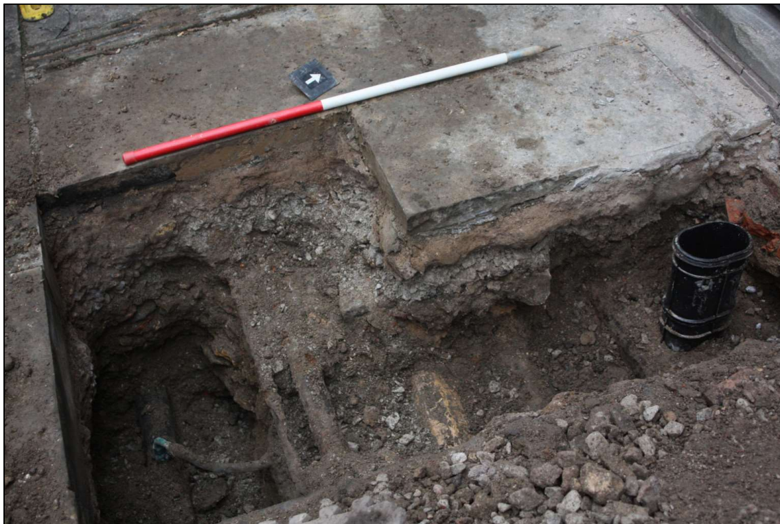
Plate 1: Area of excavation showing east facing section and service pipes in plan, oblique view. Scale 1m, looking north-west.
