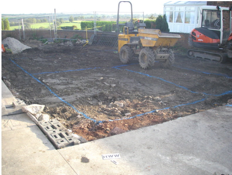
Plate 1: View looking across the site in a N-E direction prior to excavation of foundation trenches
