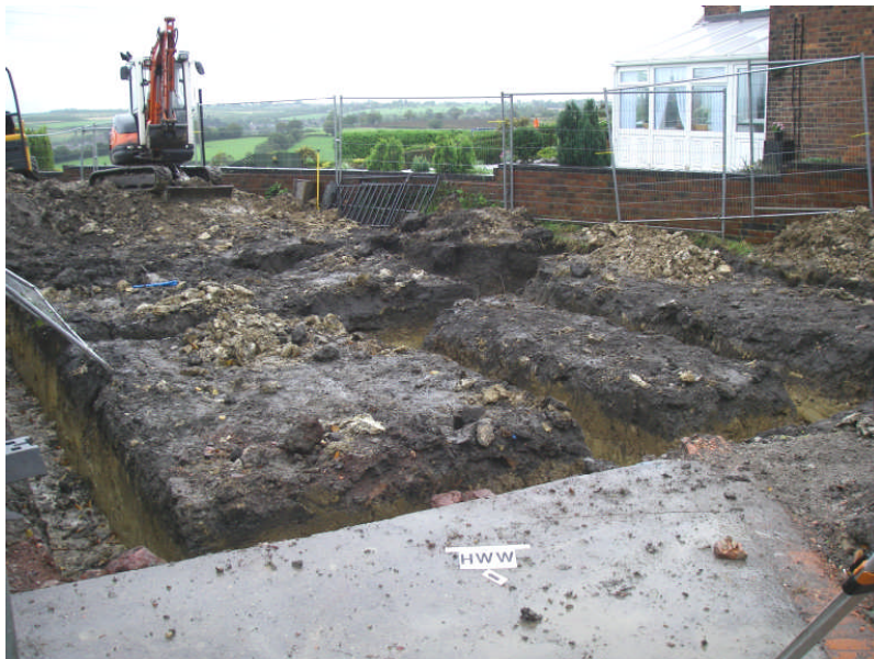
Plate 2: View looking across the site in a N-E direction after foundation trenches completed
