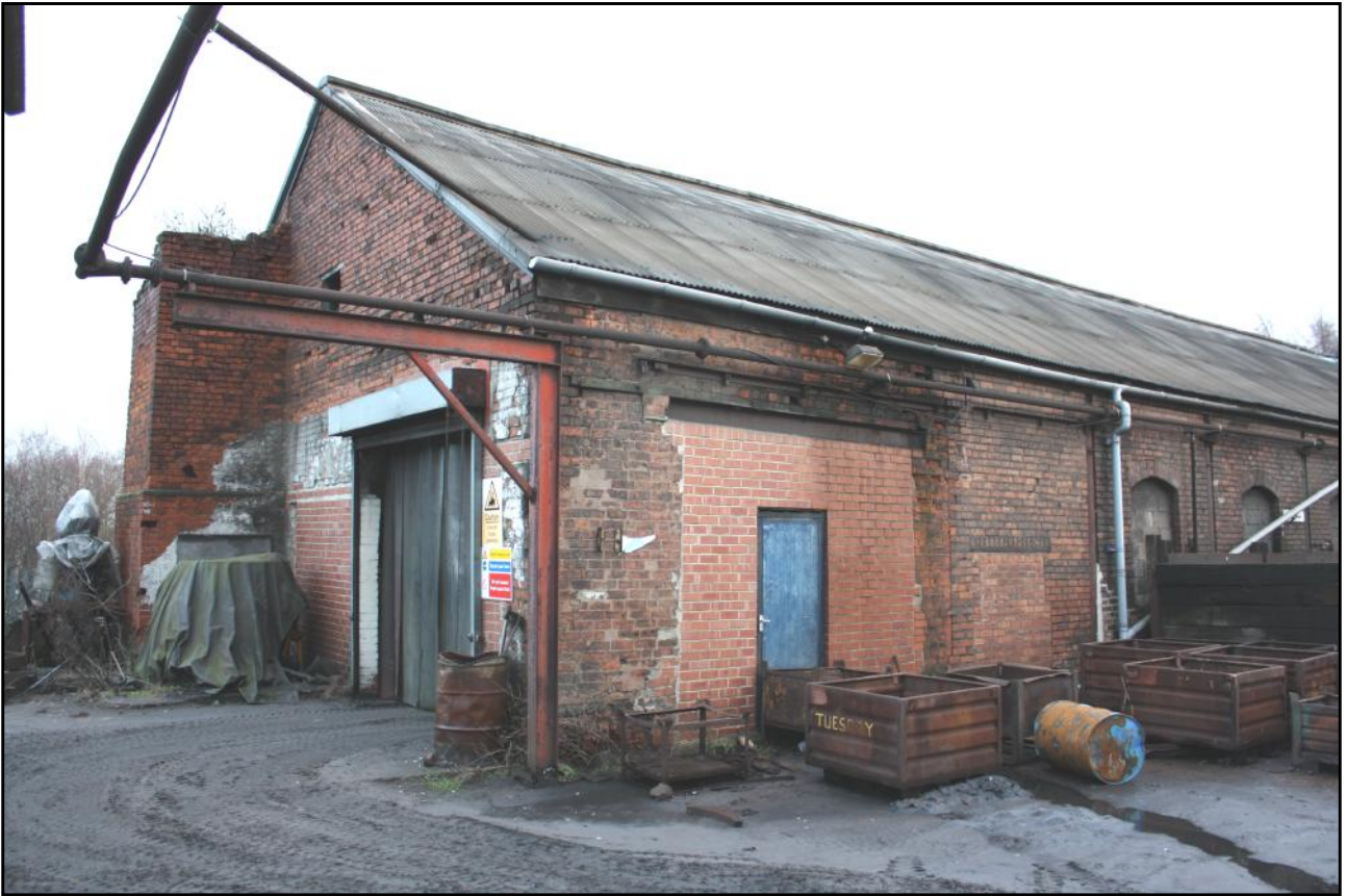
Plate 14: The Canlin Castings Ltd site at Langley Mill: north end of Building 7A showing the base of a large chimney, the scar of a former lean-to and, to right, part of the west frontage with infilled former openings and cast iron pillars showing to far right.
