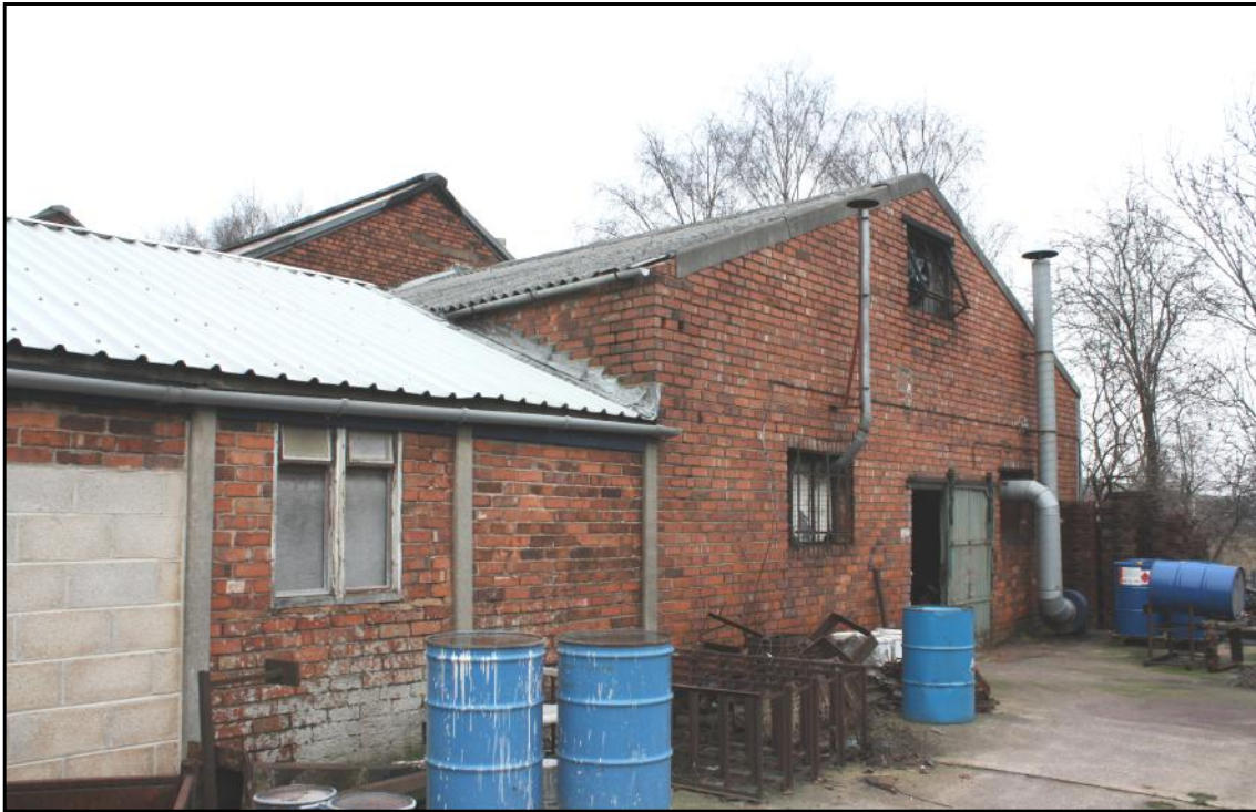
Plate 20: The Canlin Castings Ltd site at Langley Mill: south end of Buildings 7E (to right) and 7F (to left).
