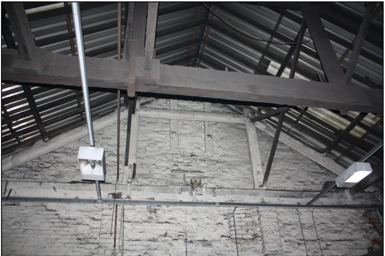
Plate 13: The Canlin Castings Ltd site at Langley Mill: queen-post timber trusses in Building 6A, as originally used in all the pre-1900 structures on the site.
