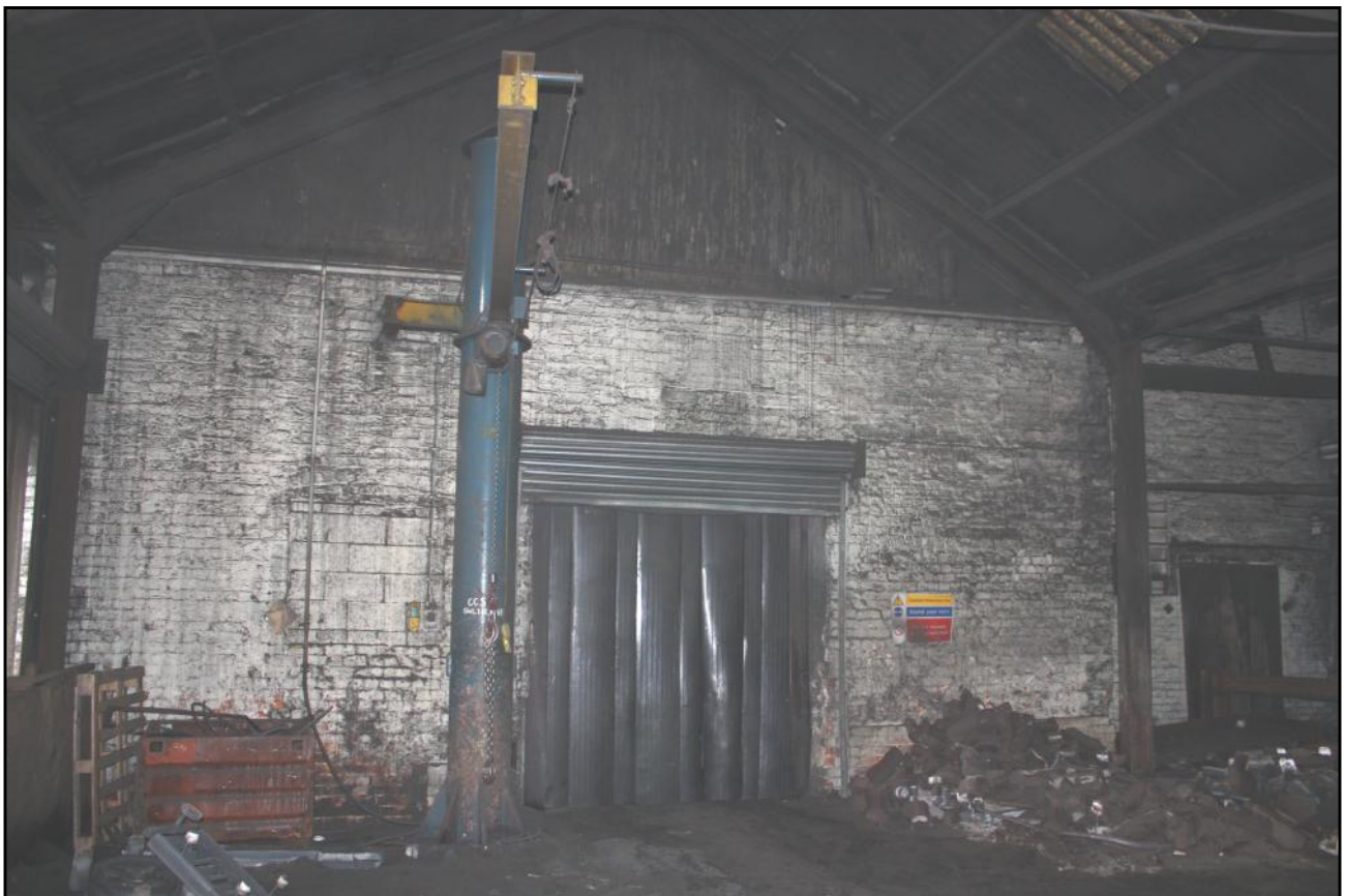
Plate 9: The Canlin Castings Ltd site at Langley Mill: north end of Building 6A (with blocked window to left) and metal roof truss of now largely rebuilt Building 6D.
