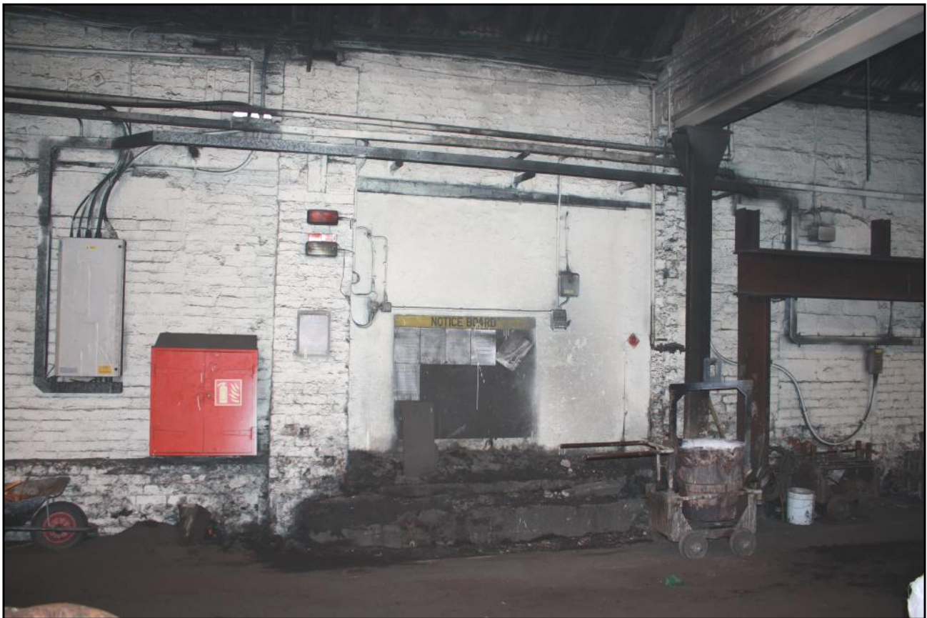
Plate 17: The Canlin Castings Ltd site at Langley Mill: base of a former external cupola furnace showing in the west wall of Building 7B.
