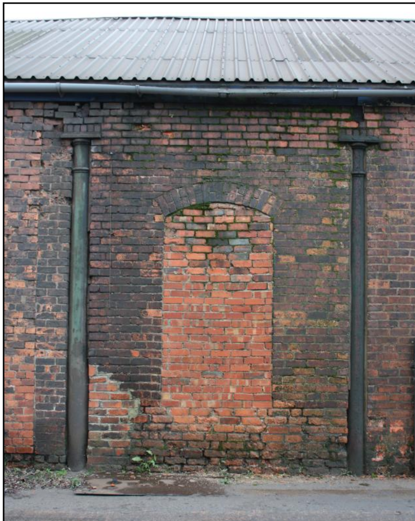
Plate 11: The Canlin Castings Ltd site at Langley Mill: exposed cast iron pillars showing in the east external wall of Building 6A, with straight joint to extension 6B showing to far left.
