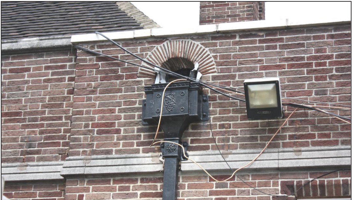
Plate 5: Decorative cast-iron rainwater head on the rear frontage of the Bull's Head public house, Hanford, Staffordshire.
