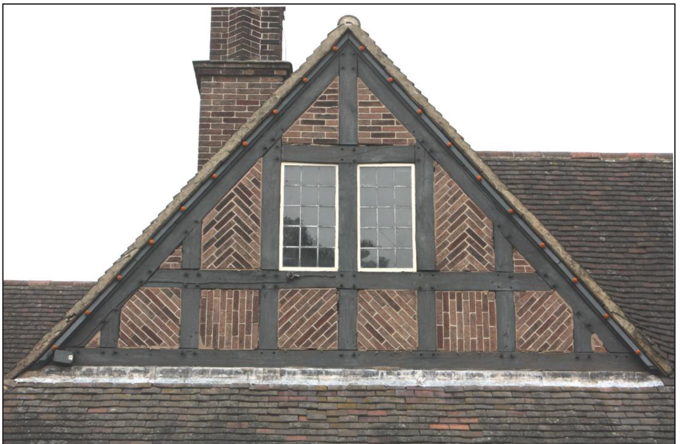
Plate 4: View of brick infill (nogging) to timber panels and the last remaining original leaded lights in an attic window in the south-east gable-end of the Bull's Head public house at Hanford, Staffordshire.
