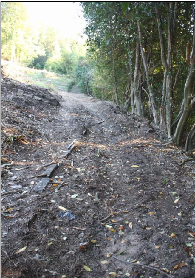
Plate 21: Surviving base stones of a former wall on the east side of the lower rail track, close to where it has been lost.
