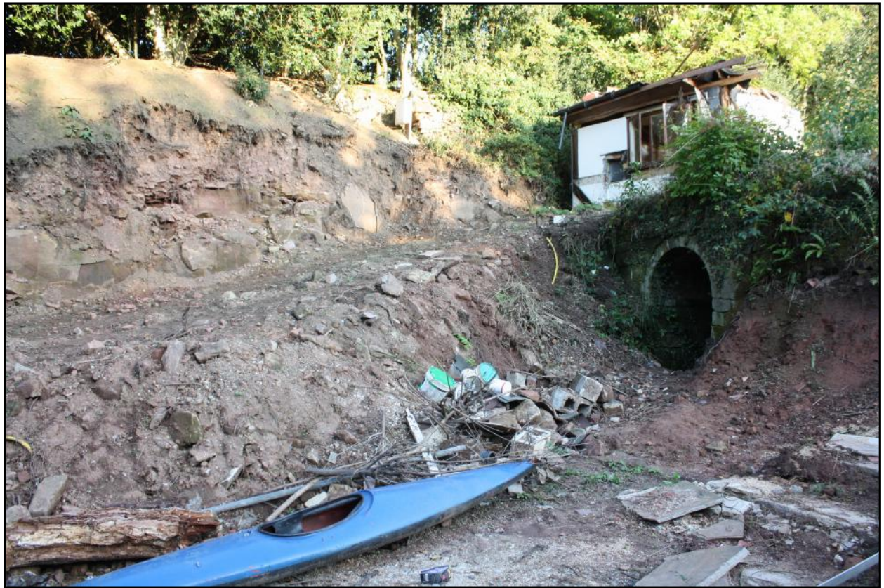
Plate 11: The north end of the Long Tunnel at Loner's Lair, Duffield Bank in October 2010.
