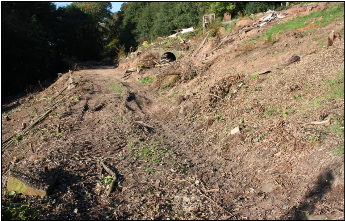
Plate 8: View looking northwards towards the south end of the Long Tunnel at Loner's Lair, Duffield Bank after the clearance of vegetation and the demolition of The Bungalow (top right) in October 2010. Original edging still shows where the ranging rod is standing.
