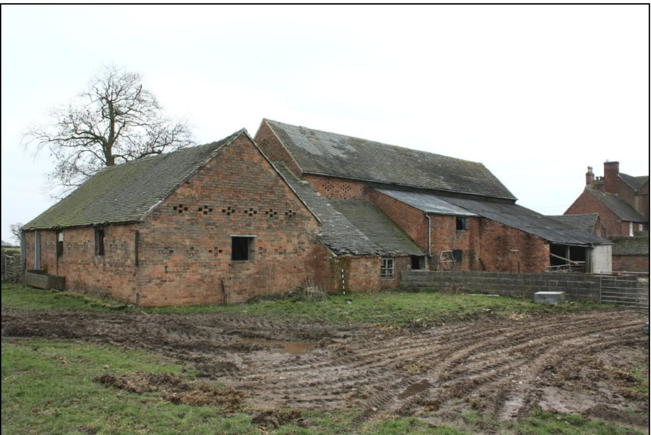
Plate 11: View looking south-east showing the two-storey original part of the north range and other additions on the north and west sides. The former farmhouse shows far right.
