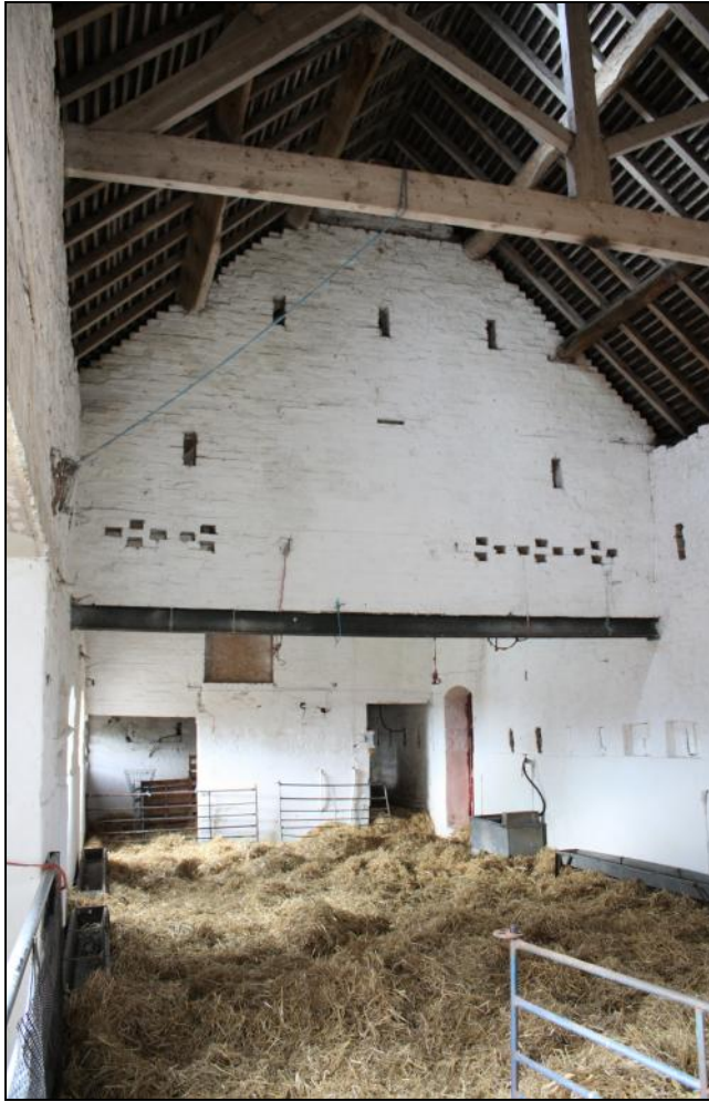
Plate 7: View of Rooms 4 and 5 in the central range of Pastures Farm showing a missing upper floor, vents within an internal wall and a king-post roof structure.
