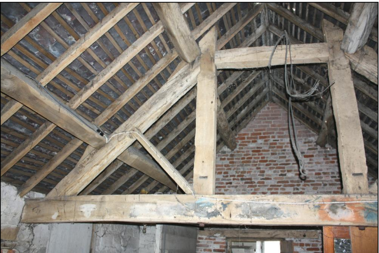
Plate 6: The upper floor of Room 2 showing the staircase (bottom left), a queen-post truss and internal brick walling.
