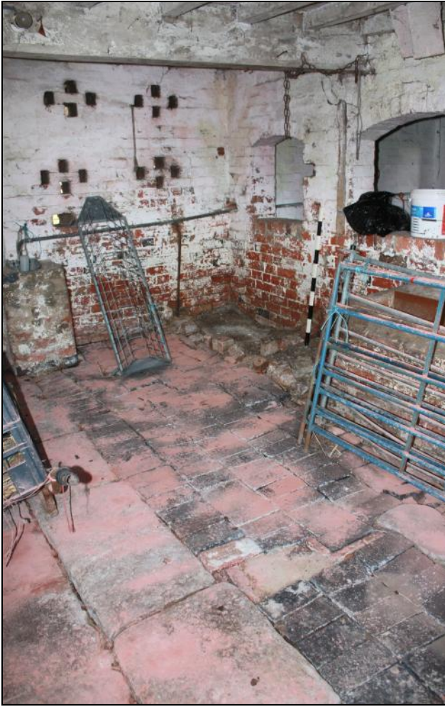
Plate 12: View of Rooms 1 in the north range of Pastures Farm, showing stone flagged floor, arched openings in the internal wall and diamond-shaped vents in back wall.
