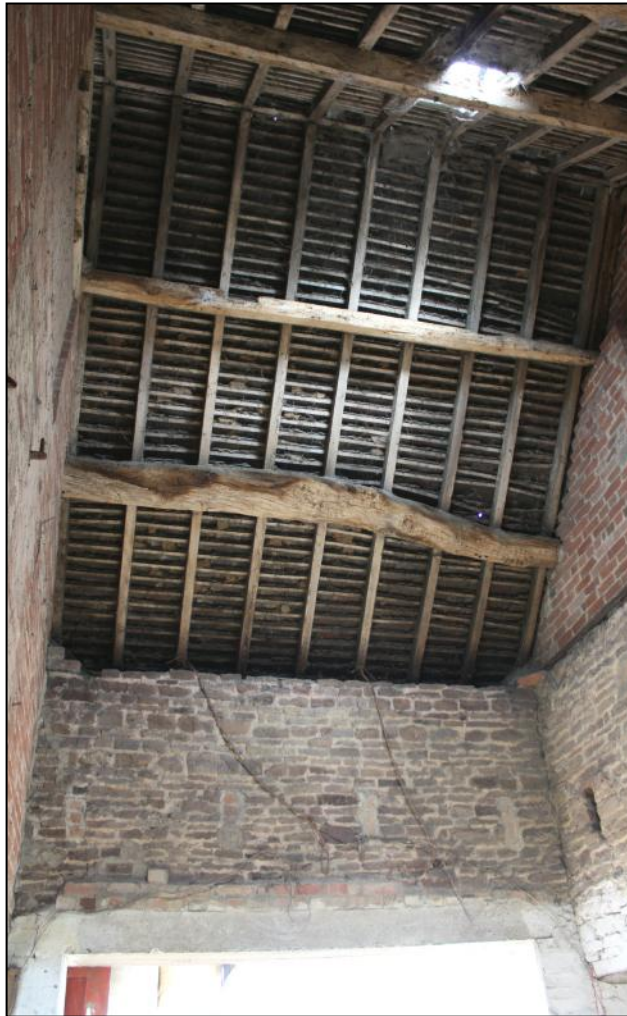
Plate 8: Roof structure above Room 6, the east end room of the original part of the central range.
