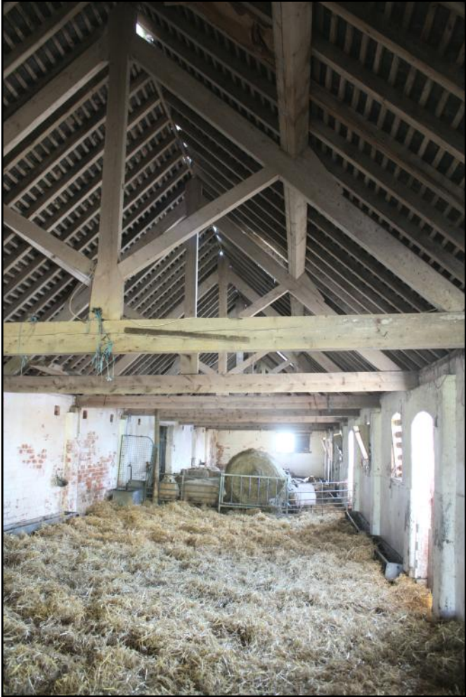
Plate 18: Internal view of the open 9-bay south range showing roof structure and lighting from west (right).
