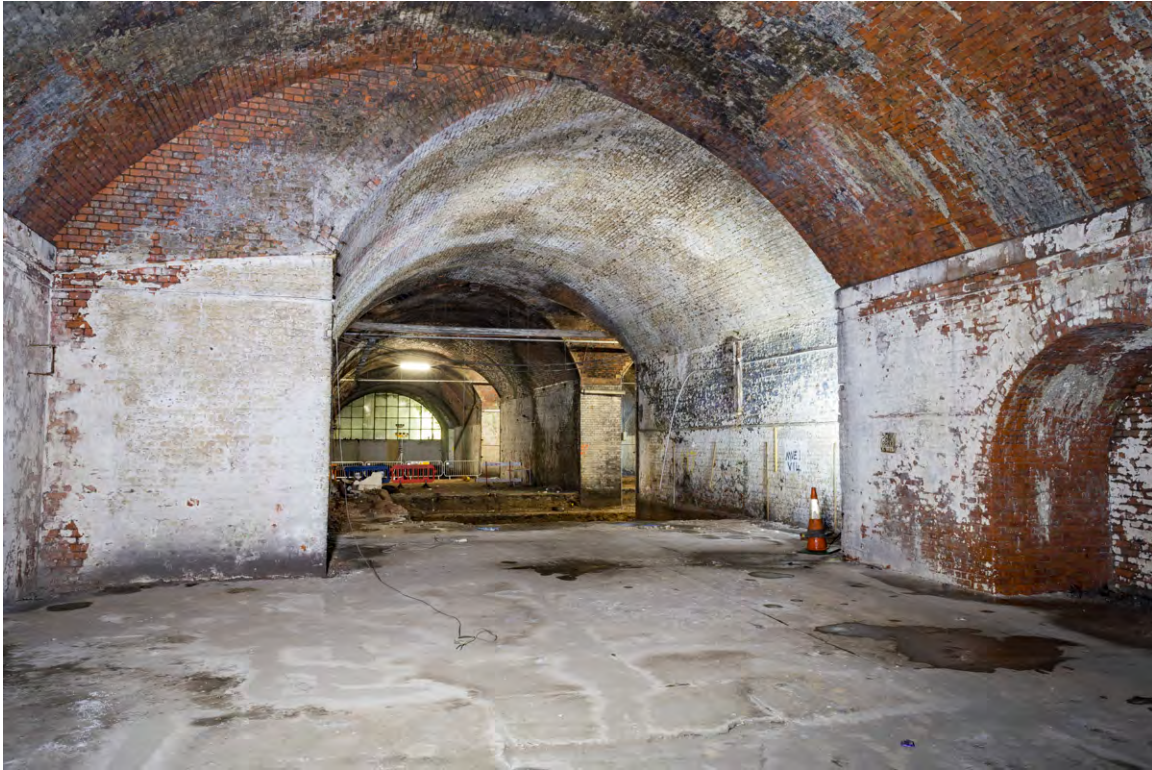
Plate 42 Vault 4A, looking south to vaults 4 and 3, showing dis-alignment
