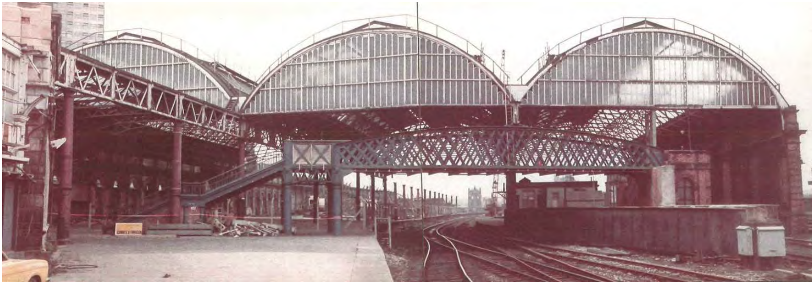
Plate 11: Rebuilt trussed roof over platforms 3, 4 and 5, c.1981, looking west ©Salford Local History Library
