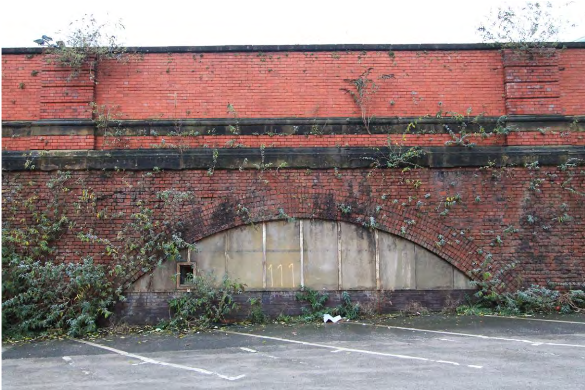
Plate 26 Detail of vault 11B arch and parapet wall to podium level, looking north
