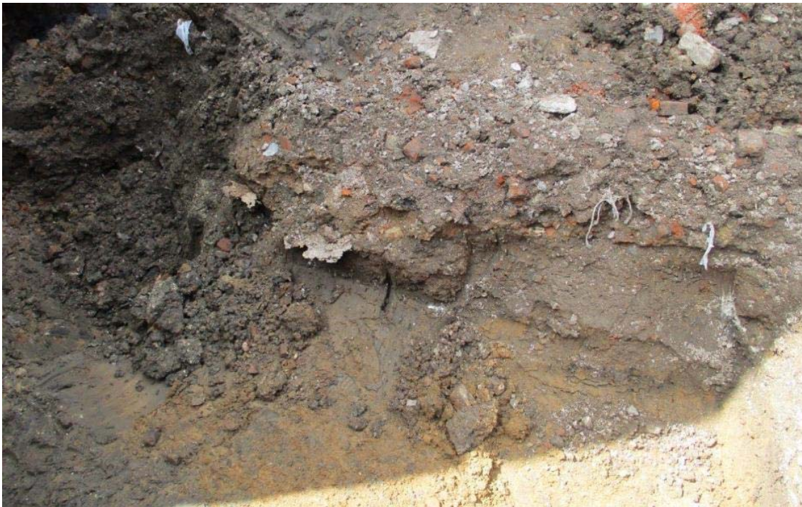
Plate 4 – West section of new foundation excavation in progress. View to south-west. No scale. Photo courtesy of Ingrid Peckham.
