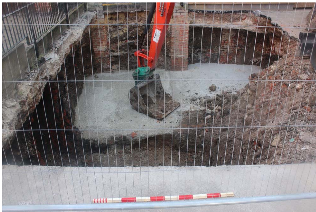
Plate 1 – Mass concrete poured against existing foundation piers. View to south. Scale 1m.
