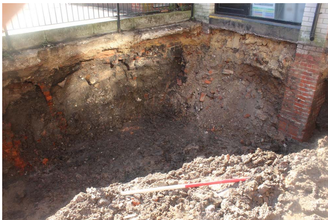
Plate 2 – East and south sections of new foundation excavations. View to south-east Scale 1m.
