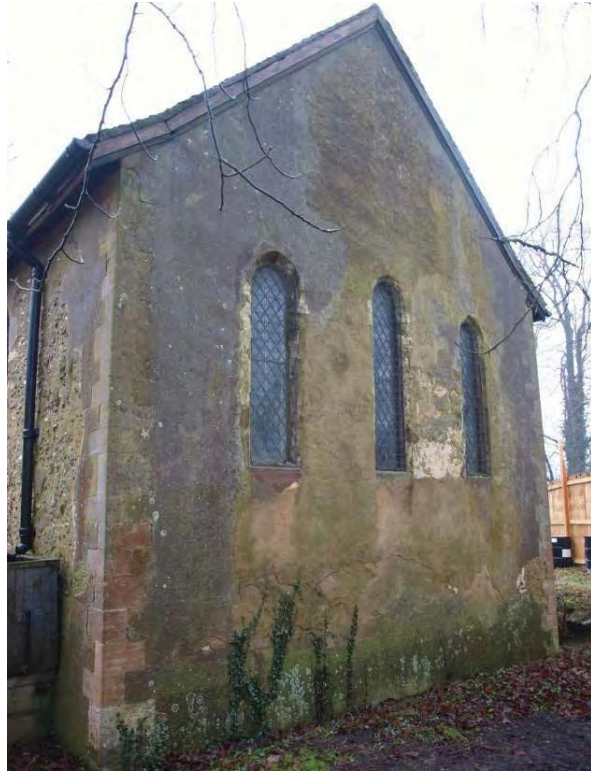
Plate 9. East elevation of the chancel with three original lancet windows but newer barge boards, stone quoins and cement render.
