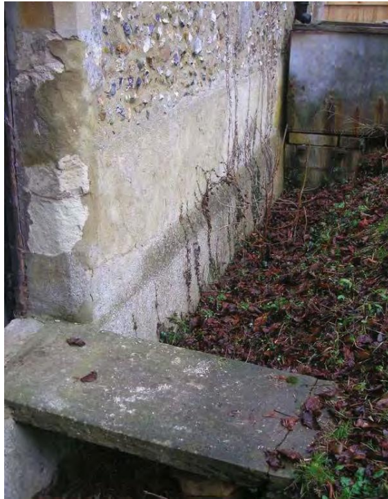
Plate 13. South elevation of the chancel showing the cement render, stone slab to the priest door and plinth.
