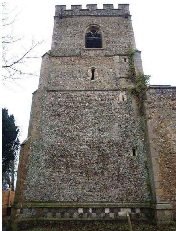
Plate 20. South elevation of the tower, with small windows on right illuminating spiral staircase.
