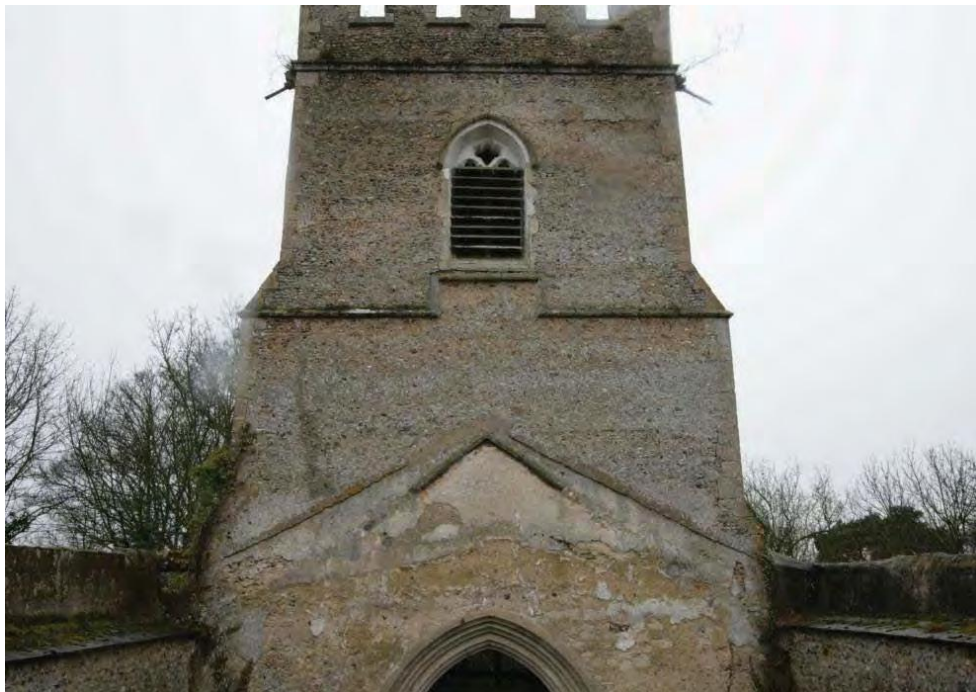
Plate 26. East elevation of the tower showing previous nave rooflines and concrete and slate capping of nave walls.
