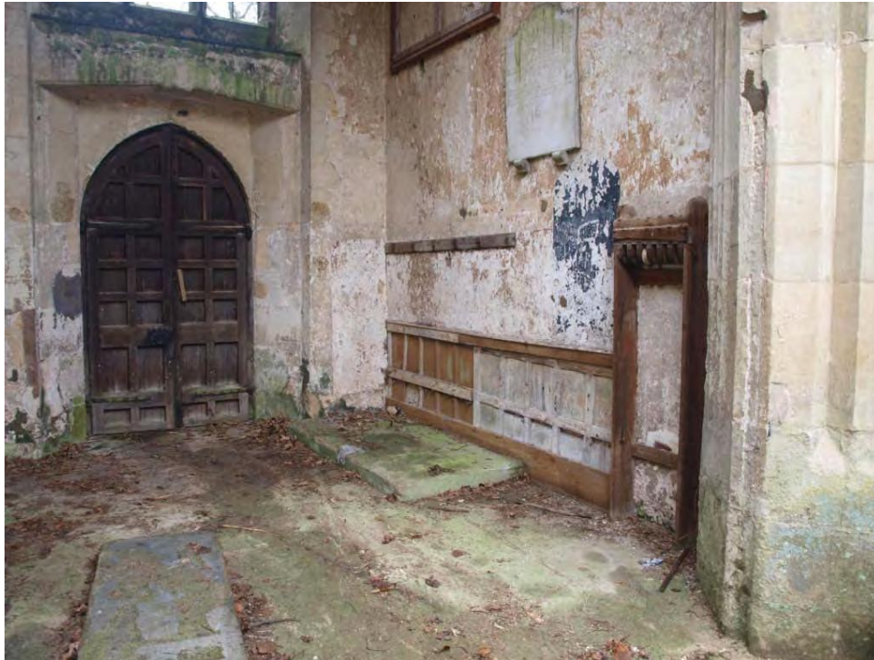
Plate 41. Base of the tower showing doors in west elevation, timber panelling and fittings for bell ropes. Also noticeable is a vertical groove cut into the centre of the tower/nave arch to house a timber screen.
