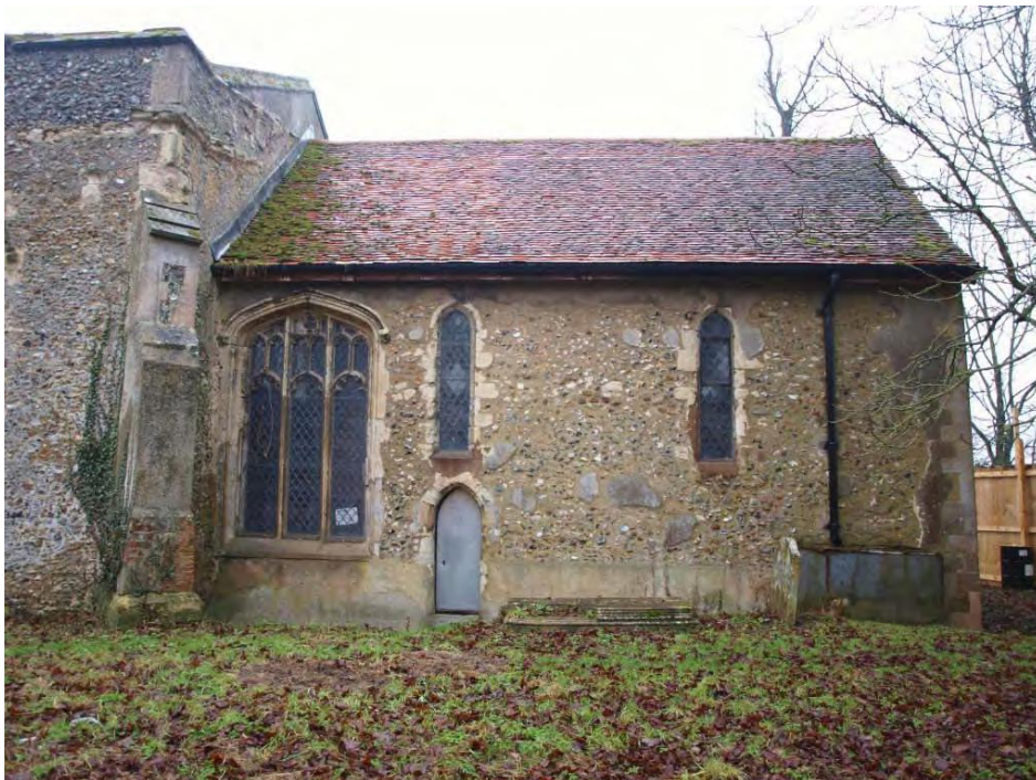
Plate 12. South elevation of the chancel with two original lancet windows and doorway and a large inserted fifteenth century window.
