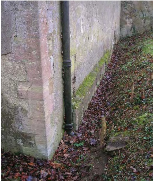
Plate 11. Detail of the north elevation of the chancel with replacement quoins and moss growing on the cement rendered upper edge of a shorter plinth or possible former wall on a slightly different alignment.
