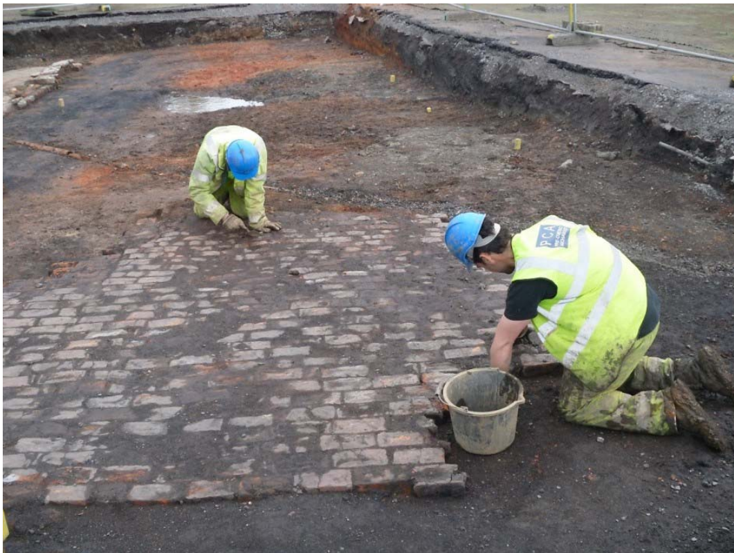
Plate 8. Area A, working shot Phase 4b brick surface [1064] (northern part), looking east
