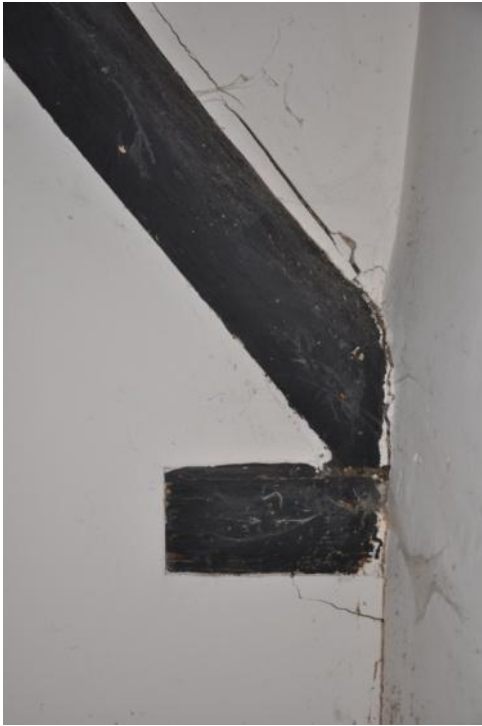
21. Sawn off tie beam in bedroom 2.
