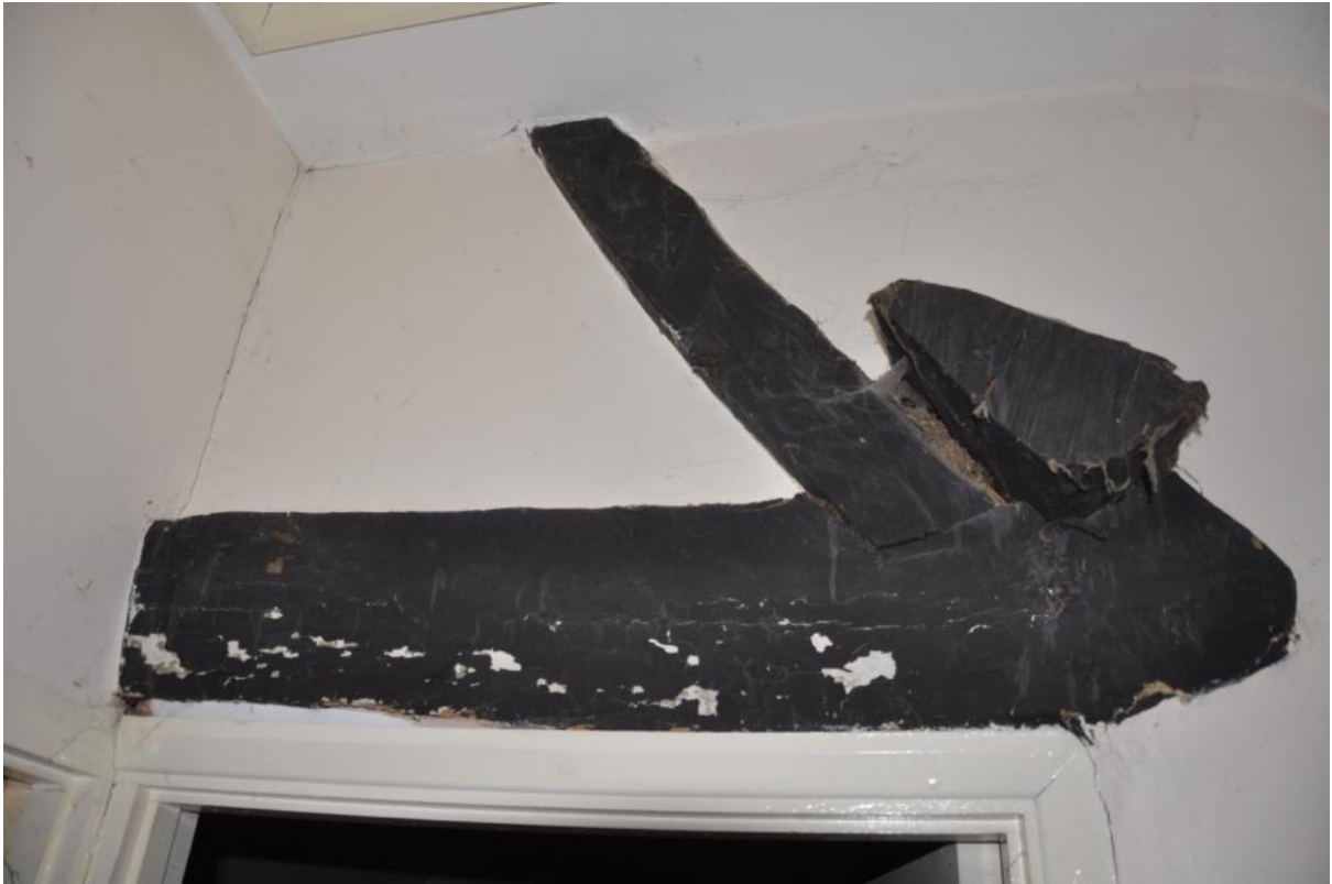
19. Detail of truss showing principal rafter and collar and sawn off purlin.
