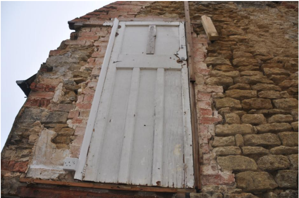
6. First floor doorway showing brick patching and later brick and stone southern wall.
