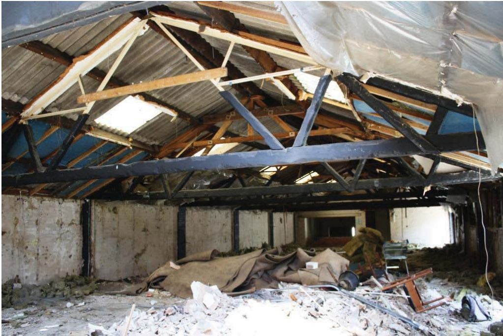
Plate 15. Interior of Link Building (Building 3), looking north-west, showing lower half of steel roof truss clad in timber below a now removed ceiling.
