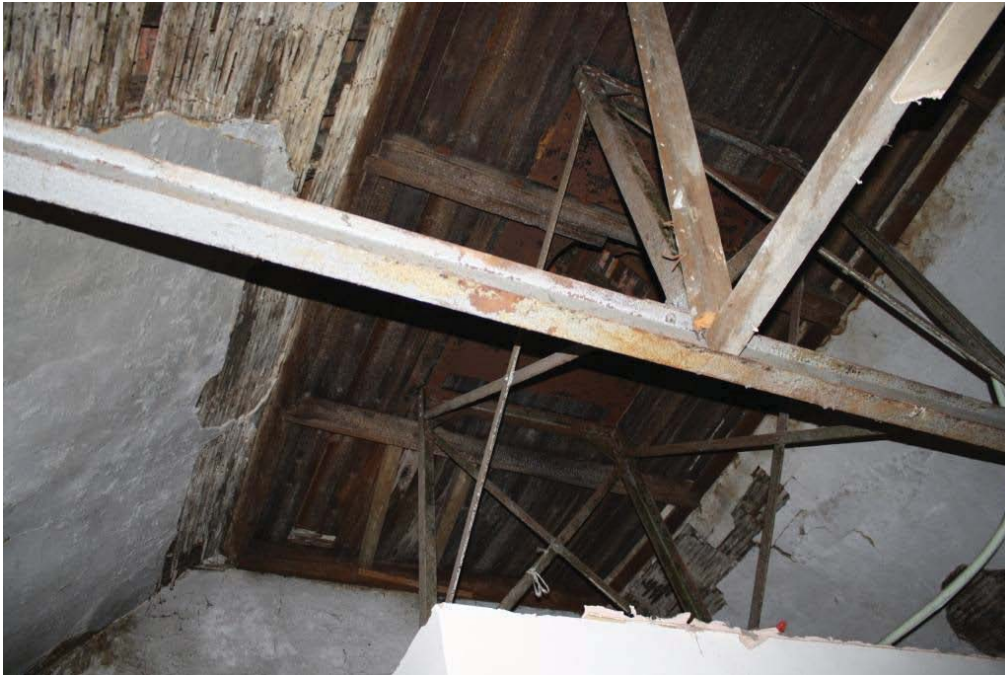
Plate 13. Steel frame and ventilation system in apex of roof in the southern part of Building 2, looking north-east.
