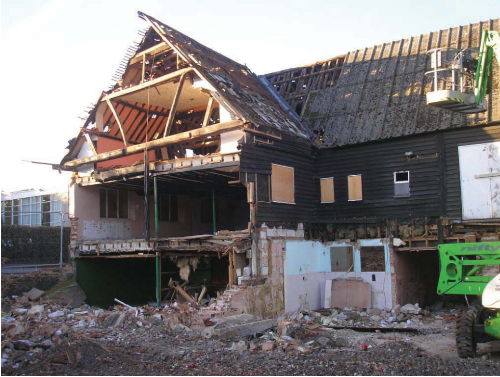
Plate 36. East-west block (left) and north-south block (right) of Maltings Building 5 during demolition of the east-west block, looking south-west.
