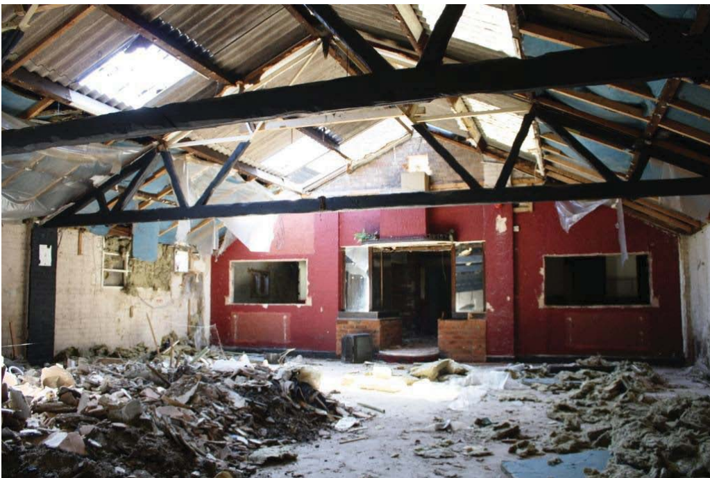
Plate 16. South end of the interior of Link Building (Building 3) with access into Building 6, looking south-east.
