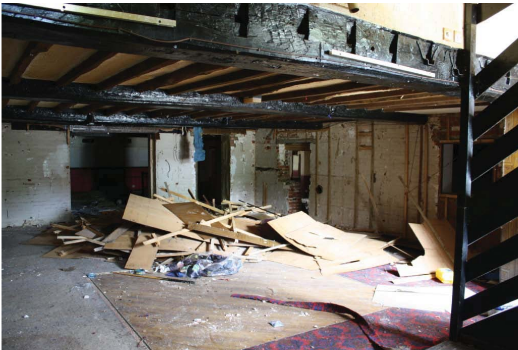
Plate 41. South end of ground floor of Building 7, looking north-east. Inserted steps on the right provide a fire exit to Park Street.
