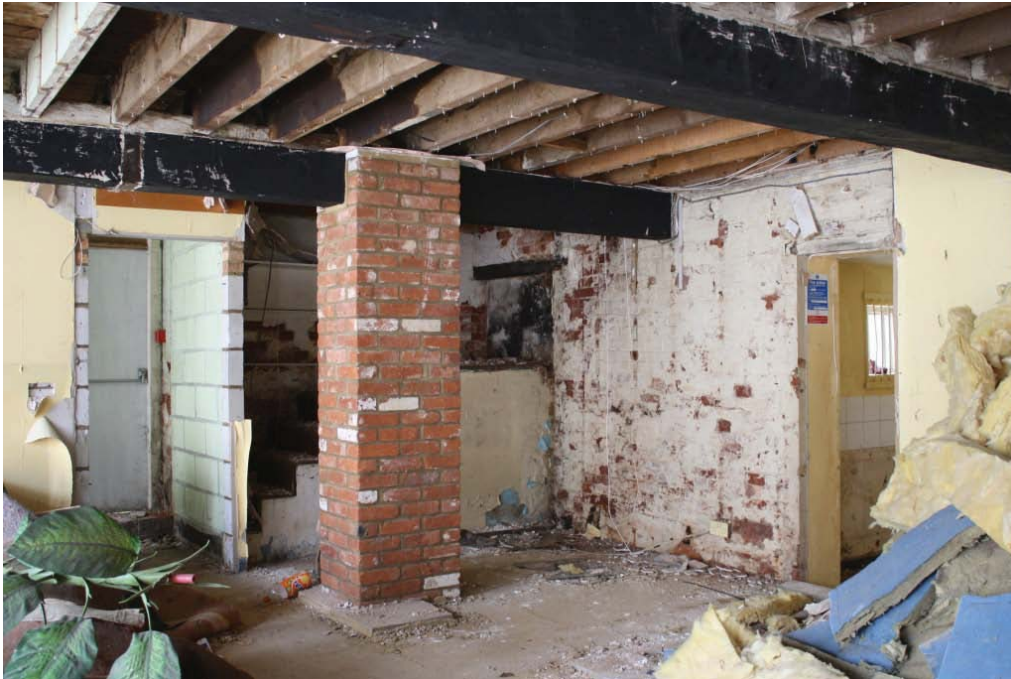
Plate 5. South-east corner of no. 31a Hitchin Street shop (Building 1), showing inserted brick pillar and blockwork partitions, with a blocked door and truncated flight of steps to the first floor in the corner of the room.
