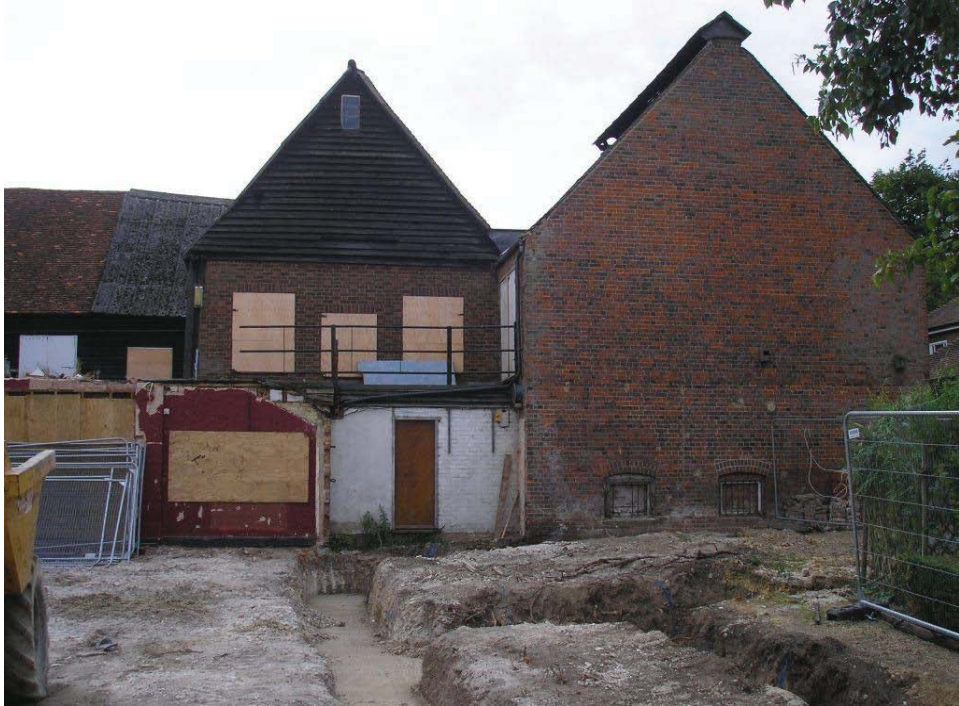
Plate 23. North elevation of Building 5 (left) and brick gable of later Building 7 (right), looking south.
