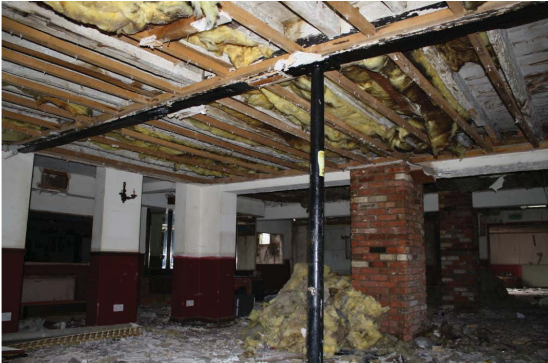
Plate 27. Ground floor of the north end of the north-south block of Maltings Building 5 (snooker club bar), showing iron post, joists and floorboards, looking north-east into Building 6.
