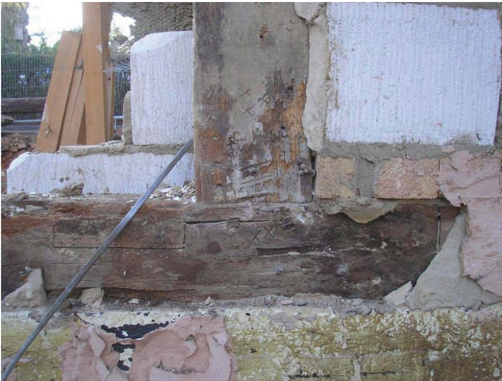
Plate 22. Carpenters marks 'XX', visible on each side of a pegged mortise and tenon joint, connecting a vertical post with the cill beam set on a low brick wall. This was exposed during demolition of the north elevation of the central section of Building 5, looking south (see Plate 36 for location).
