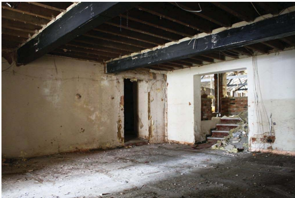
Plate 6. Building 1 extension at ground floor level showing narrow doorway into Building 2 and wider doorway and steps up into Building 3, looking south-east.
