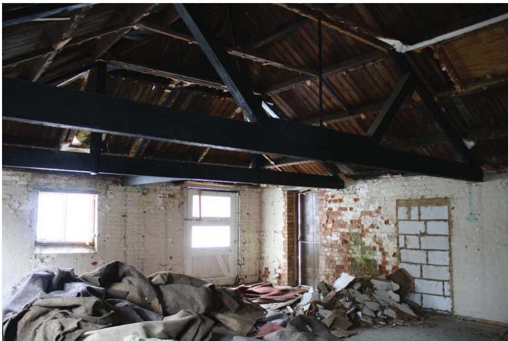
Plate 10. South-east corner of the main part of no. 31a Hitchin Street (Building 1) at first floor level, showing from right to left a blocked door, an inserted door and an original loading door.
