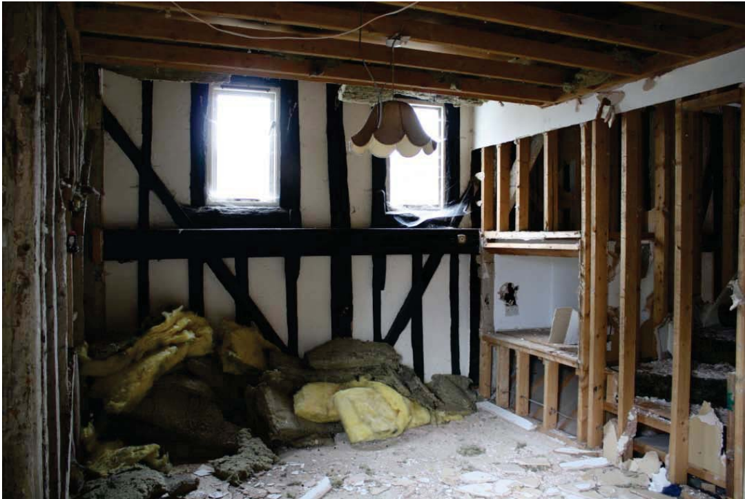
Plate 29. First floor living accommodation in the east wing of Maltings Building 5 looking east, showing modern inserted timber stud wall (right).
