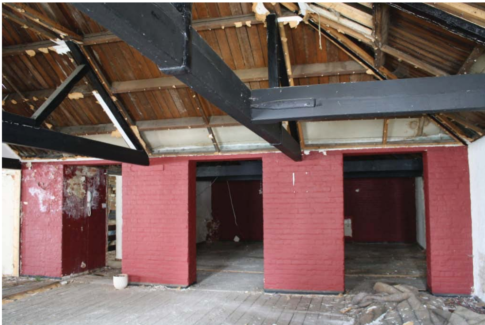
Plate 8. West end of the main part of no. 31a Hitchin Street (Building 1) at first floor level, showing iron reinforcing brackets on timber trusses and doorways to the extension, looking south.
