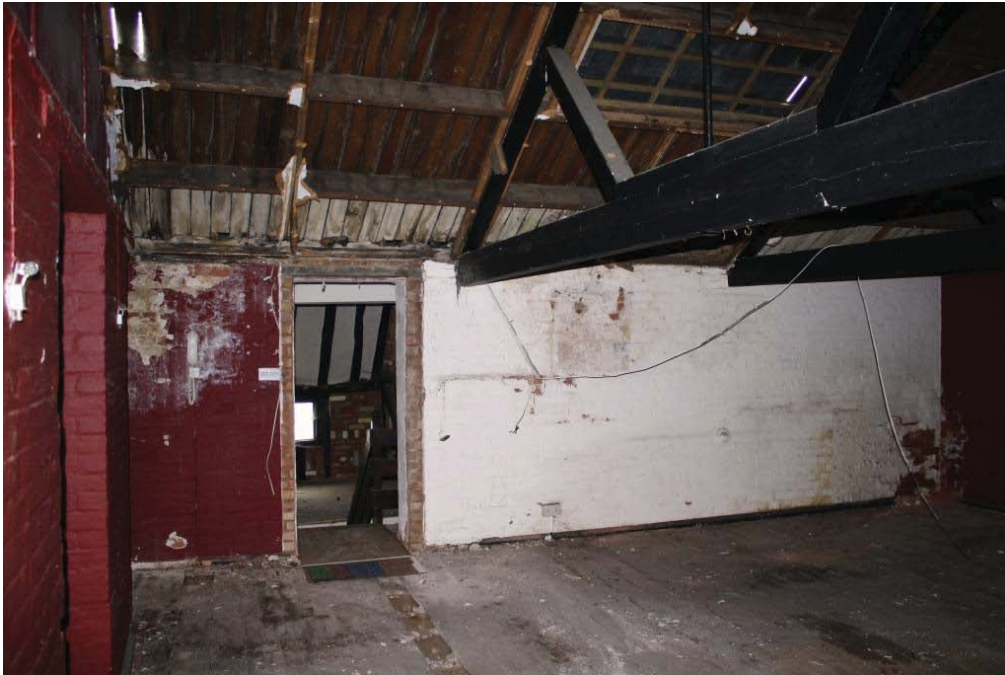
Plate 7. East wall of Building 1 extension at first floor level looking east, showing blocked skylight and doorway to stairs.
