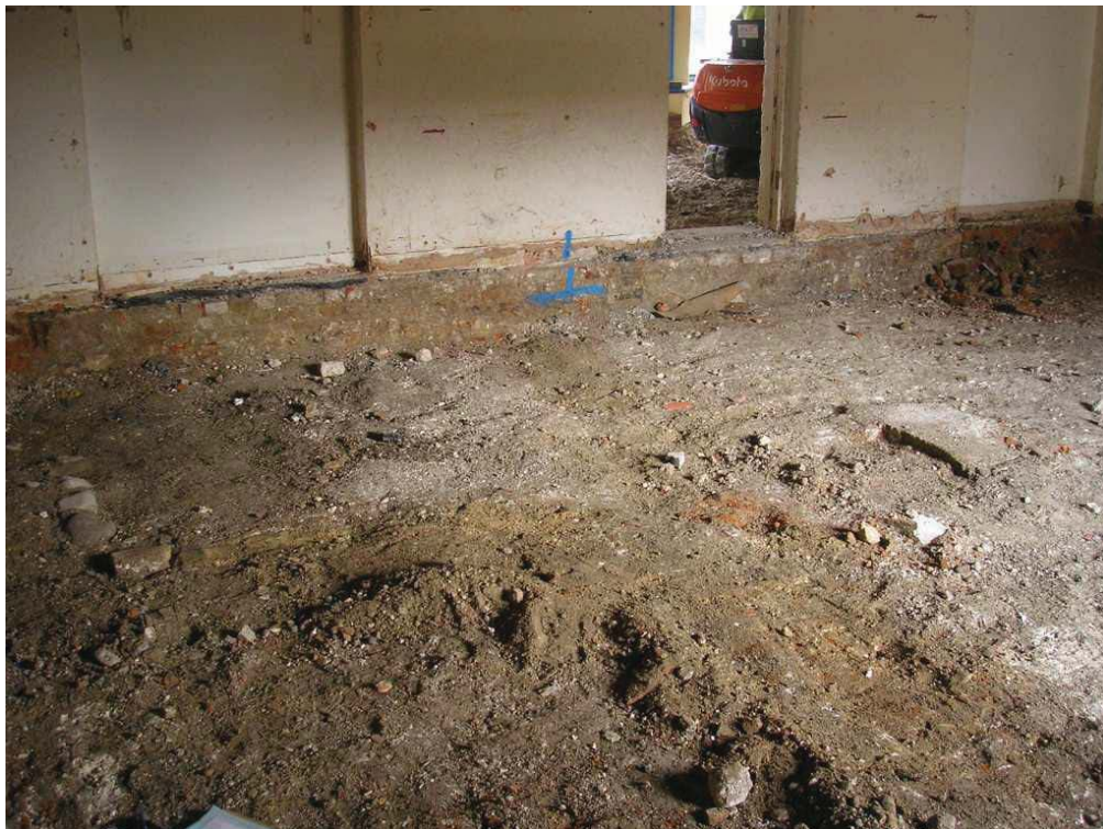
Plate 47. Trench 2 within the extension of Building 1, looking north-east, showing brick features and areas of excavated chalk.
