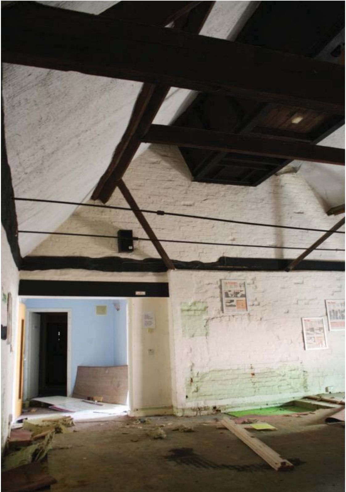
Plate 43. North end of first floor of Building 7, looking south toward dividing brick wall.
