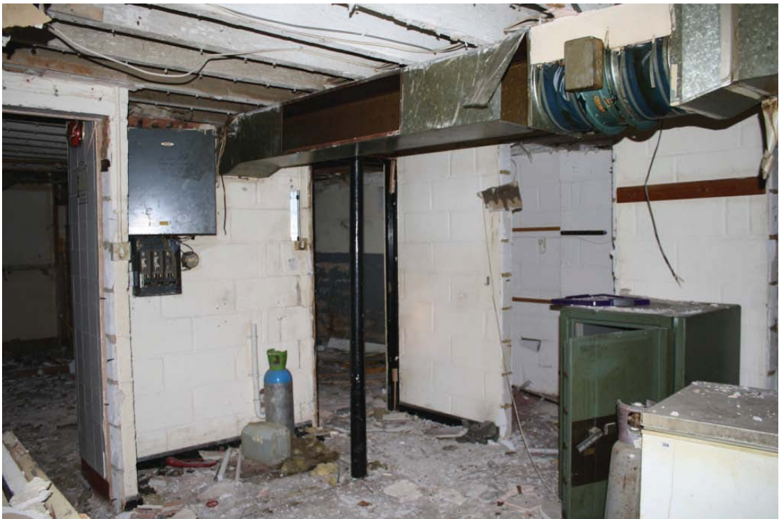
Plate 28. Cold store, on ground floor at south end of the north-south block of Maltings Building 5, looking north-east with doorway into kitchen on left.
