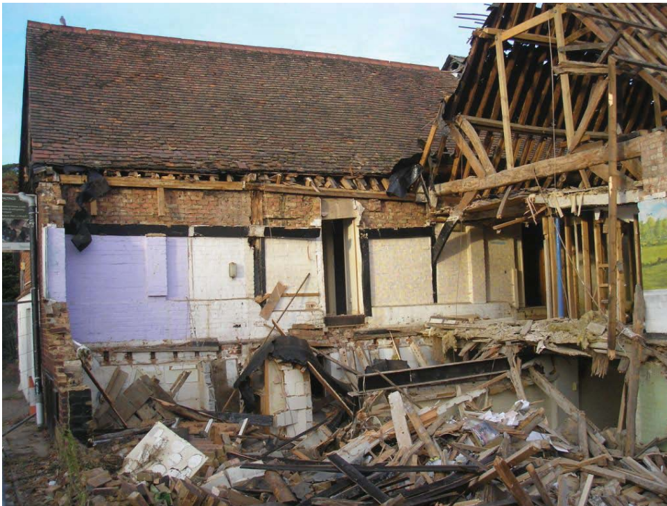
Plate 24. North-south block of Maltings Building 5, largely demolished, showing how the brick walls of the later Building 7 infilled between the timber posts of Building 5, looking north-west with Park Street to the left.
