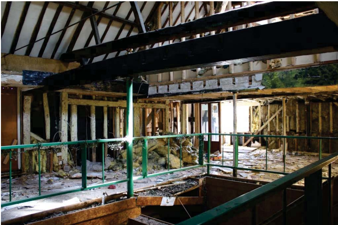
Plate 30. First floor of east-west block of Maltings Building 5, looking north-east, showing timber-framing, inserted stairs down to ground floor in foreground and missing floor joists above.
