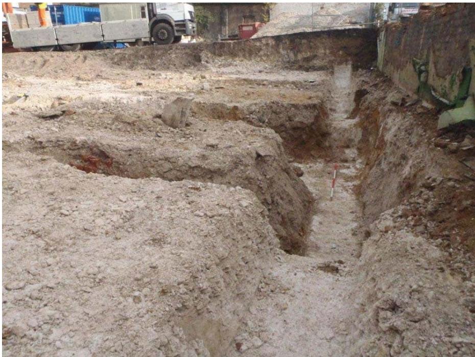
Plate 49. View looking north-east of the excavated foundations of Trench 5, with on the right, the retaining wall on Park Street.
