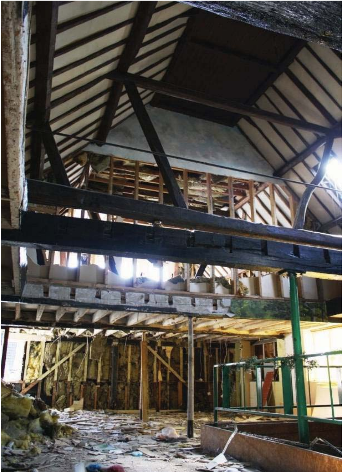
Plate 31. First and second floors of south-east corner of east-west block, Maltings Building 5, looking east.
