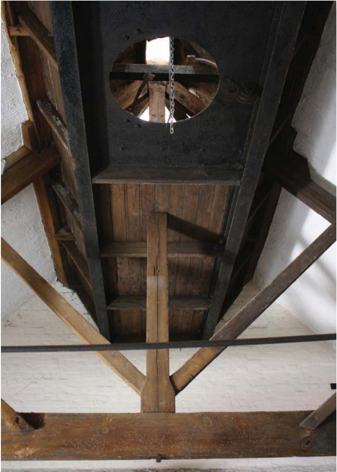
Plate 45. Roof truss and ventilation at north end of first floor of Building 7, looking north.
