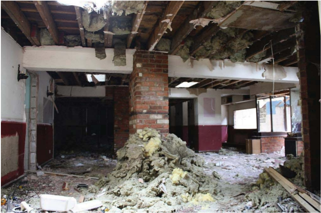
Plate 38. View of Building 6 interior, looking west, with access into the snooker hall of Link Building 3 on the right and snooker club toilets on the left.
