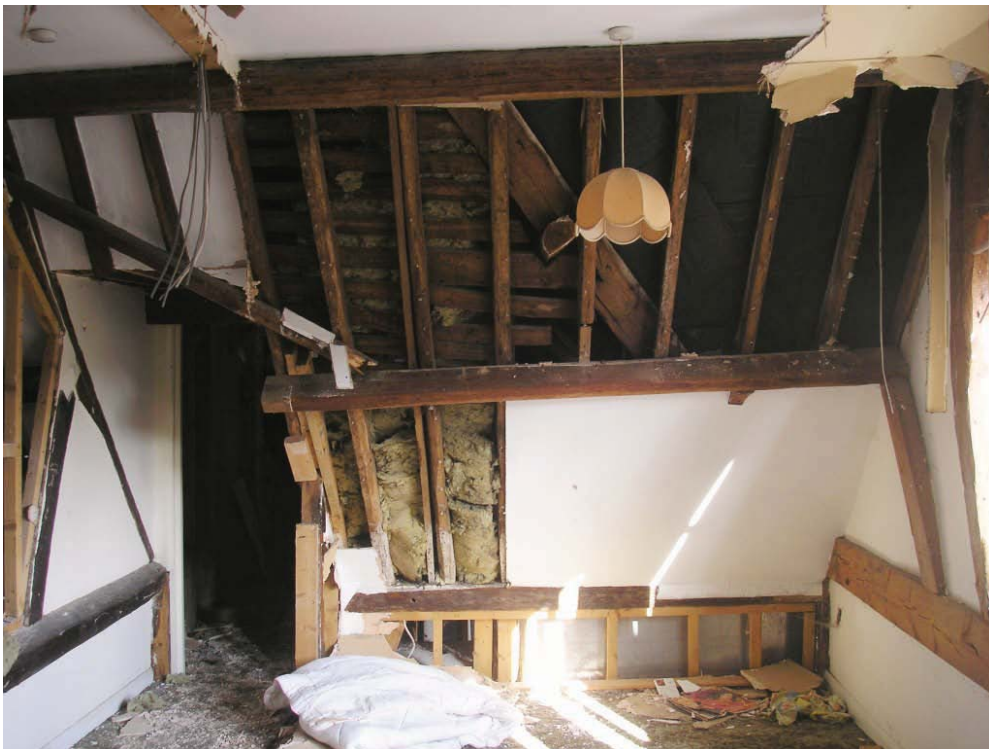
Plate 33. Inserted doorway at second floor level, between east-west block and east wing in Malting Building 5, looking north. The purlin has been severed and the roof line of the added east wing is visible through the rafters.
