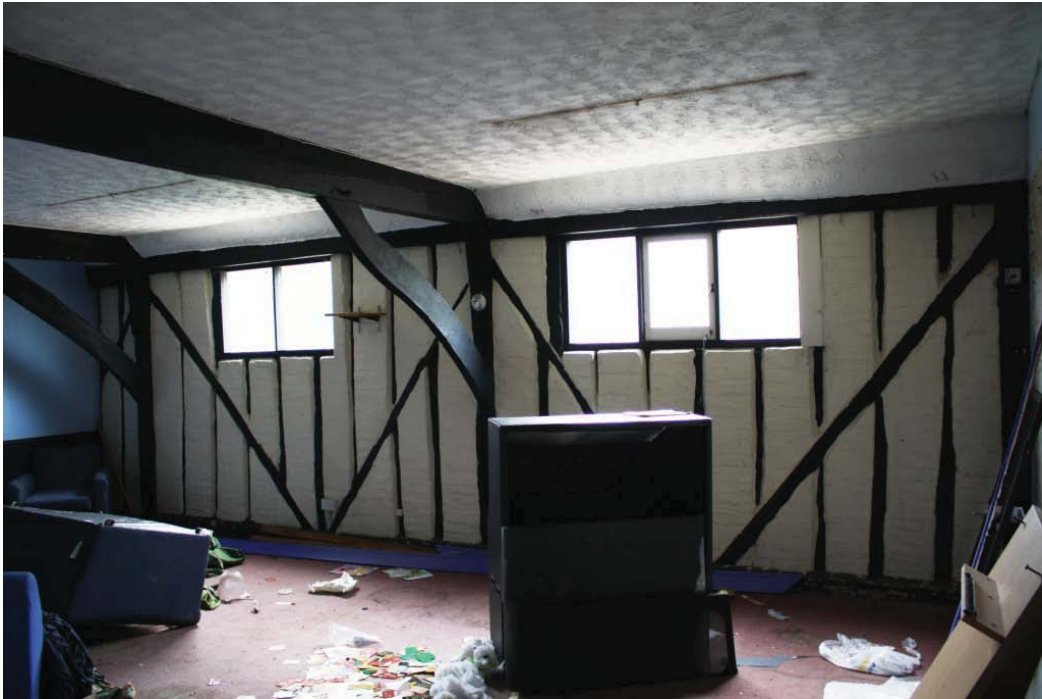
Plate 42. Central room on first floor of Building 7 (spa TV room), looking west.
