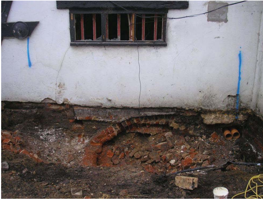
Plate 48. Trench 4 excavated along the east elevation of Building 2, looking west, showing lower section of brickwork probably infilling a previous doorway the same width as the window. Visible below this is a partially demolished red brick segmental arch [19].
