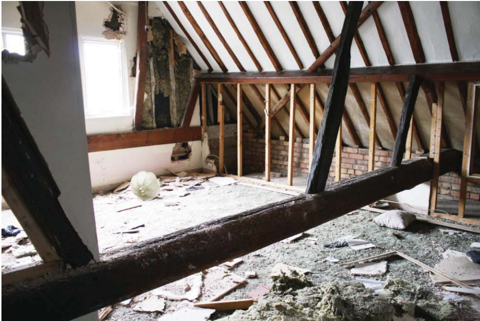
Plate 34. Second floor bedroom at east end of east-west block of Maltings Building 5, looking south-east, showing tie-beam, braces and modern brick wall. In the far corner, below the tie-beam, the gable wall retains original boarding down to the floorboards.
