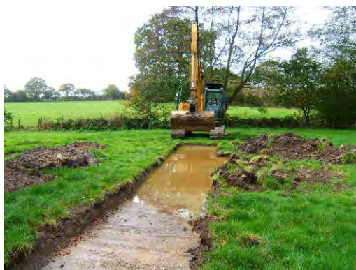
Plate 25: Trench 148b: Flooding at south end of trench. View looking south.
