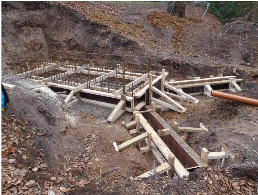
Plate 8: View looking south of main spillway area to west of rear access road showing culvert under construction.
