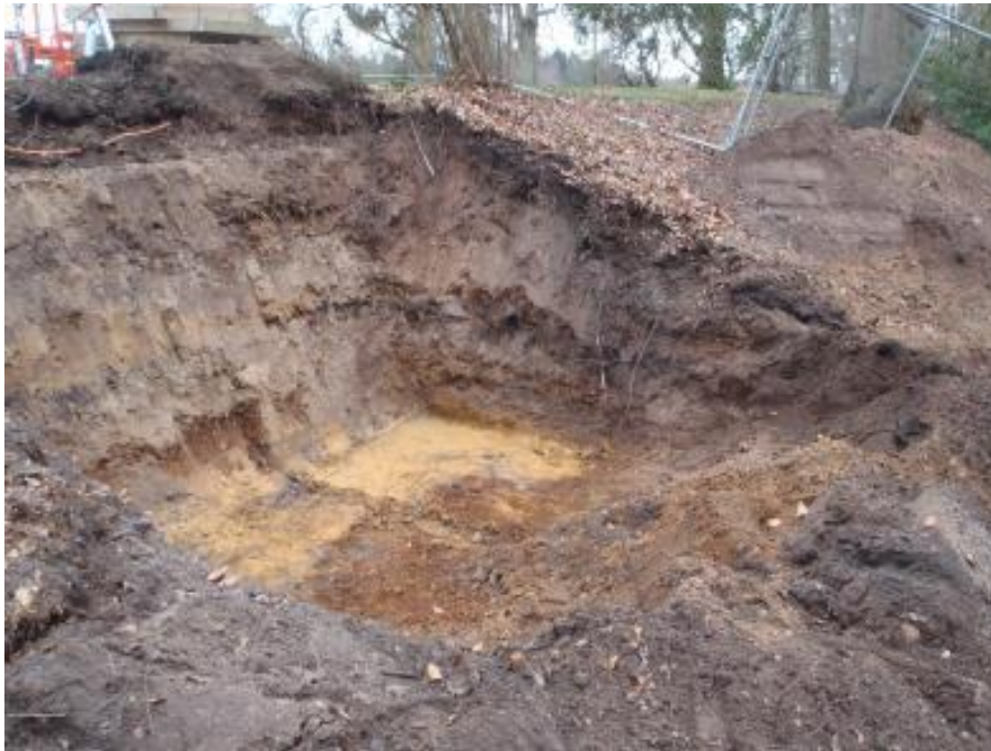
Plate 7: View looking south of main spillway area to west of rear access road
