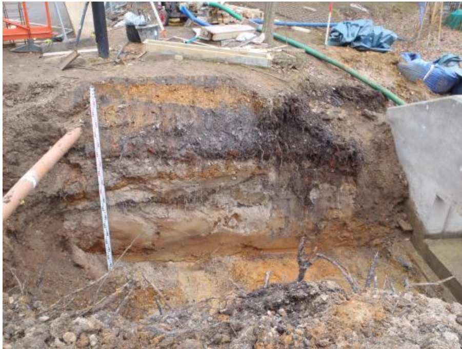
Plate 9: View looking north of main spillway area on eastern side of rear access road showing section through lake embankment
