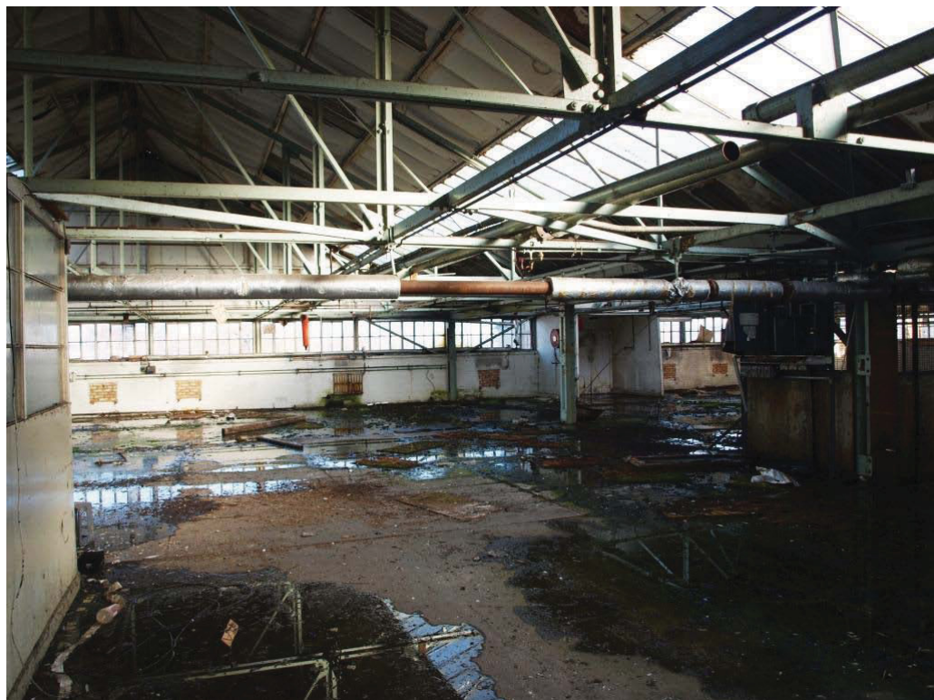
Plate 20. Open plan mezzanine office space in northwest corner of Old Bronze Foundry (5).
