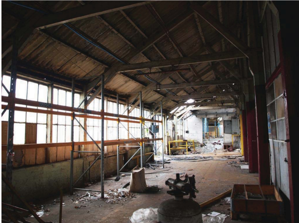
Plate 77. Timber framed corridor space on the east side of Building 29, looking south.
