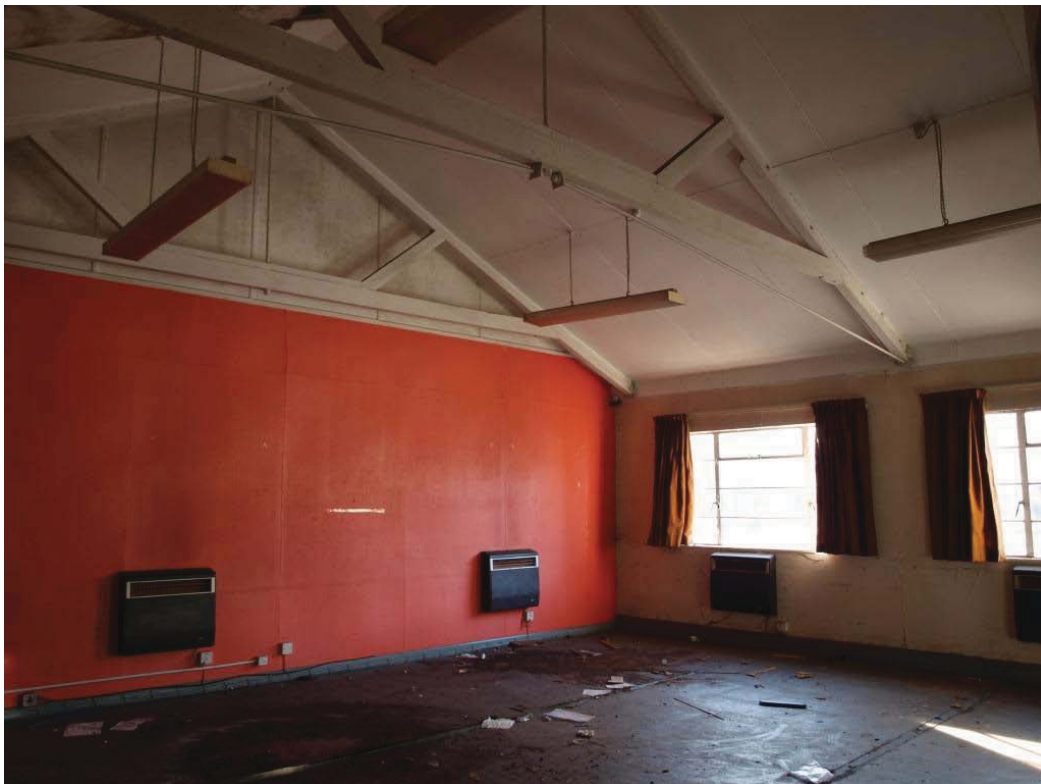
Plate 40. Large interior space at the east end of the Works Pavilion, showing the timber roof truss construction with metal tie rods for additional strength.
