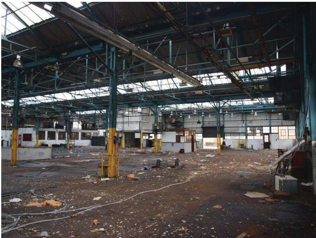
Plate 32. East side of the interior of the Union Machine and Assembly Building (7).
