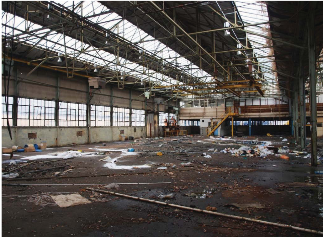
Plate 19. West side of Old Bronze Foundry (5) looking north, with mezzanine open plan office at the north end.
