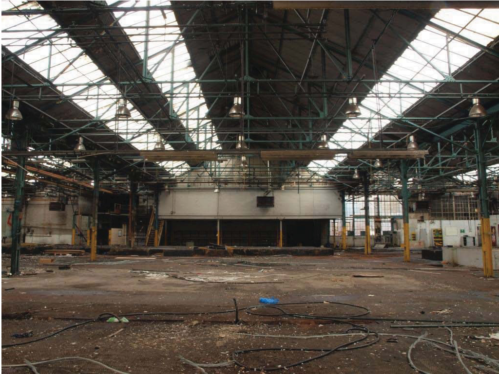
Plate 33. North side of the third bay from the east showing mezzanine (Building 7).
