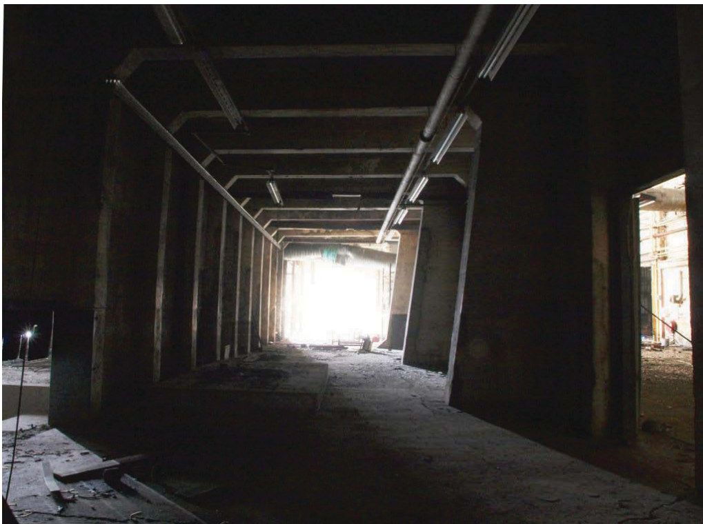
Plate 46. Interior space on west side of Malleable Core Shop (14), showing concrete casing of steel buttresses to main building on right.
