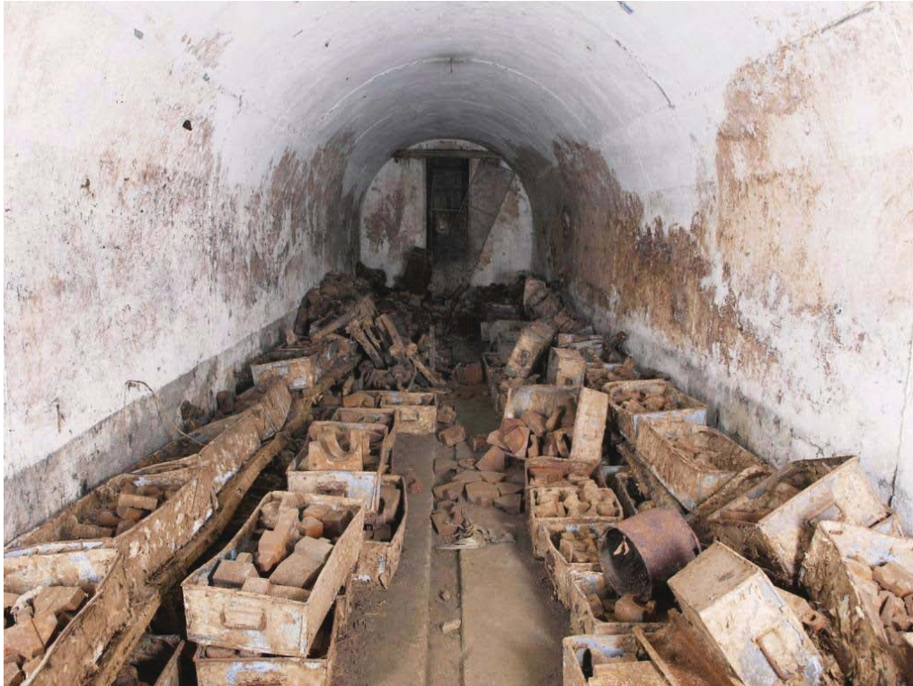
Plate 53. Air Raid Shelter 4 looking north, containing stored metal components on collapsed original wooden benches. At the far end is an emergency escape ladder.
