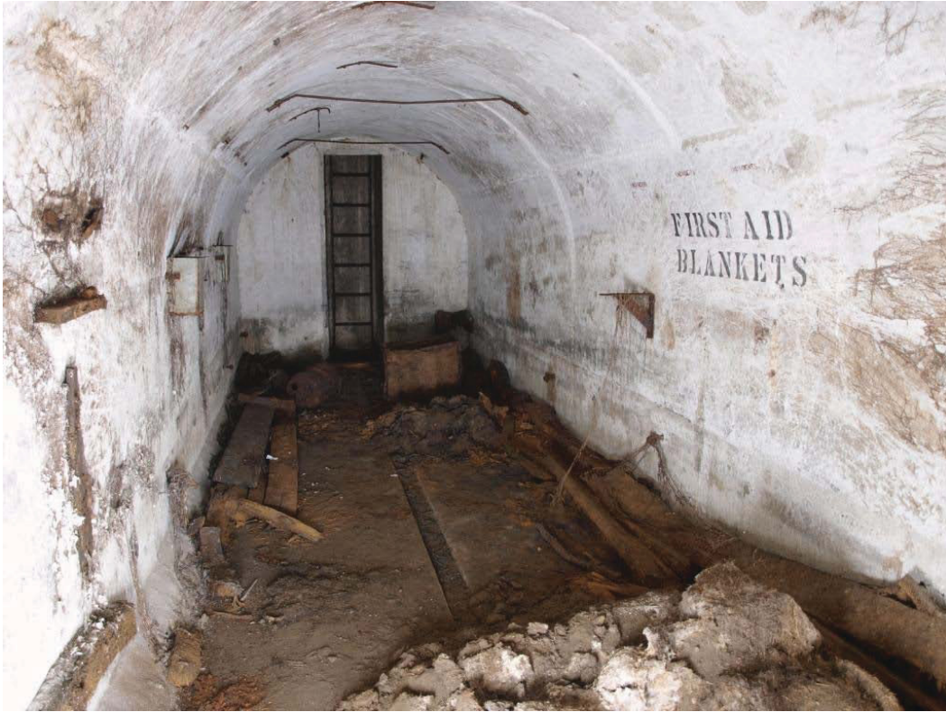
Plate 55. Interior of Air Raid Shelter 2, looking north, showing remains of original timber benches and signage.
