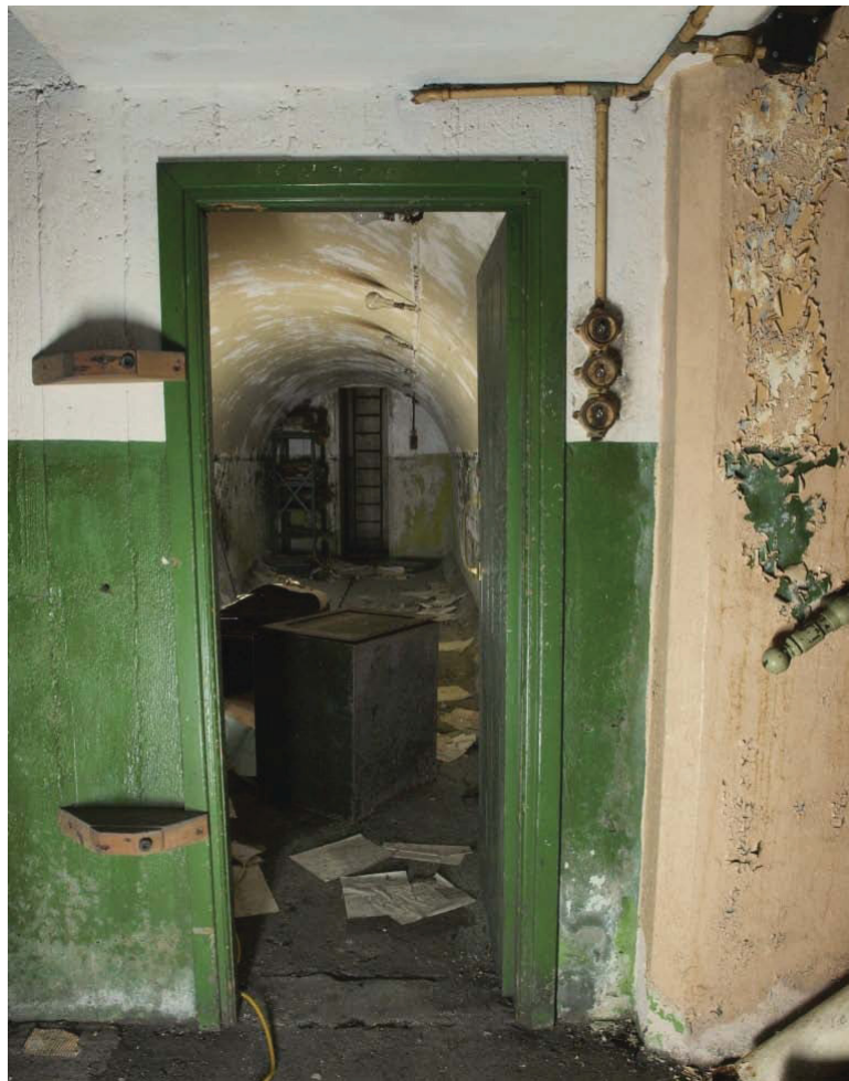
Plate 74. Air Raid Shelter 1 beneath Building 27, looking west. On the right are the concrete entrance steps and behind the camera is a same sized second chamber.
