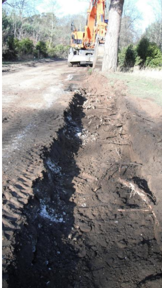
Plate 42: Widening eastern side of track. Note root activity
