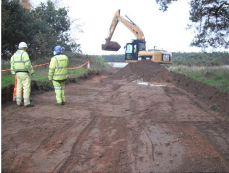
Plate 13: Reduction of eastern end of T68. Excavation did not penetrate below subsoil
