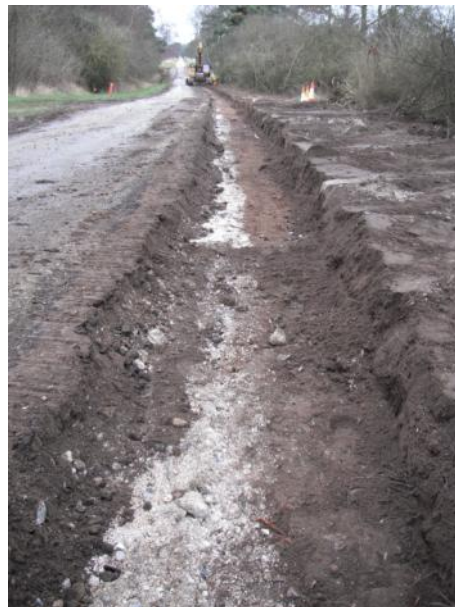
Plate 51: Ground disturbance by existing track. View West
