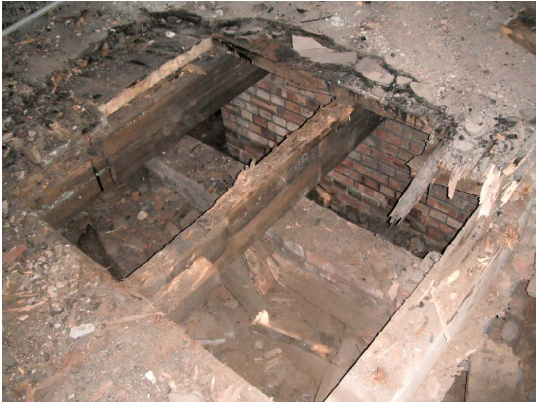
Plate 4. West side of Trench 2, showing partially dismantled timber platform supported on timber joists and brick walls, looking north-west.
