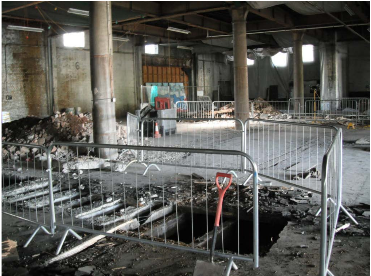
Plate 1. Trenches 1 and 2 (in the distance and in the foreground, respectively) in the Midland Goods Shed at ground floor level, looking north-west.
