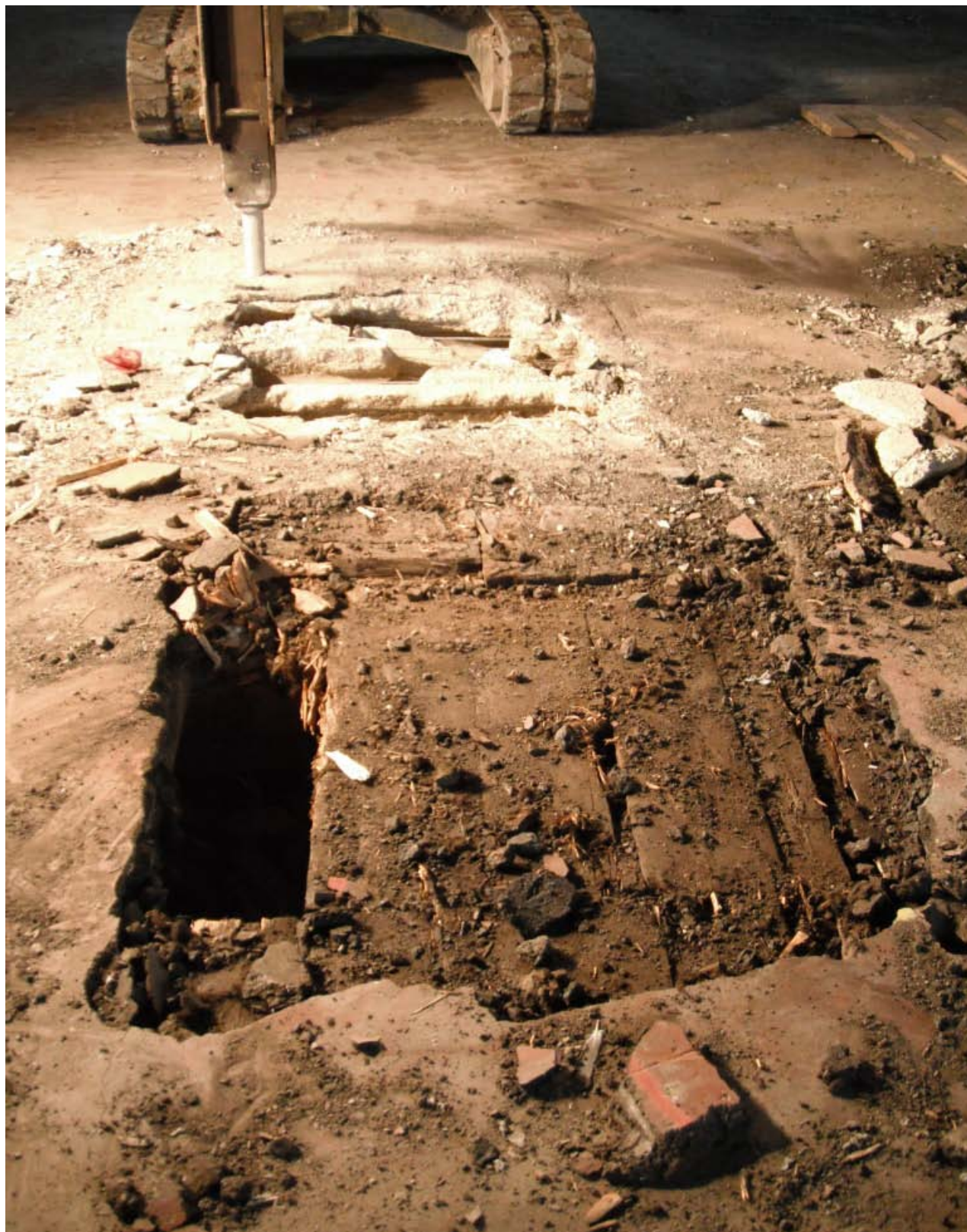
Plate 2. Asphalt being removed at the east end of Trench 1, exposing timber platform with reinforced concrete beams over previous location of railway track, looking west.
