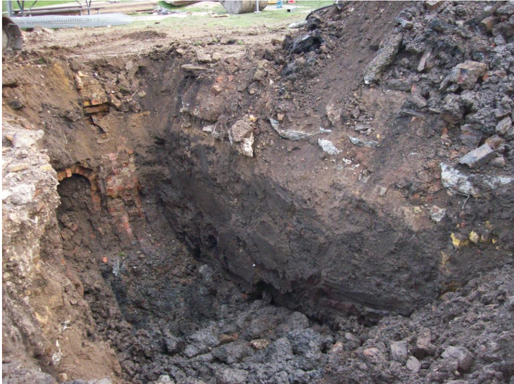
Figure 5: Enabling trench for breaking out modern storm drain Note the peat deposit evident in the base of the section
