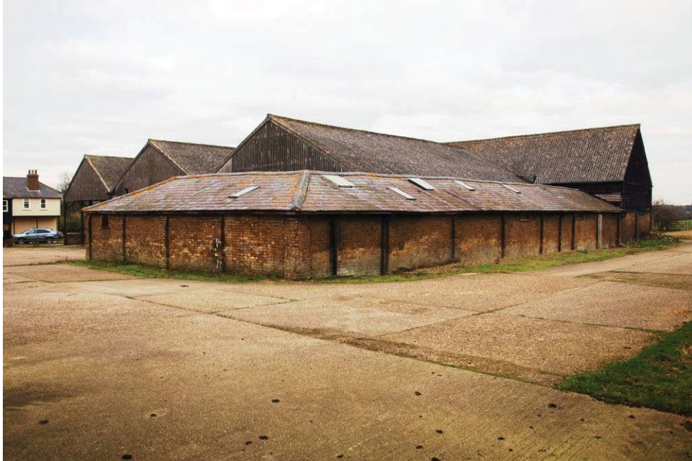
Plate 11. East and south elevations of Building 2, with east gable end of Building 1 on the right and the three south gables of Building 4.
