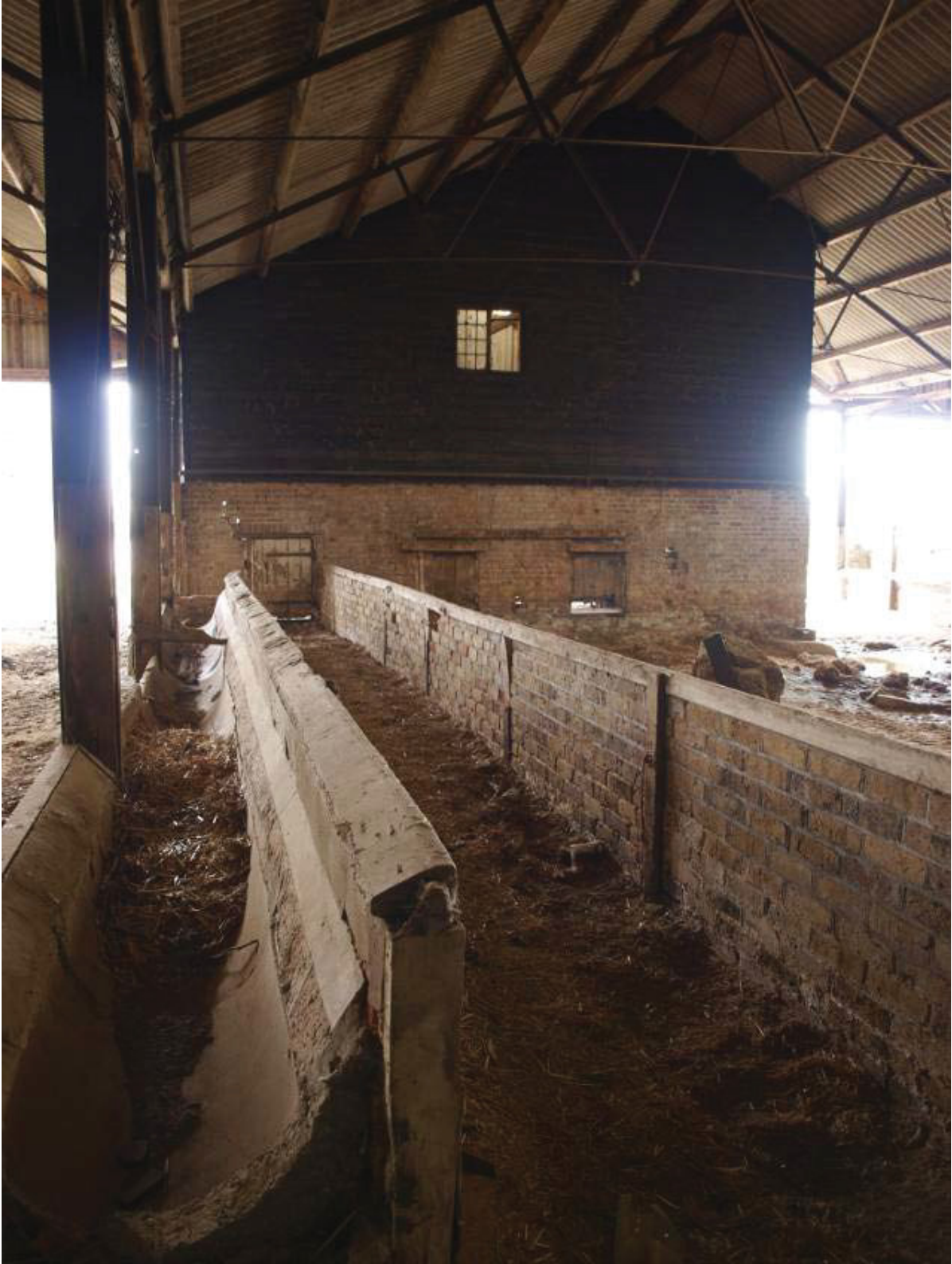
Plate 22. North elevation of Building 3 with brick and concrete feeding trough of Building 4 in the foreground.
