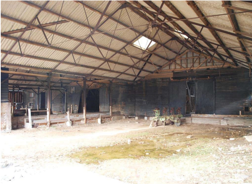
Plate 5. South elevation of Building 1 with three pairs of sliding doors view across the covered yard (Building 4).
