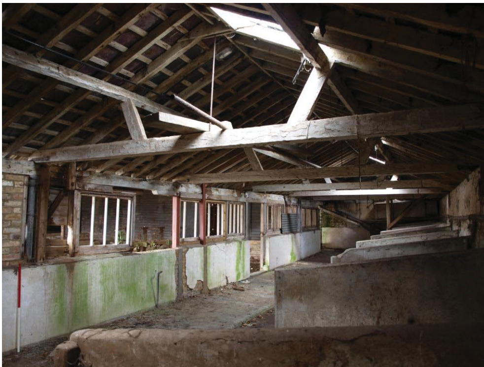
Plate 18. West side of Building 2, looking north-west, with cast iron column in wall on left.
