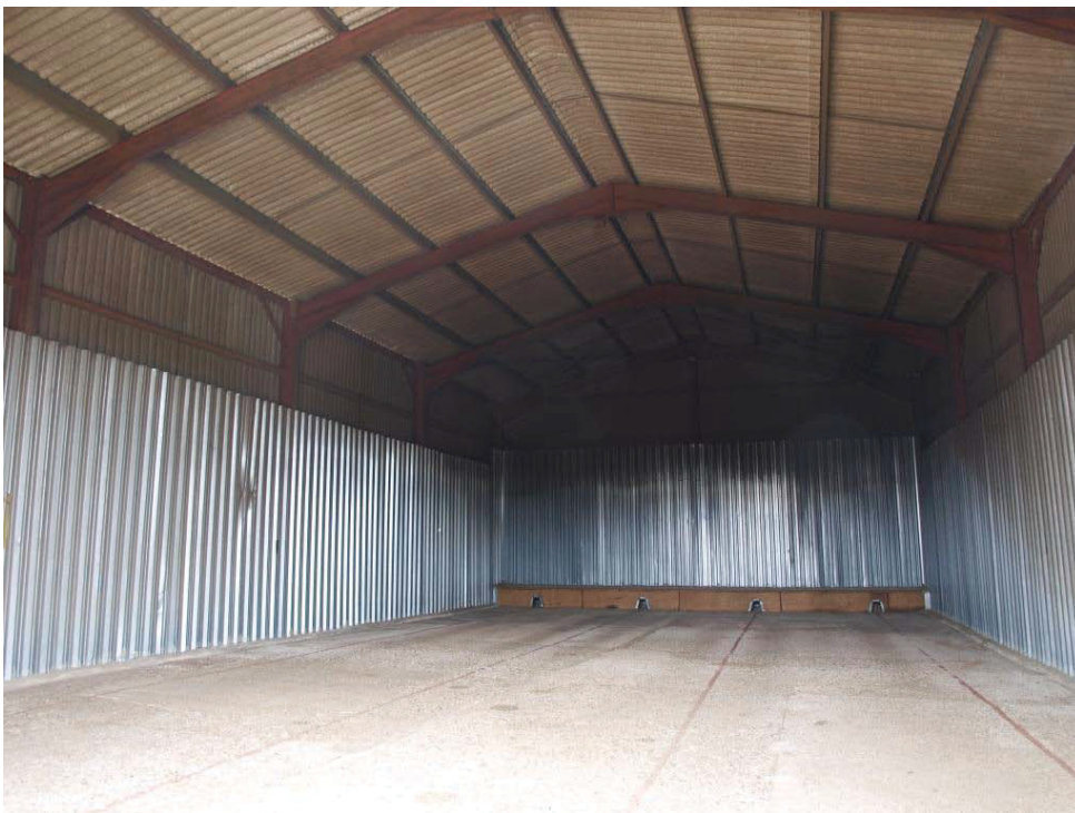
Plate 28. Interior of Building A with inserted air vents at the far end.
