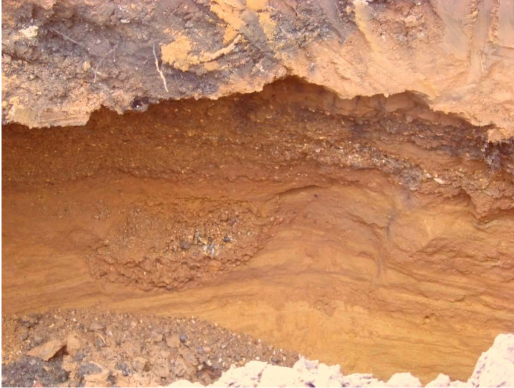
Figure G7: Trial Pit 2, Collapsed West Face (east facing)
