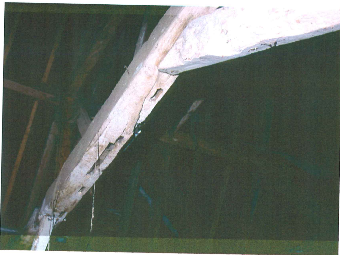
Plate 6: Slots in roof truss in timber barn
