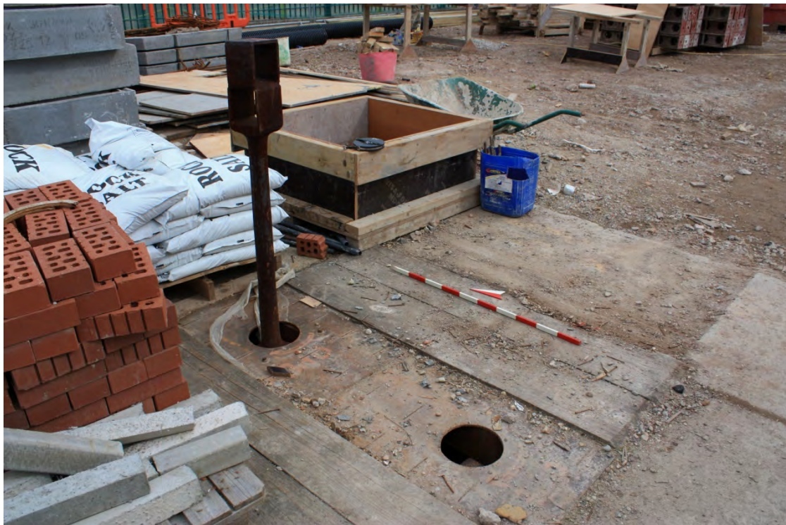
Plate 3. D308/17. Penstock valve P11 opening gear on the surface. NW corner Dry Dock No. 3. Scale 1.0m looking NE.
