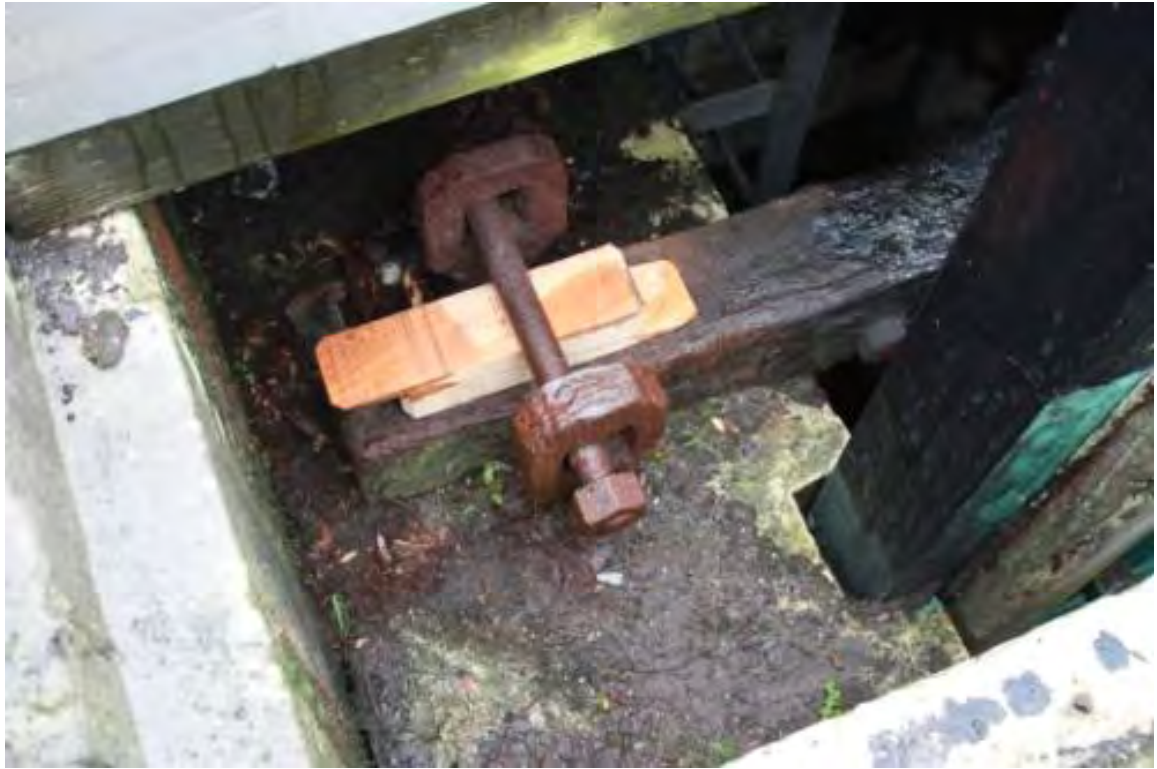
Plate 7. D.314/6. Operating Penstock valve located NW of HMS Victory. View looking south.
