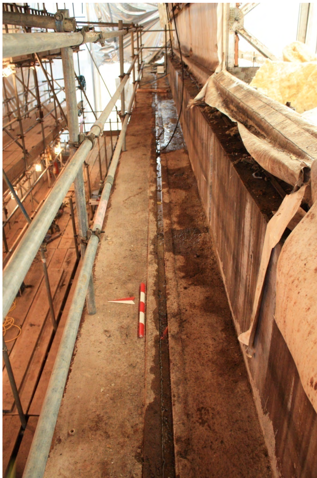
Plate 15. D304/19. 1920s inner facing dockside crane rail, inside the Weymes building, set into concrete along southern side of the dockside. Scale 0.5m looking E.
