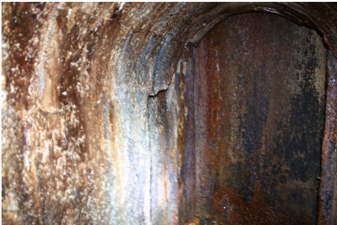
Plate 10. D305/61. 9.0m inside culvert [108]. On the right is the closed metal gate of Penstock valve P11 This isolates this section of the culvert from the rest of the system. Looking N.
