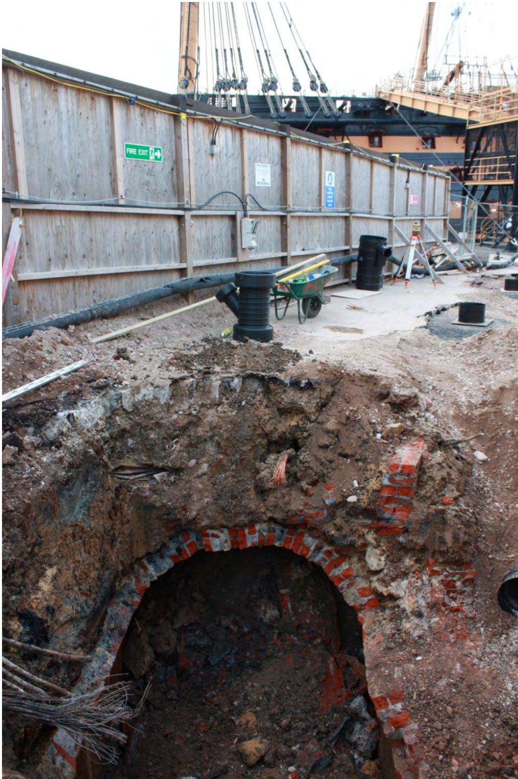
Plate 18. D 316/66. [142] Demolition shows sewer roof in section. Looking W back towards HMS Victory.
