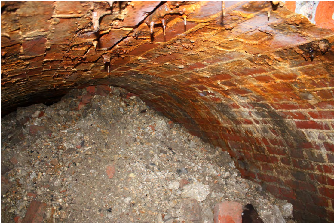
Plate 17. D 316/61. [142] Backfilled sewer at its western end. Note: material entered through hole in roof. Looking W.
