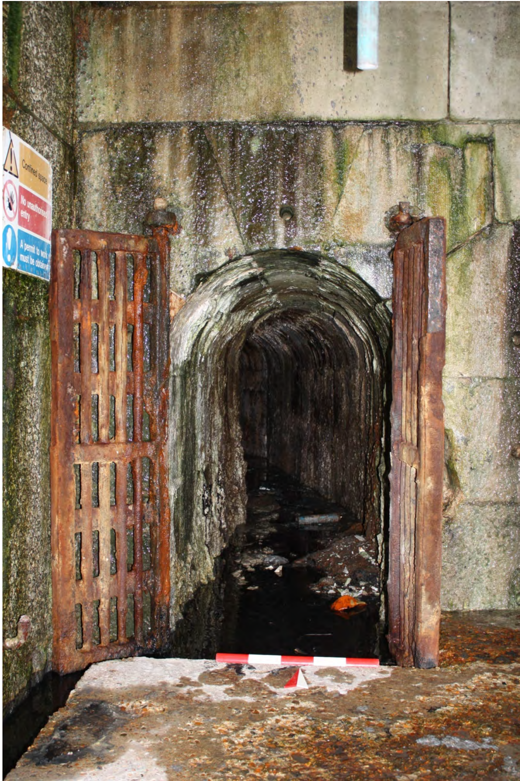
Plate 11. D305/74. Entrance to culvert [108] in the base of the NW corner of Dry Dock No. 3. Cast iron gates open. The standing water is c. 0.20m deep. Scale is 0.5m looking N.
