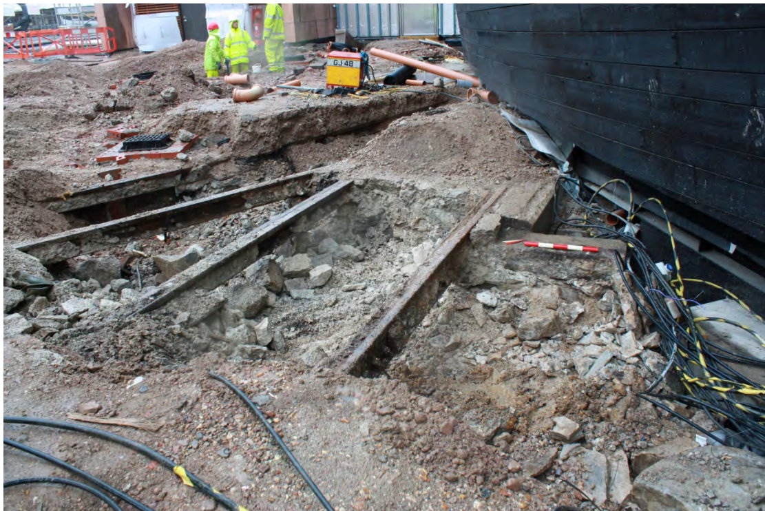
Plate 14. D320/26. 1920s crane rails at SE end of Dry Dock No. 3. Scale is 0.50m looking W.
