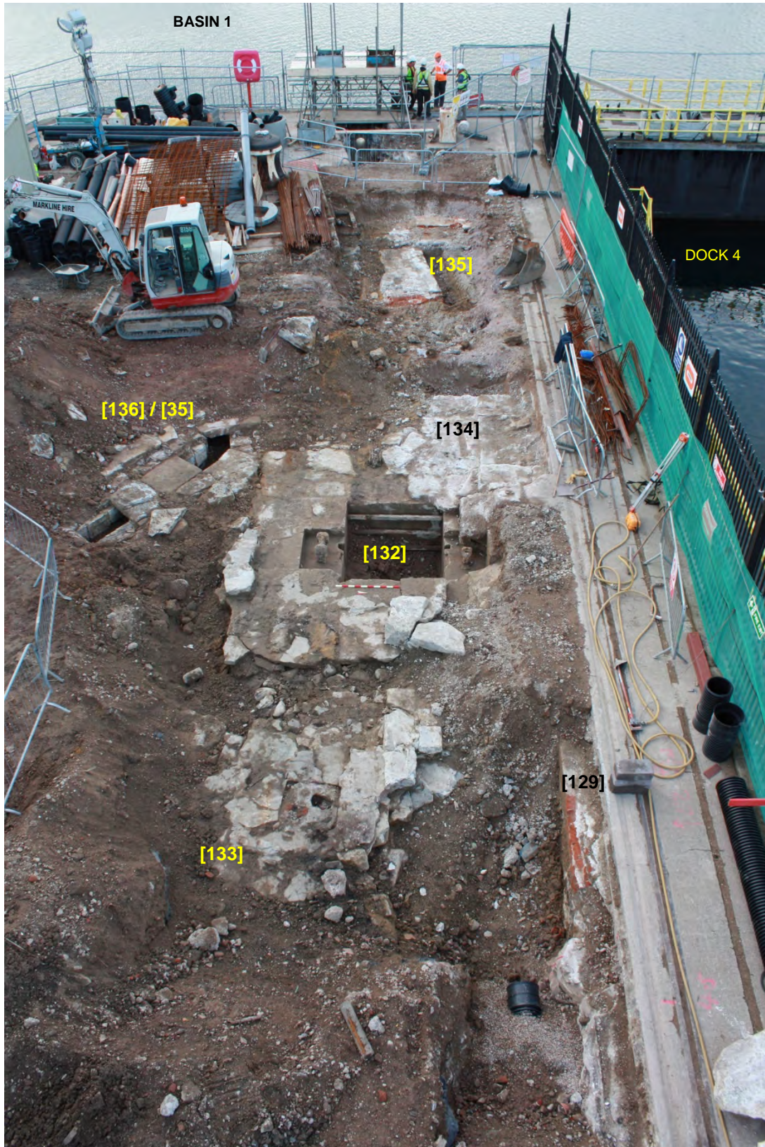
Plate 8. D312/40. Aerial view looking down on north side of Dry Dock No. 3, NW end, showing the principal features unearthed in this area. Scale is 1.0m looking west
