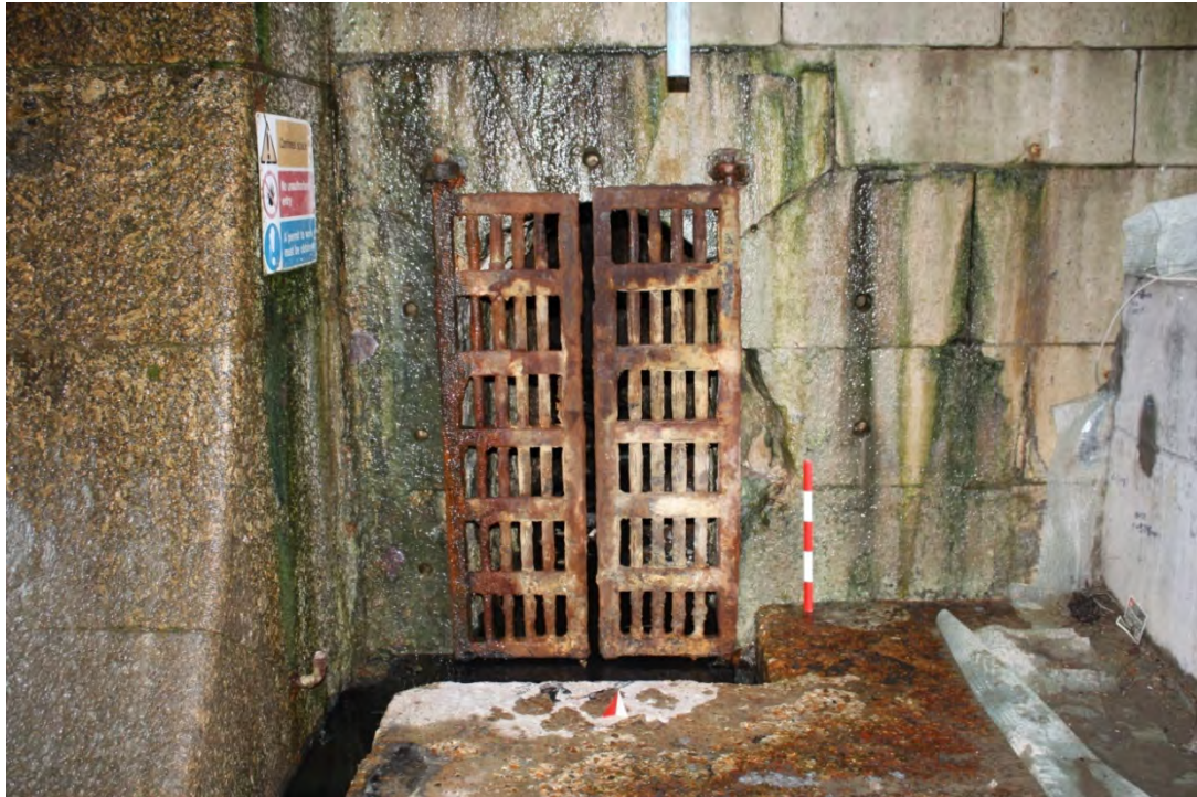
Plate 9. D305/72. Entrance to culvert [108] in the base of the NW corner of Dry Dock No. 3. Cast iron gates closed. Scale is 0.5m looking N.
