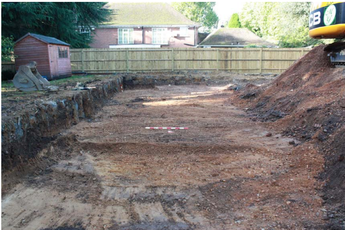
Plate 2: D1.7 taken 16/10/12. TR1. View of slighter deeper excavated eastern end of trench showing darker gravelly sand [2] overlaying the lighter sandy gravel [3]. Scales 1m and 0.5m looking W.
