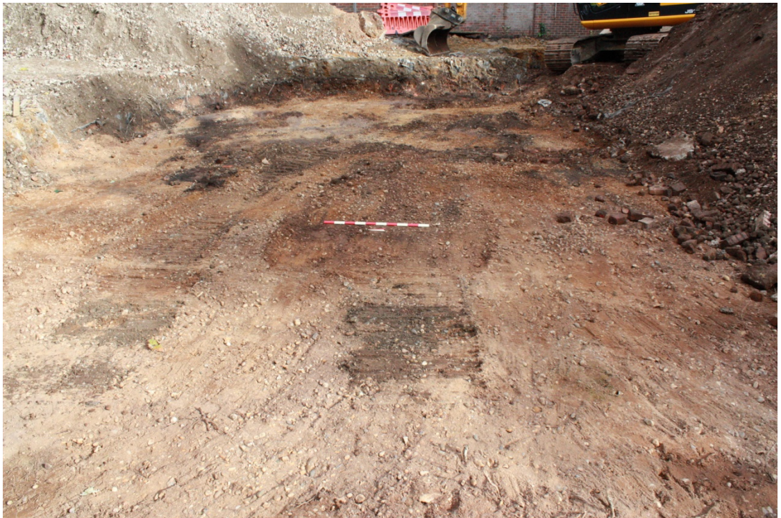
Plate 4: D1.14 taken 16/10/12. TR1. The north-east corner of the site. The dark stains are the footings of a recently demolished out-building that cuts the natural [2]. Scale 1m looking E.
