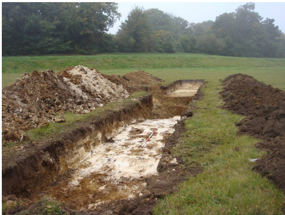
PLATE 6: Trench 3, view south-west with glacial channel in middle of trench. The terracing (cutting-away of the original ground level) on the south-west side of the site can be seen in the background.
