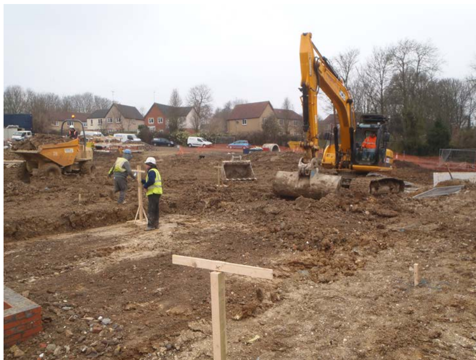
PLATE 15: Ground reduction in road corridor (central western part of site), carried out under watching brief conditions
