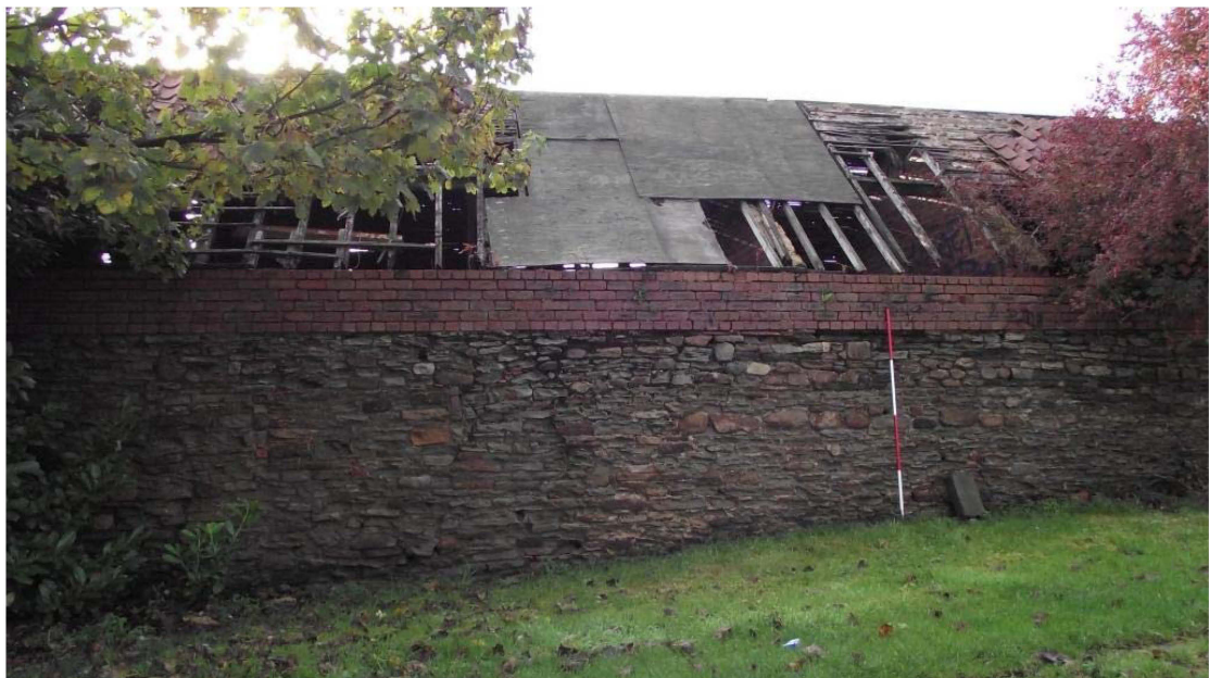
Photograph 10: North range, north-east facing elevation, south end, front on view (2m scale)
