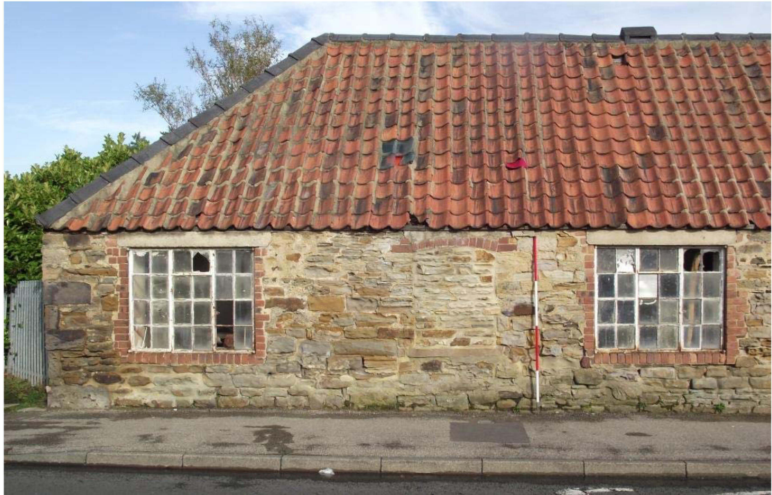
Photograph 5: South range, south-west facing elevation, north end, front on view (2m scale)
