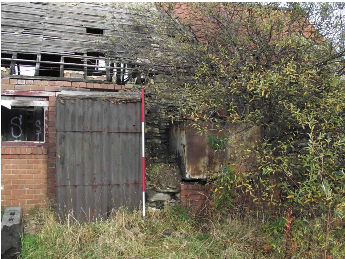
Photograph 16: North range, south-east facing elevation, south end, front on view (2m scale)
