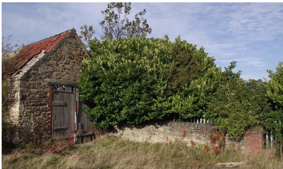
Photograph 20: North range, southern gable end and boundary wall, looking NNE (2m scale)
