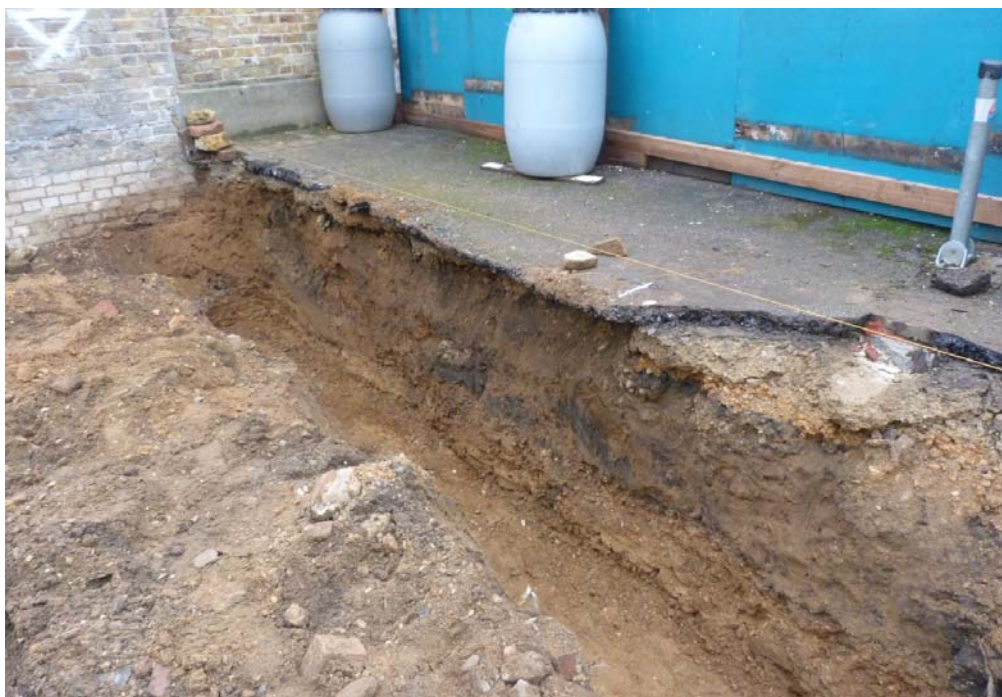
Plate 1: Representative site section, view north, at north-westernmost corner of the site, boundary with 51 Setchell Road
