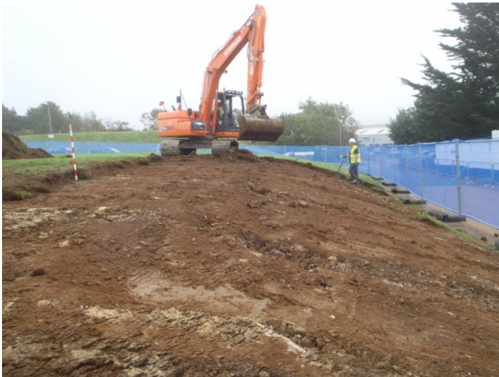
Plate 3: The stripped surface at the required maximum 200mm depth, view to west (1m scale)
