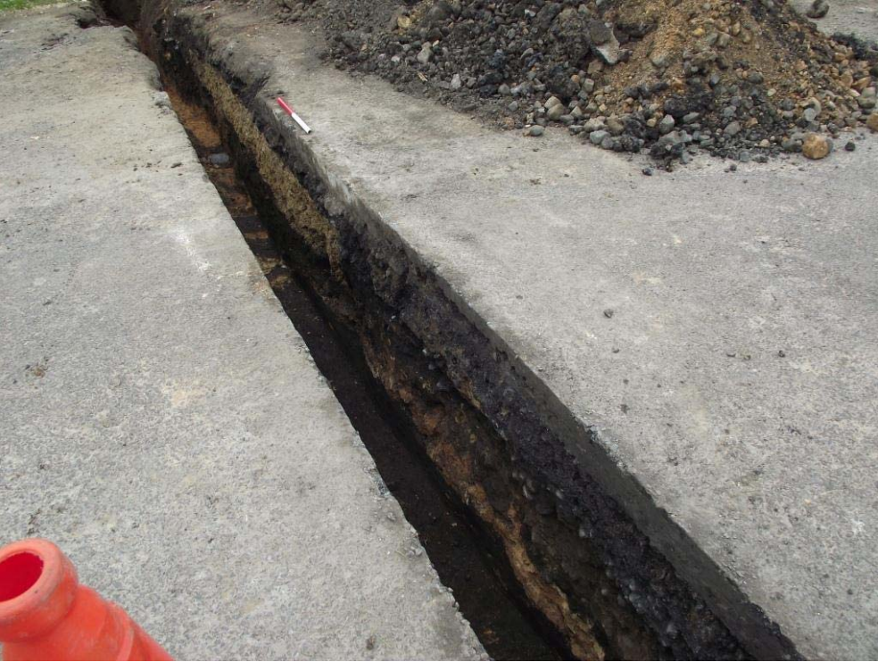
Figure 5: Overview of the cable trench across Brusselton Lane, looking WSW (scale 0.5m)
