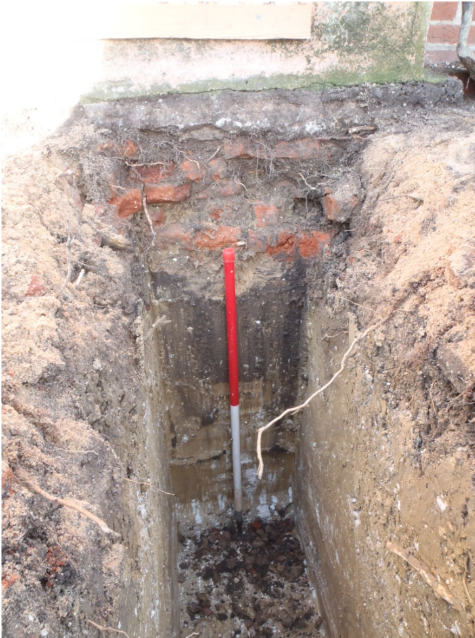
Plate 7: North-eastern strip foundation, view north-west showing brick foundation wall [5] for sill beam of existing timber-framed house (1m scale)
