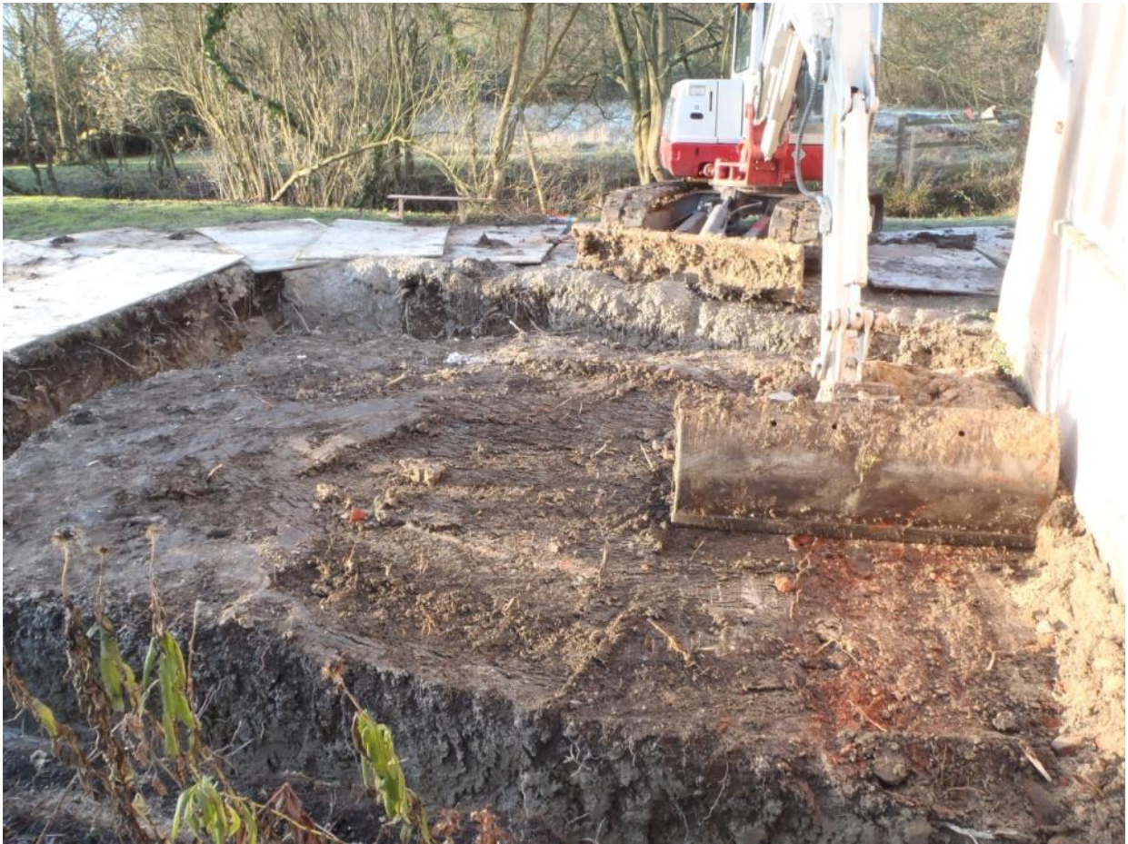
Plate 5: Removal of Made Ground (2) and (immediately adjacent to gable wall of house) Levelling Layer (6) under archaeological supervision
