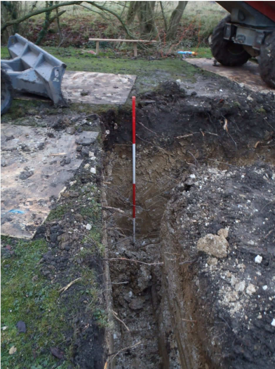
Plate 6: South-eastern strip foundation (end wall of garden room), view west showing (from top to base of section): Garden Soil (1), Made Ground (2) and Natural Clay (3) (2m scale)
