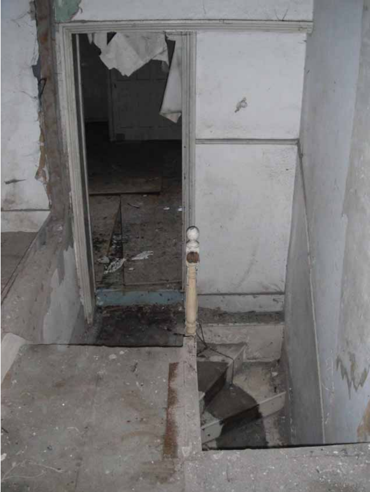
Plate 15: Stairs from the first floor to the ground floor in 204, Grange Road, looking north (PCA Archive no. GBR12 DSCF0785)
