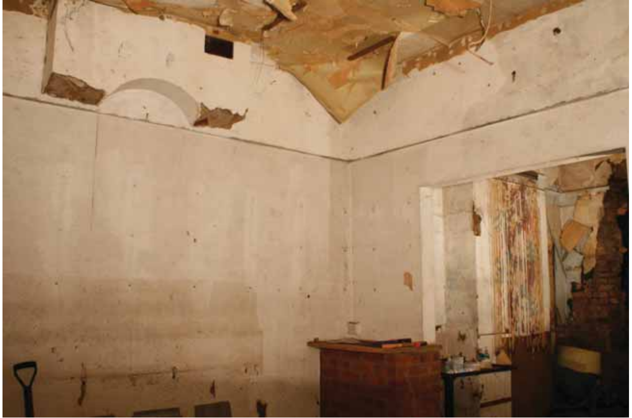
Plate 7: West wall of shop of 204, Grange Road, looking north-east (PCA Archive no. GBR12 D100 (15a))
