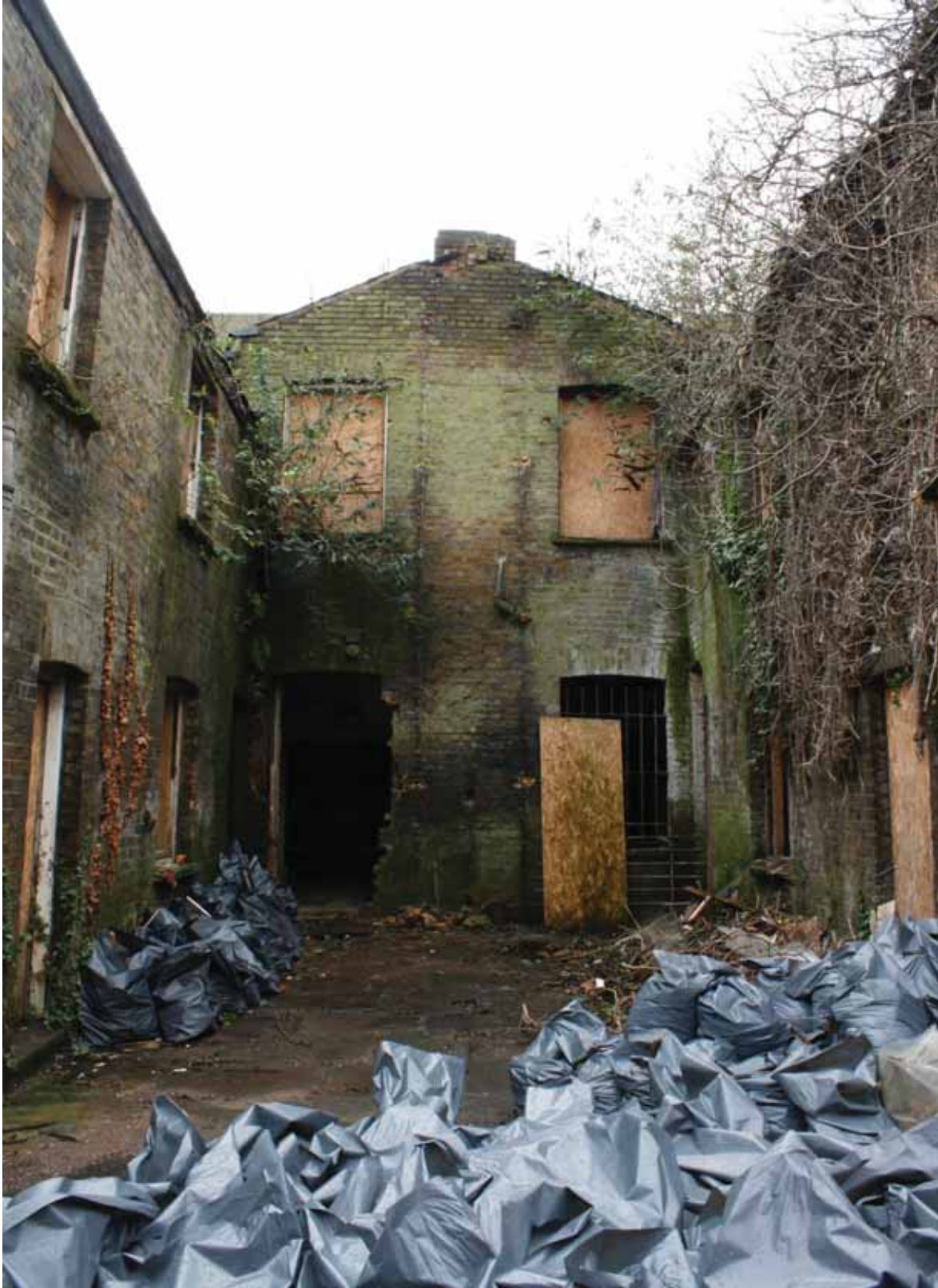
Plate 4: Rear (north) elevation of 204 (left) to 205 (right), Grange Road, looking south (PCA Archive no. GBR12 D100 (8))
