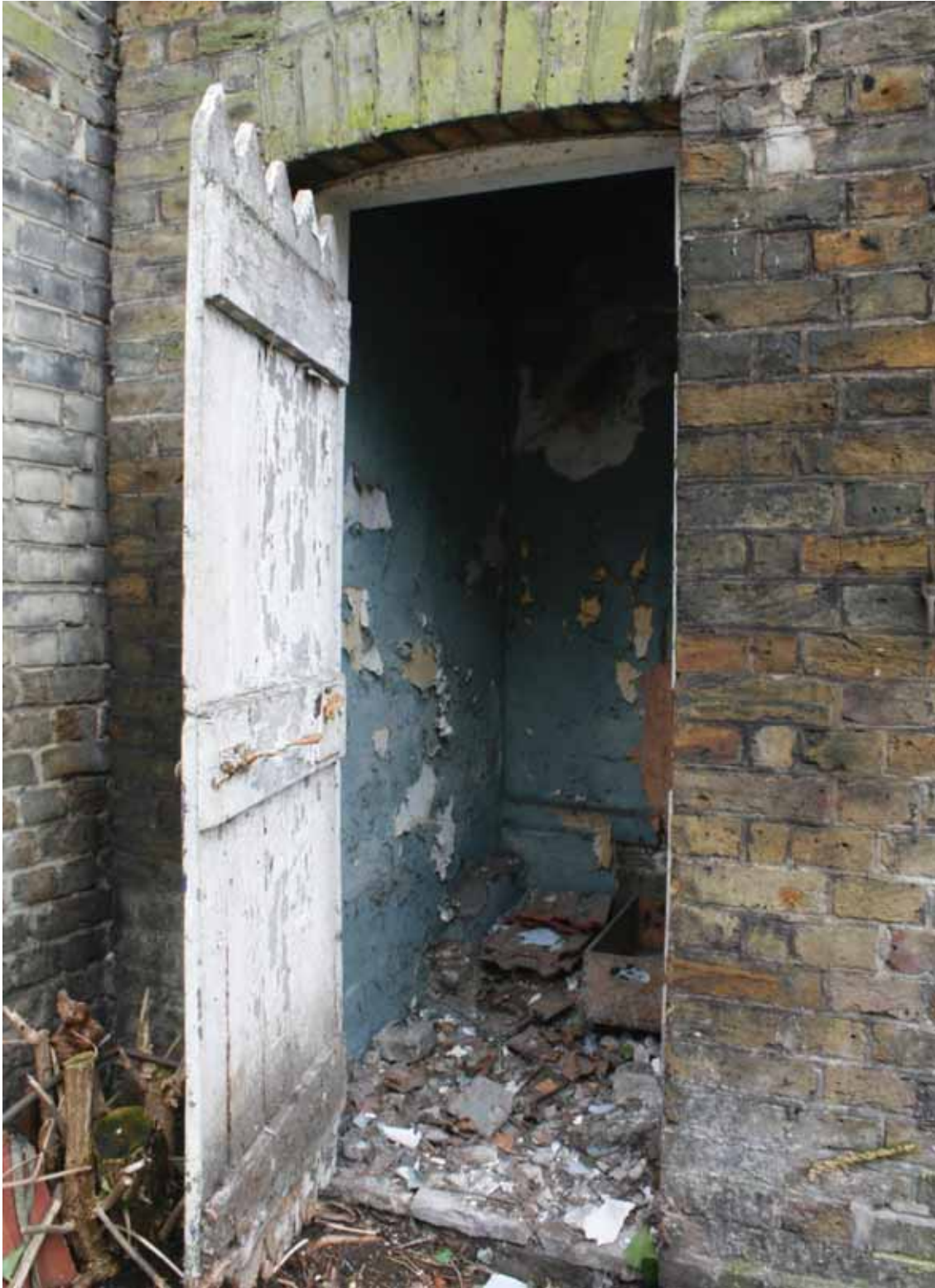
Plate 13: Toilet at the north end of 204, Grange Road, looking south (PCA Archive no. GBR12 D100 (11))
