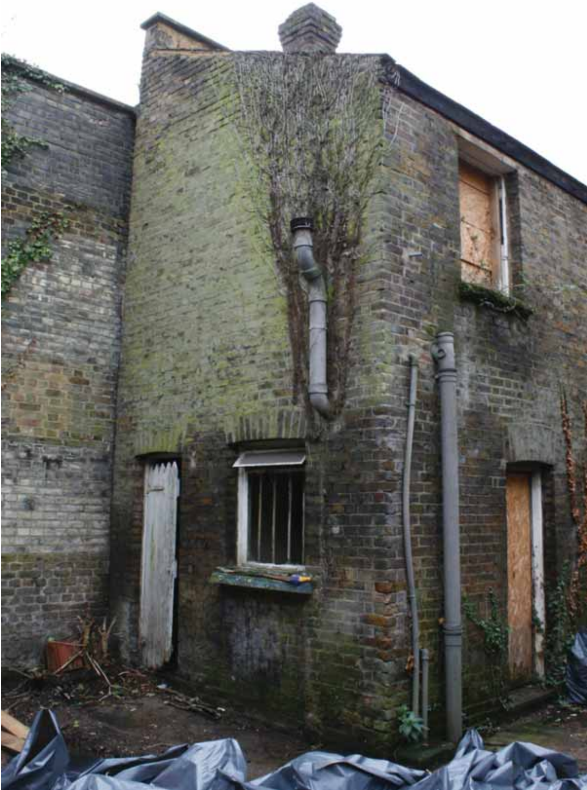
Plate 6: Rear (north) extension of 204, Grange Road, looking south-east (PCA Archive no. GBR12 D100 (6))
