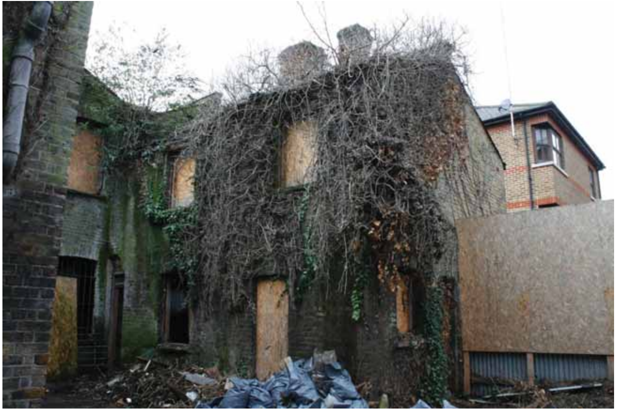
Plate 5: Rear (north) extension of 205, Grange Road, looking south-west (PCA Archive no. GBR12 D100 (9))
