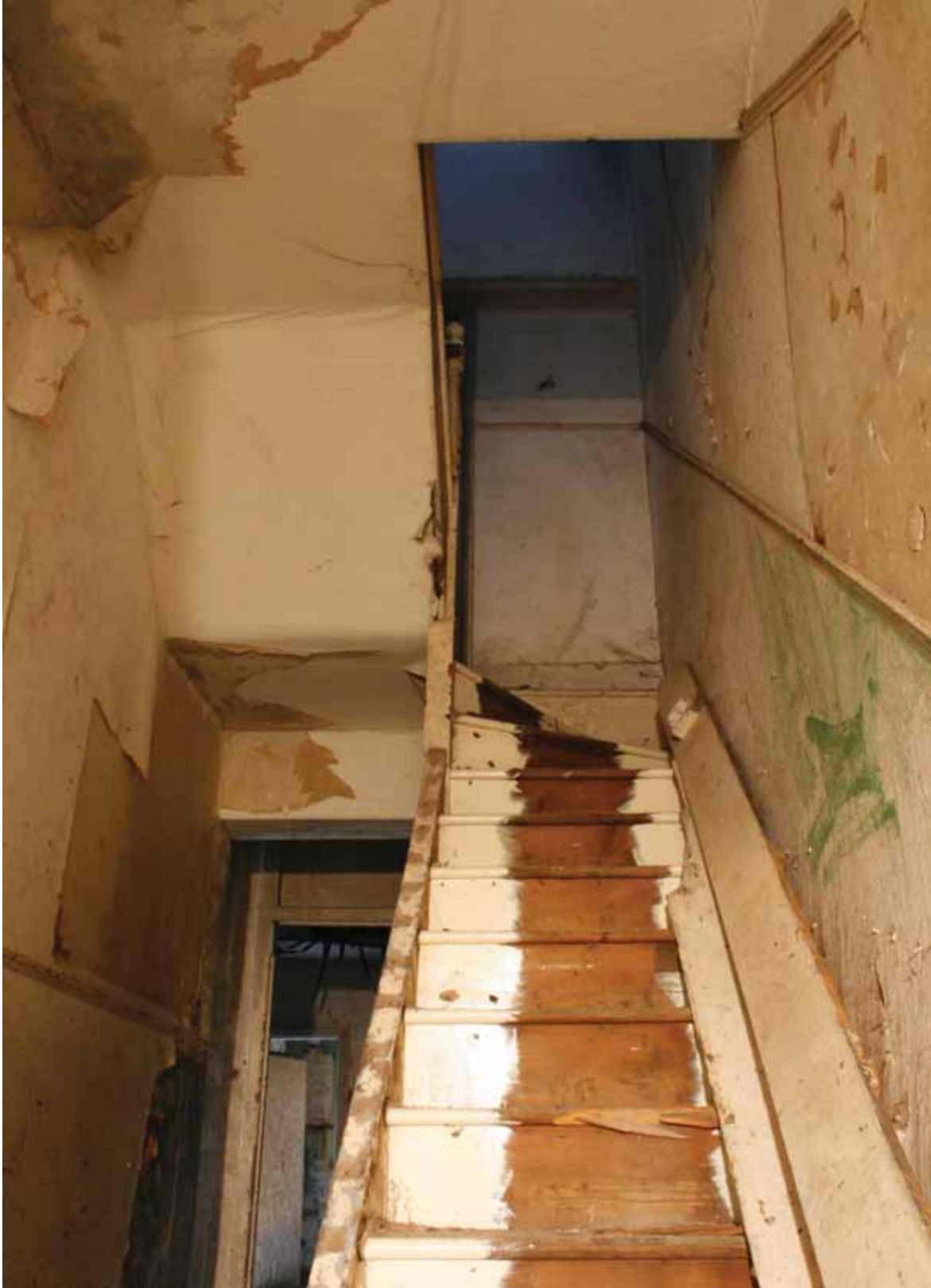
Plate 14: Stairs up to the first floor in 204, Grange Road, looking north (PCA Archive no. GBR12 D100 (21a))
