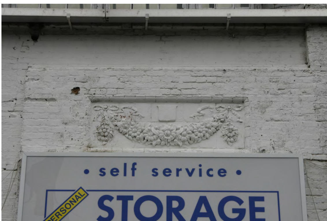
Plate 4: Terracotta embossed plaque with fruit design on south-west facade, looking north-east (72FmLa D100 030)
