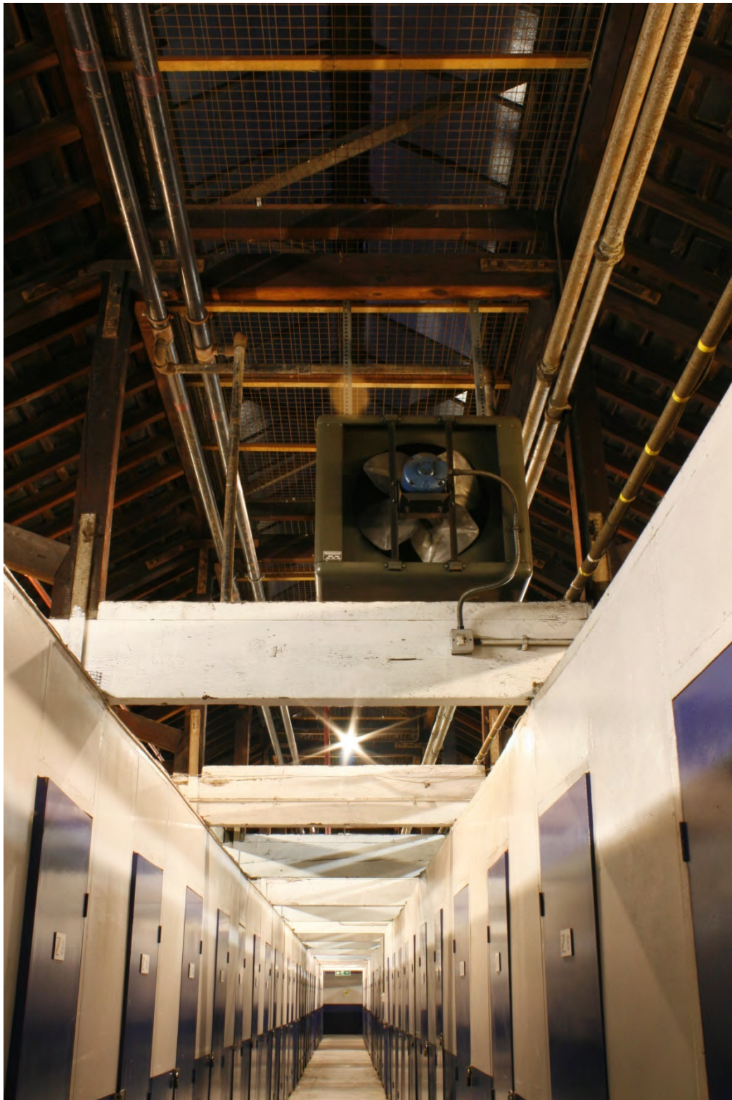
Plate 43: First floor access corridor along storage area on the north side of the building, showing original Queen truss, looking north-east (72FmLa D100 059)
