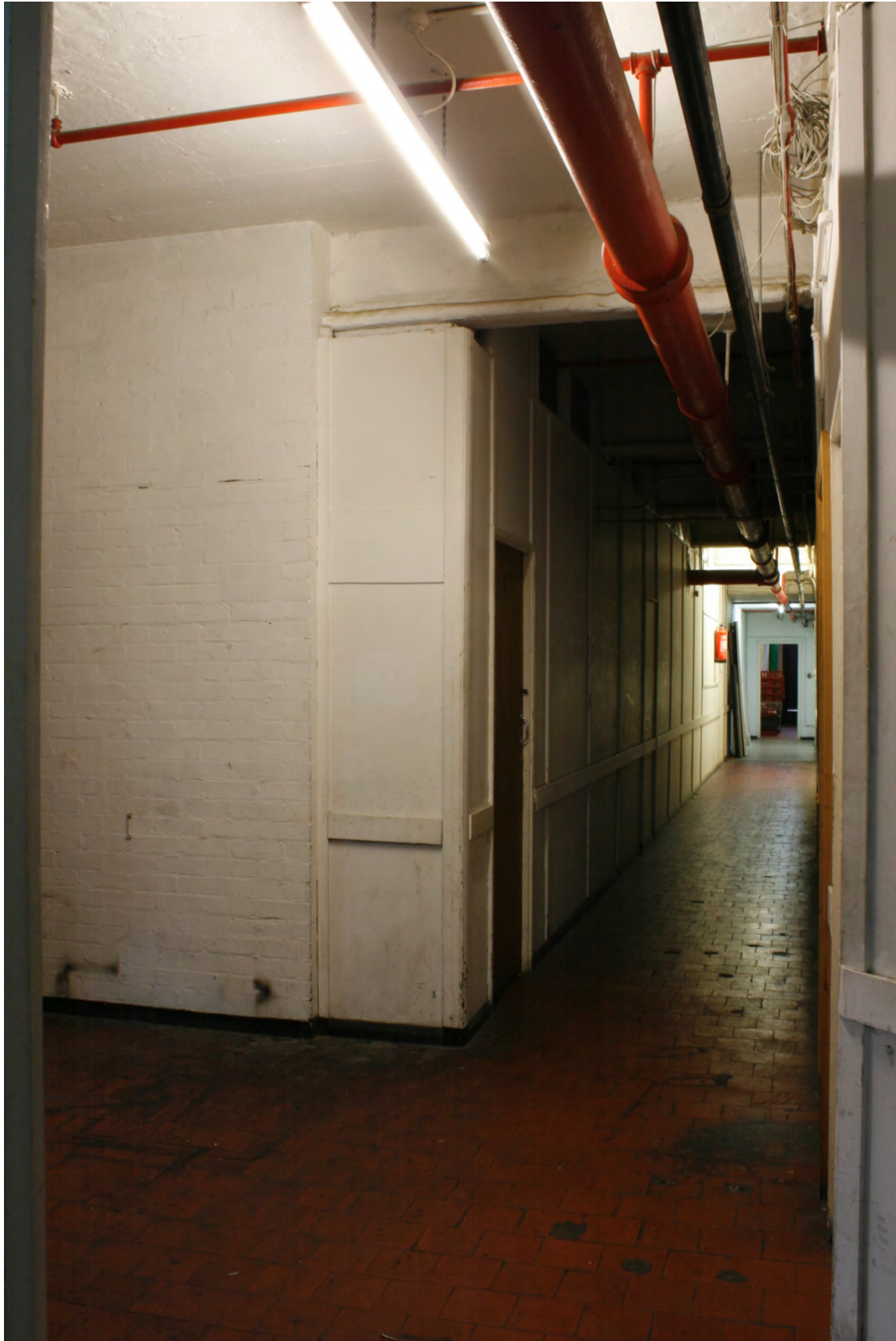
Plate 37: Ground floor access corridor within storage area on the north side of the building, looking south-west (72FmLa D100 044)
