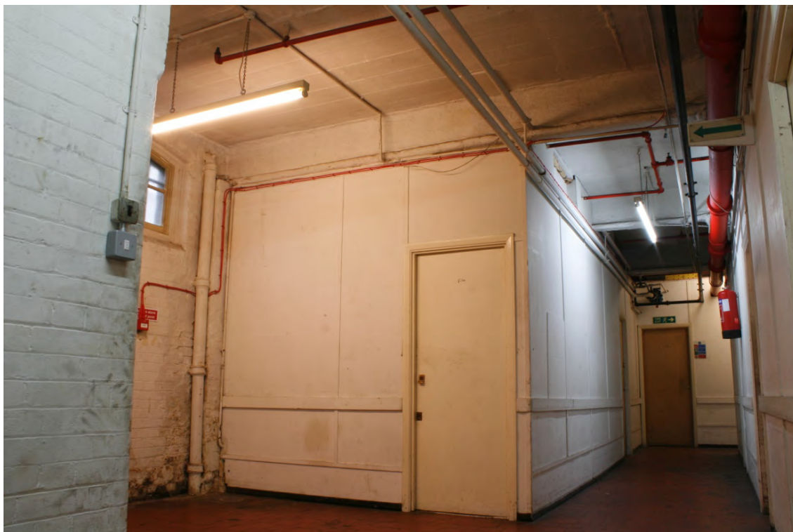
Plate 40: Ground floor access corridor within the storage area on the north side of building showing added late 20 th century plywood partition walls and two doorways, looking east (72FmLa D100 046)
