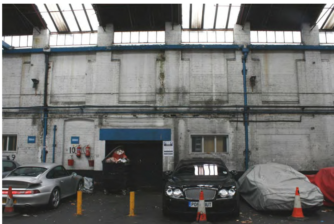
Plate 30: Inserted ground floor windows, original doorway (since infilled with brickwork), inserted double doorways (one blocked) on the north side of the building, looking north-west (72FmLa D100 034)
