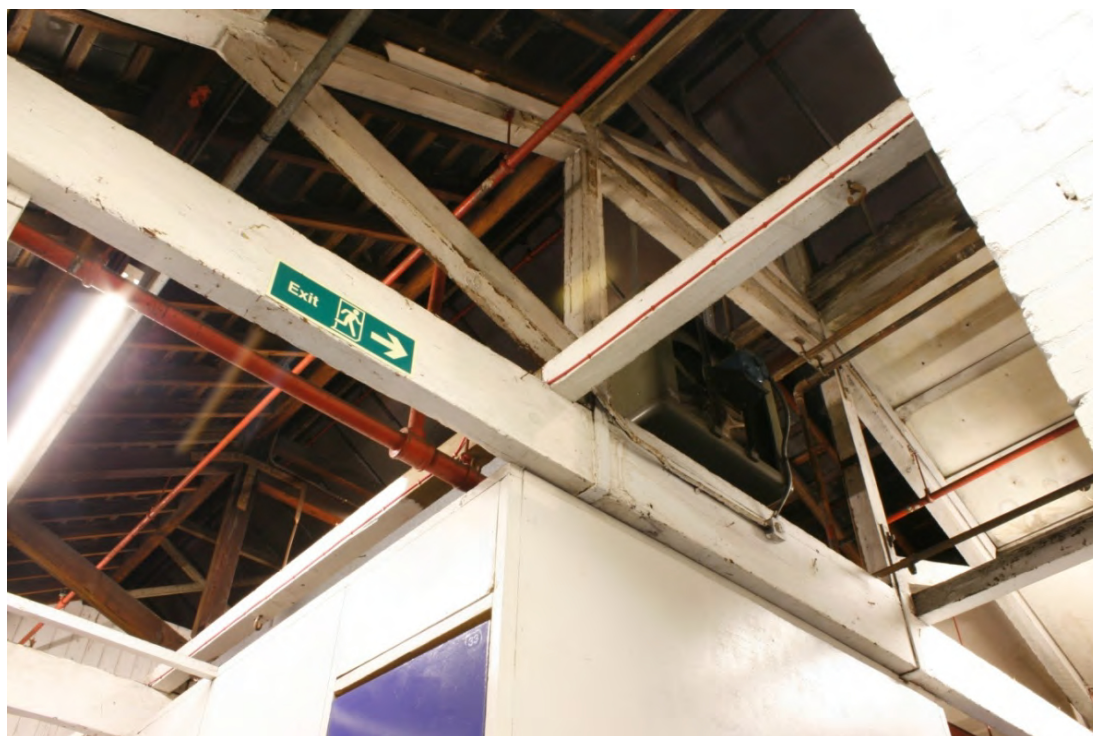
Plate 44: Original Queen truss above the first floor storage area on the north side of the building, looking east (72FmLa D100 060)
