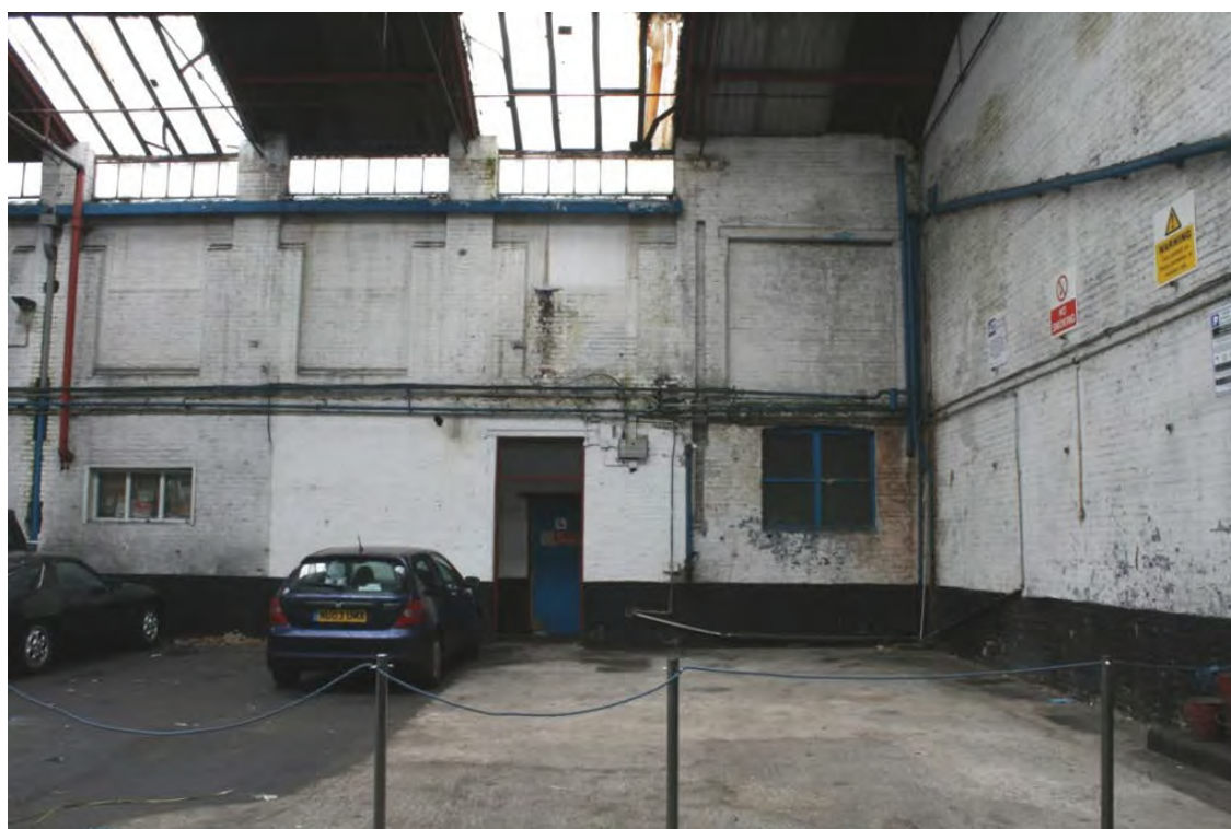
Plate 28: Original window opening (right) and later inserted door (centre) and ground floor window (left) on the north side of building, looking north (72FmLa D100 032)
