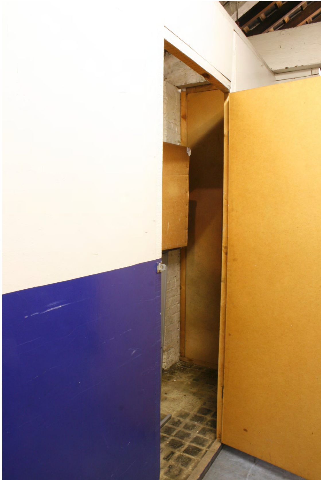
Plate 46: Original cobbling within a small storage space area on the first floor, looking north (72FmLa D100 062a)
