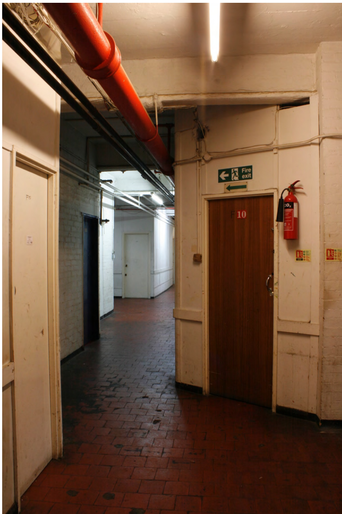
Plate 39: Ground floor access corridor within the storage area on the north side of building showing added late 20 th century plywood partition walls and doorway, looking north-east (72FmLa D100 045)
