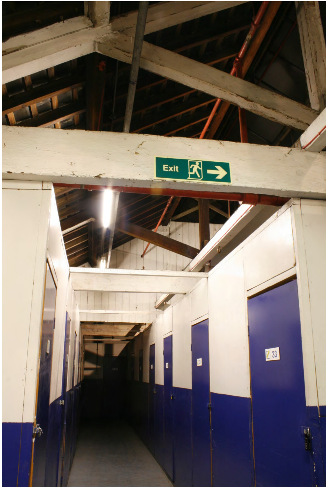
Plate 45: First floor access corridor along the storage area on the north side of building with original timber roof trusses overhead, looking north-east (72FmLa D100 041)
