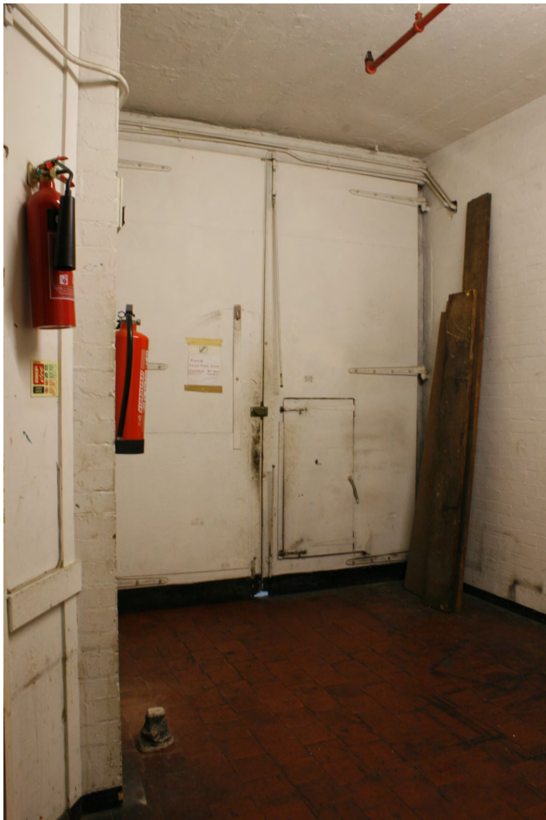
Plate 36: Double door with cast iron strap hinges stamped Charles Collinge of Lambeth, looking south (72FmLa D100 043)
