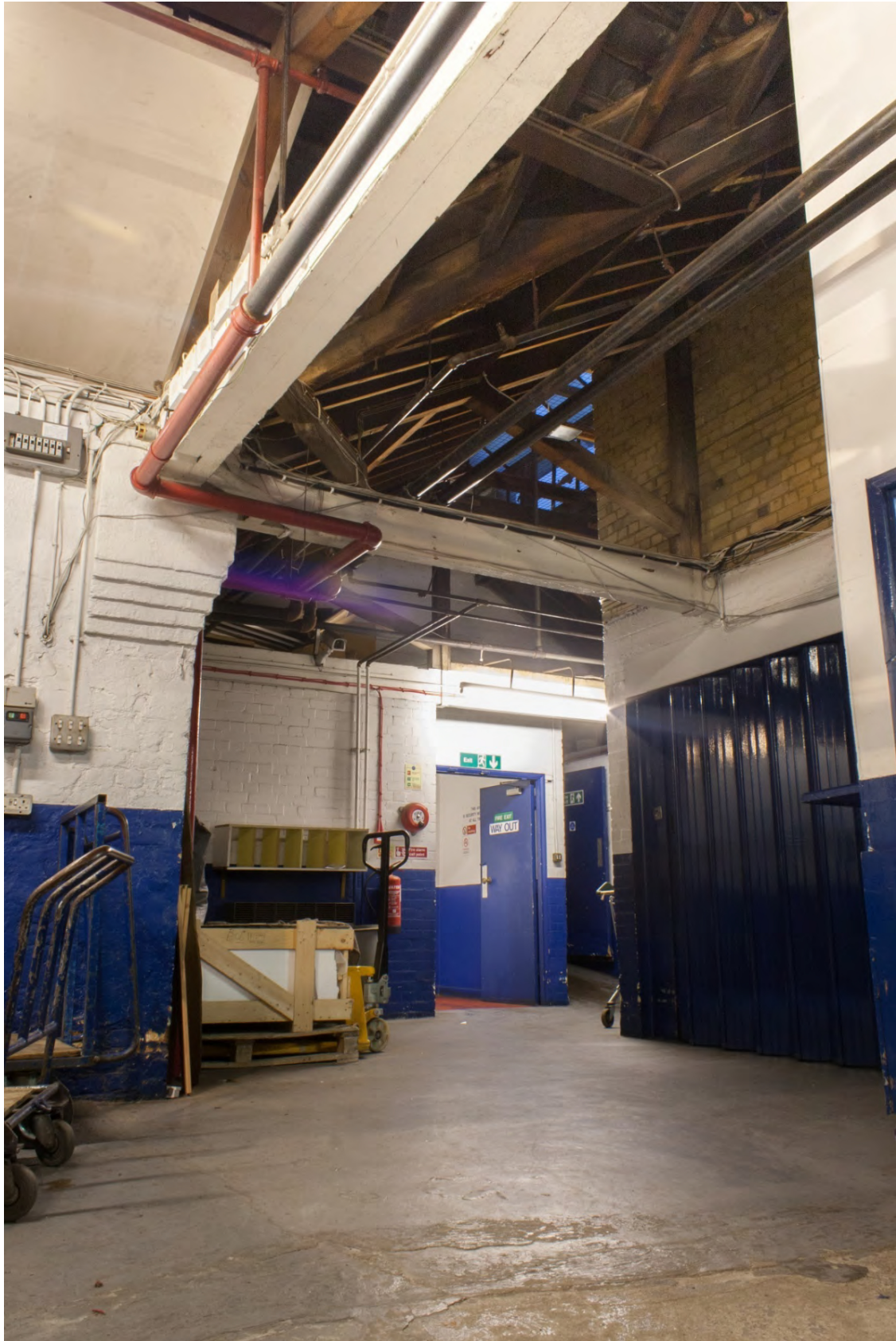
Plate 42: Entrance into the first floor storage area on the north side of the building, showing roof structure and 20 th century brick partition walls, looking south (72FmLa D100 058)
