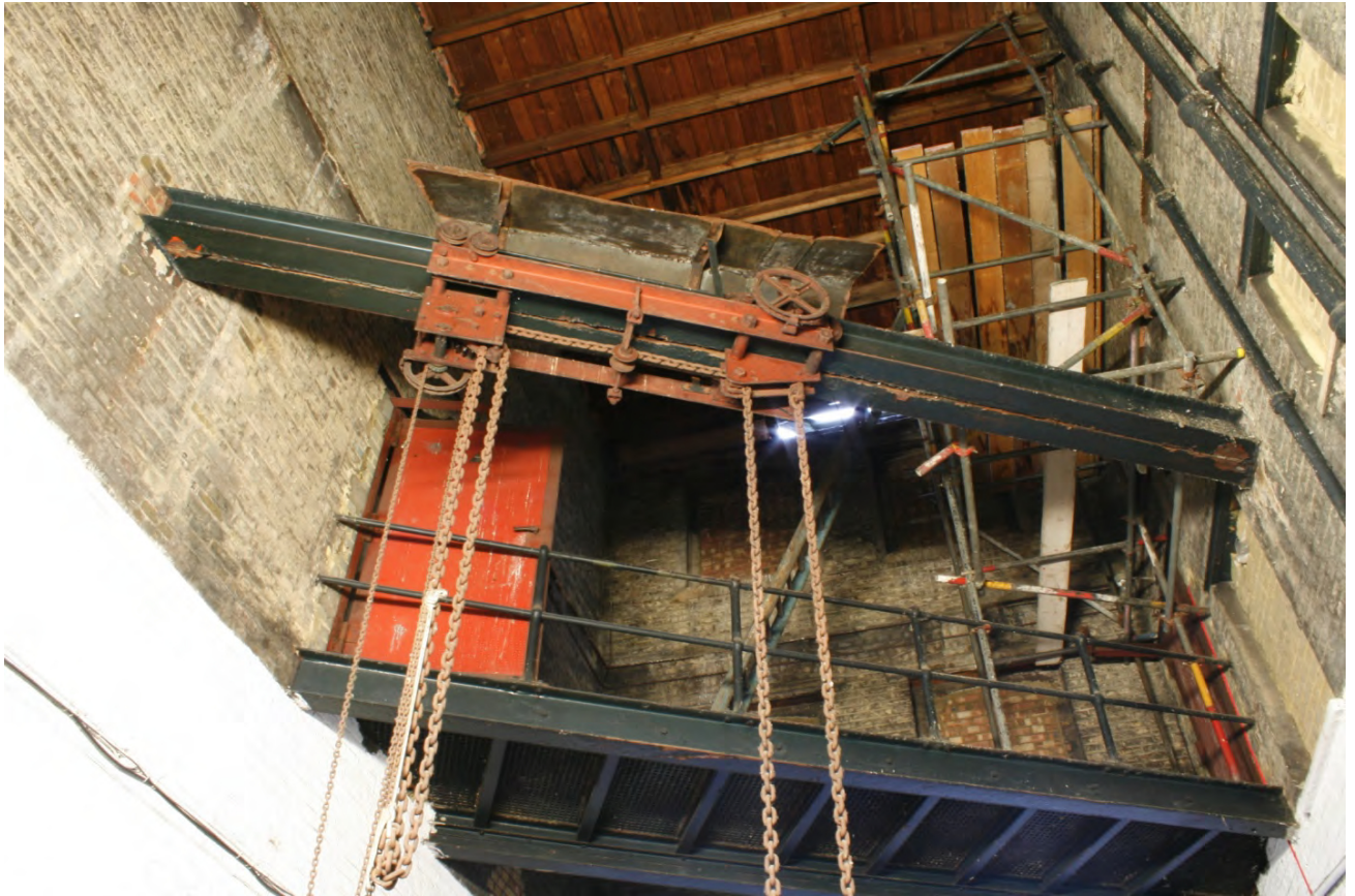
Plate 23: Overhead bridge and winching mechanisms within passageway from the main workshop area of the garage to the parking area beyond, looking south-west (72FmLa D100 053)
