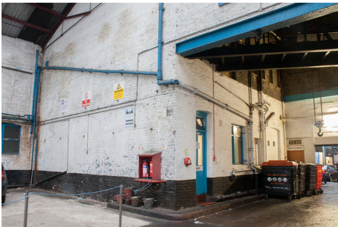
Plate 25: Passageway entrance leading from the parking area at the south-west end of the building to the main workshop area beyond, looking north (72FmLa D100 055)
