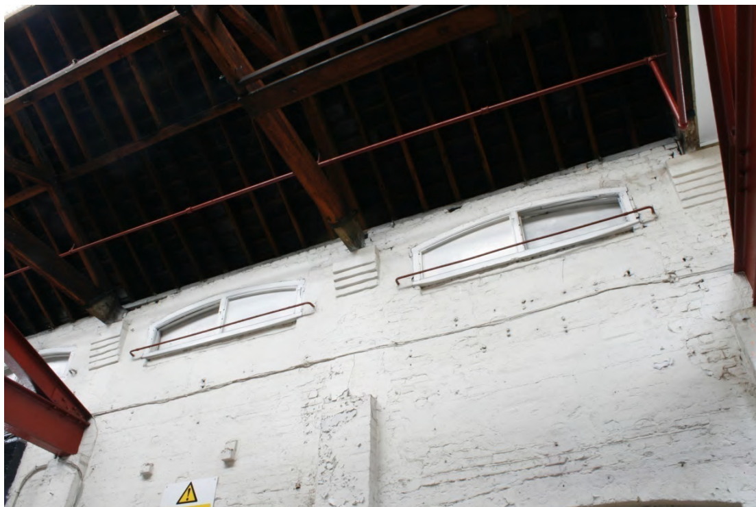
Plate 13: Internal view of blocked transom windows in the north-east elevation, looking north-east (72FmLa D100 017)
