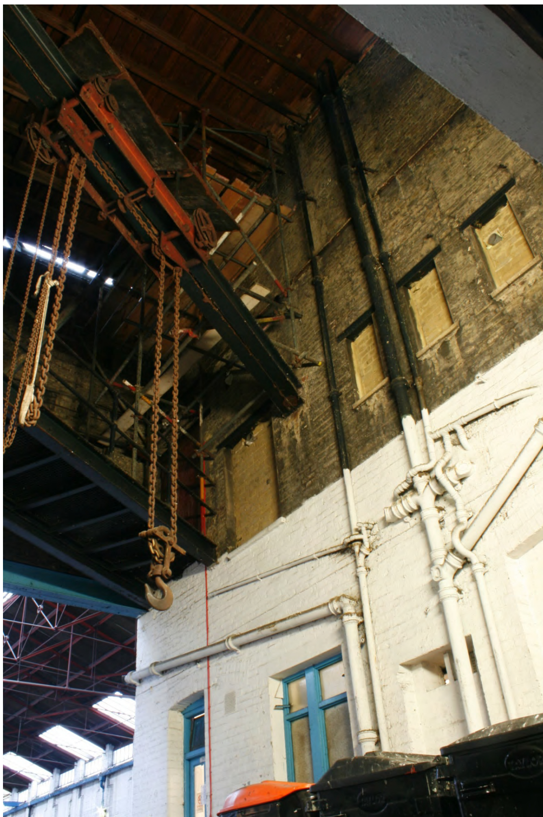
Plate 22: Passageway from the main workshop area of the garage to the parking area beyond showing blocked windows, overhead bridge and winching mechanisms, looking west (72FmLa D100 052)
