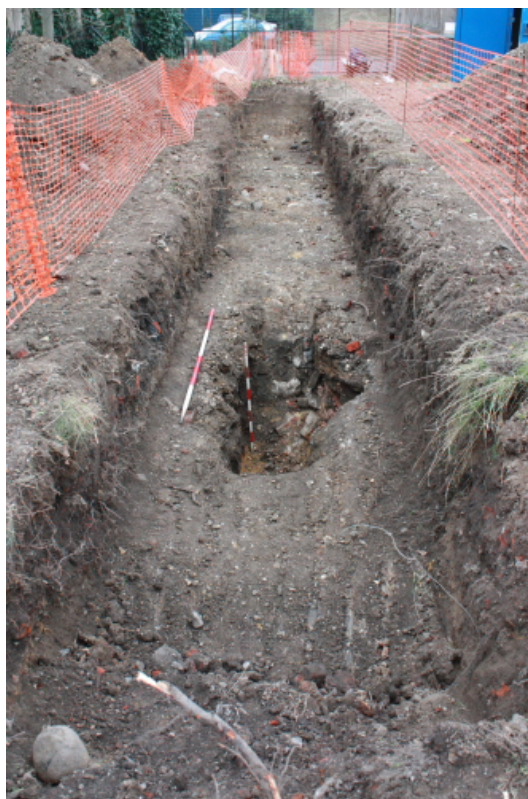
Plate 5: North-West facing view of Trench 6 showing significant modern truncation across the area
