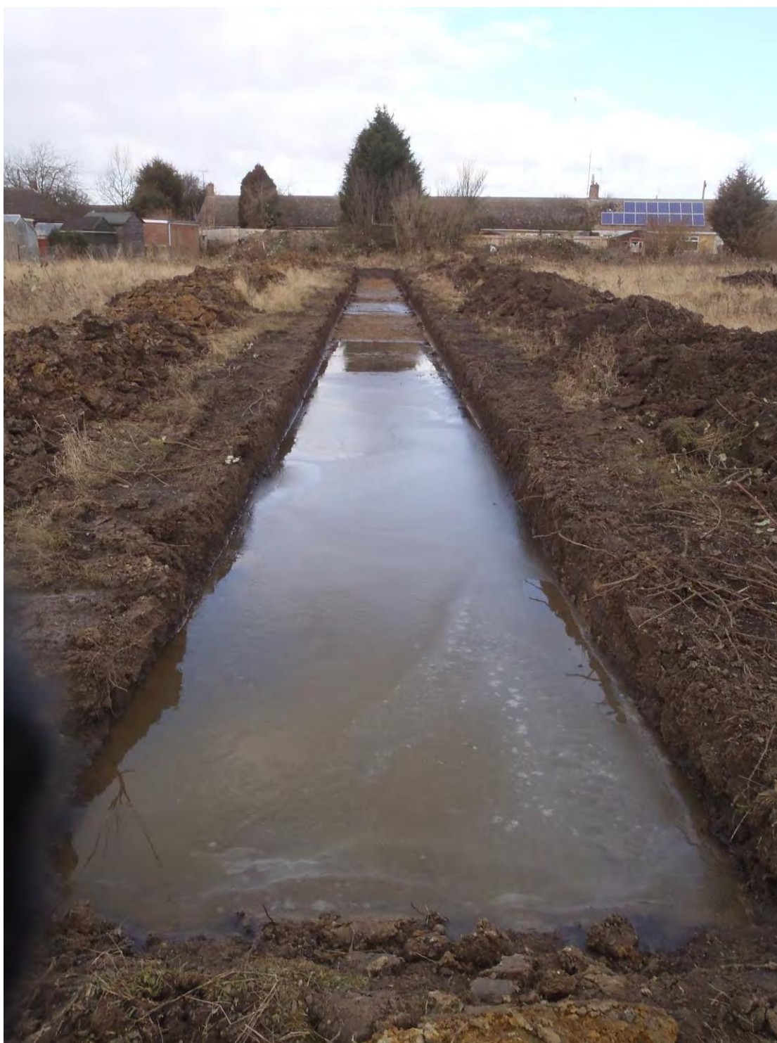
Plate 8: Trench [2], view north-west showing full extent of flooding
